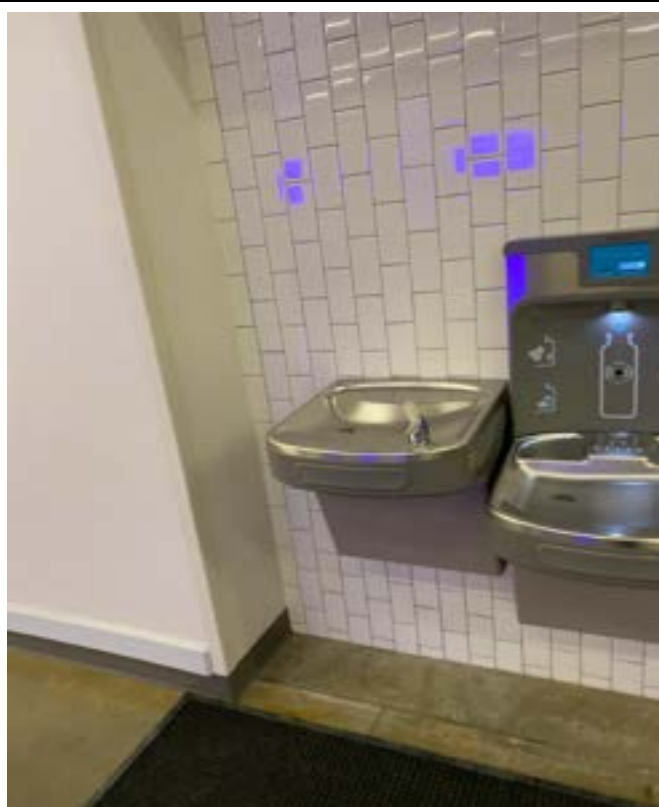
1/16/2024 - 3901-34 - Northview Elementary - Cafeteria-Left
