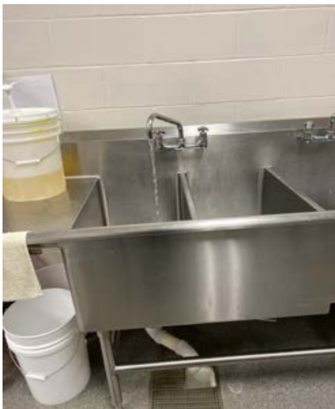
1/16/2024 - 3901-31 - Northview Elementary - Kitchen-Three Bay Sink-Left
