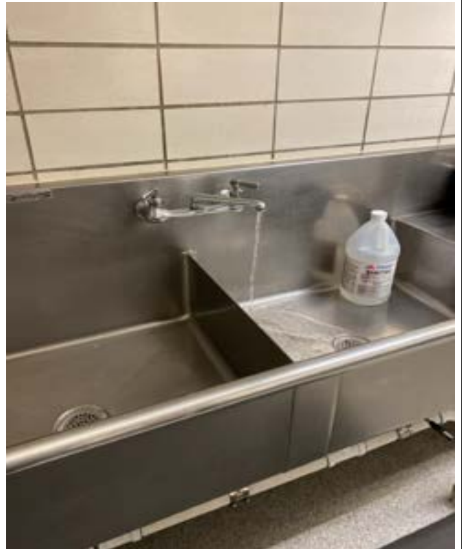
1/17/2024 - 5300-14 - Maple Park Middle School - Kitchen-3 Bay Sink-Right
