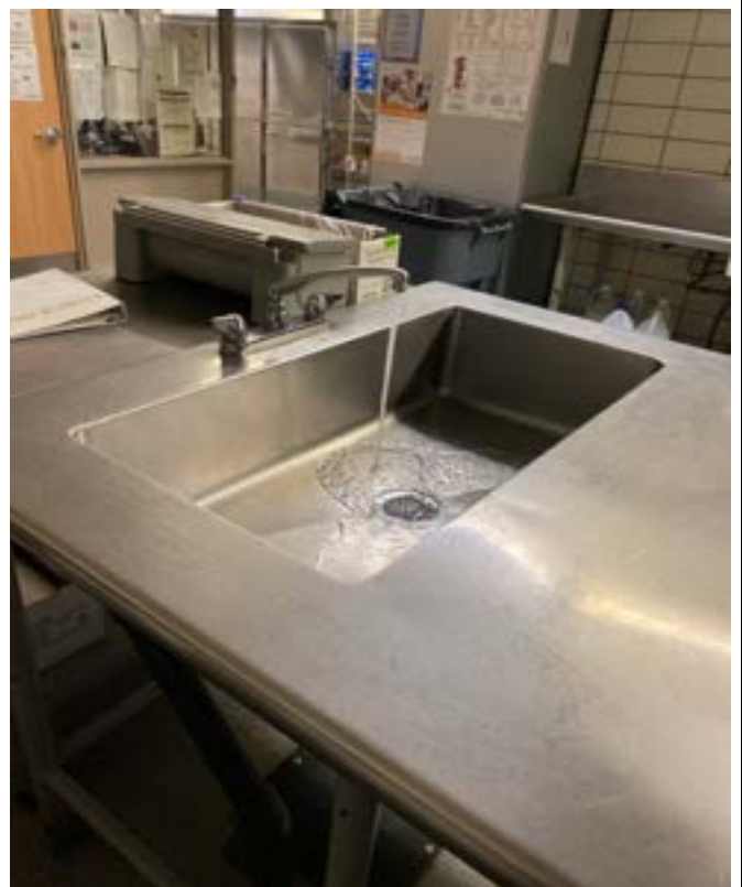
1/17/2024 - 5300-12 - Maple Park Middle School - Kitchen-West Middle Sink
