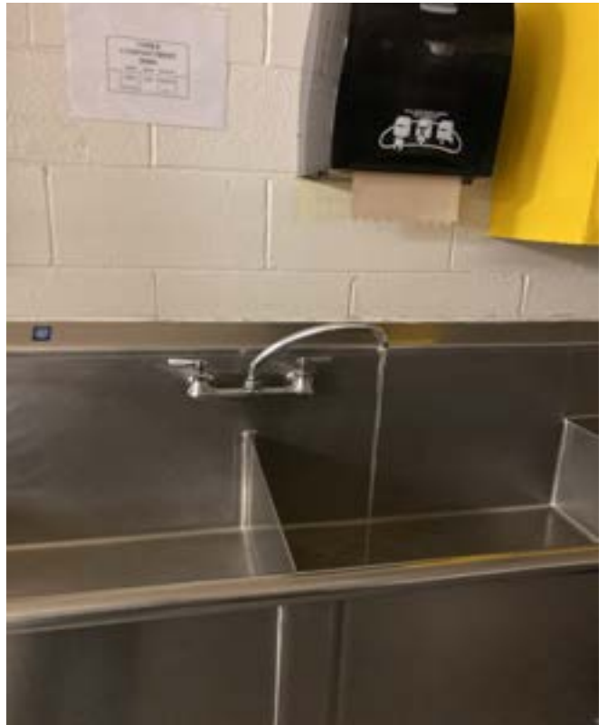
1/11/2024 - 7333-22 - Linden West Elementary - Kitchen-Three Bay Sink-Right
