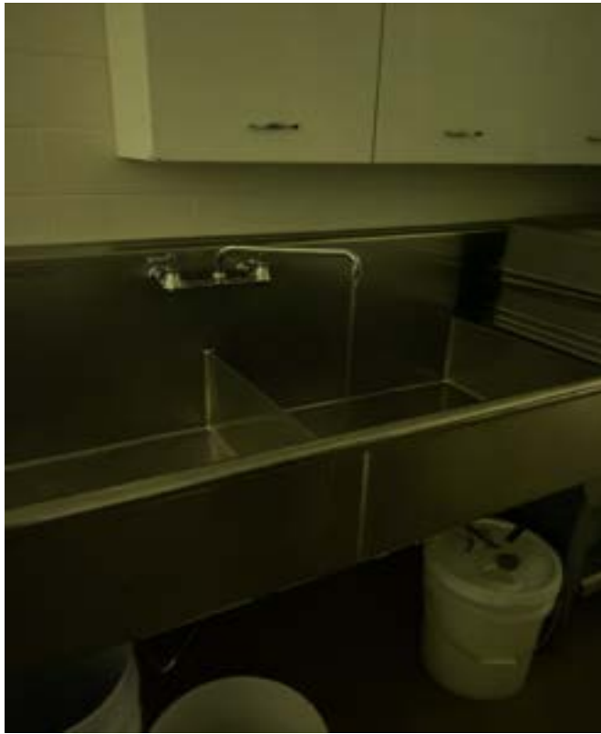
1/5/2024 - 5125-65 - Gracemor Elementary - Kitchen-3 Bay Sink-Right
