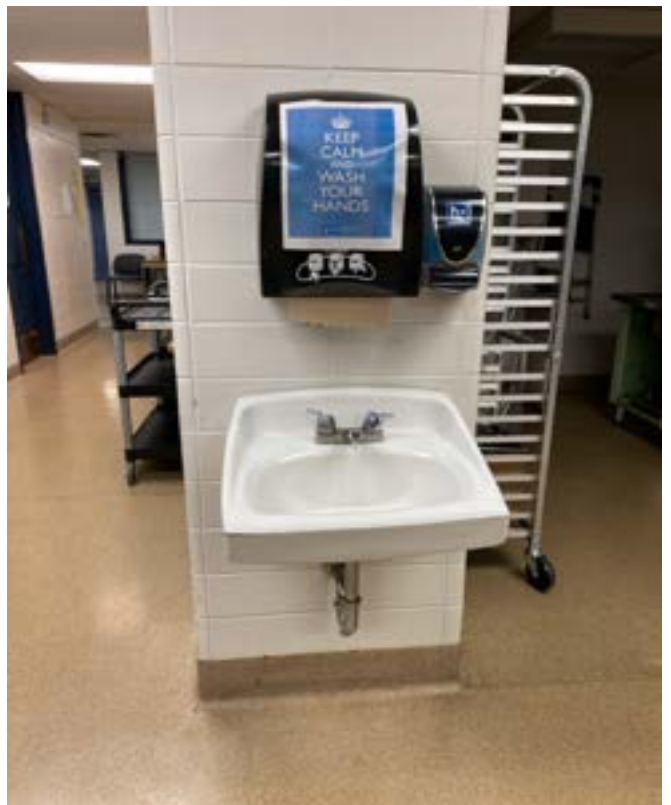
1/5/2024 - 5125-68 - Gracemor Elementary - Kitchen-South Handwashing Sink
