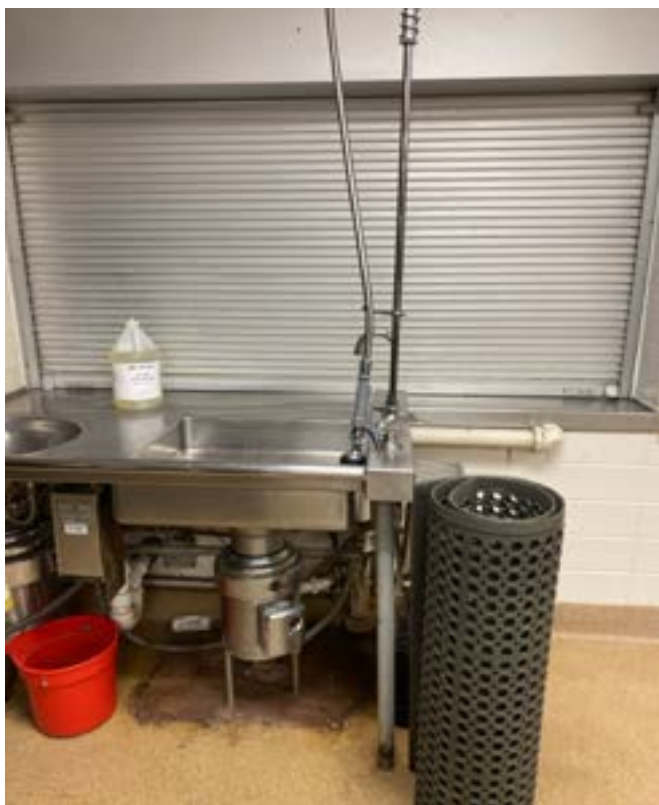
1/5/2024 - 5125-63 - Gracemor Elementary - Kitchen-North Sink
