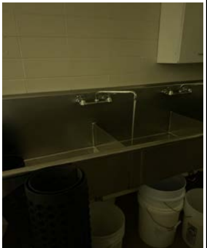
1/5/2024 - 5125-64 - Gracemor Elementary - Kitchen-3 Bay Sink-Left
