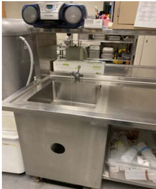
1/16/2024 - 9201-53 - Gateway Middle School - Kitchen-North Middle Sink
