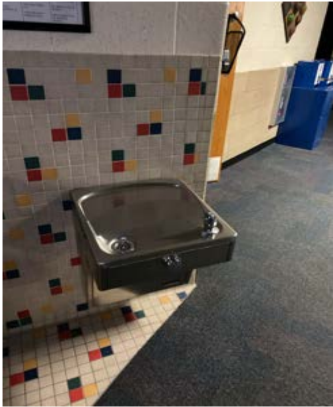
1/16/2024 - 9201-29 - Gateway Middle School - Outside 400 Pod-Right
