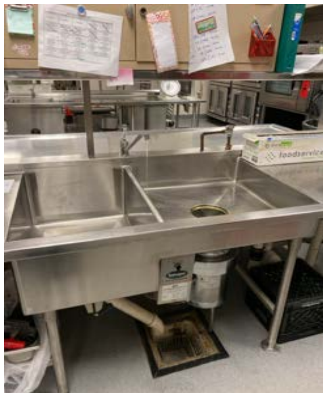
1/16/2024 - 9201-51 - Gateway Middle School - Kitchen-South Middle Sink
