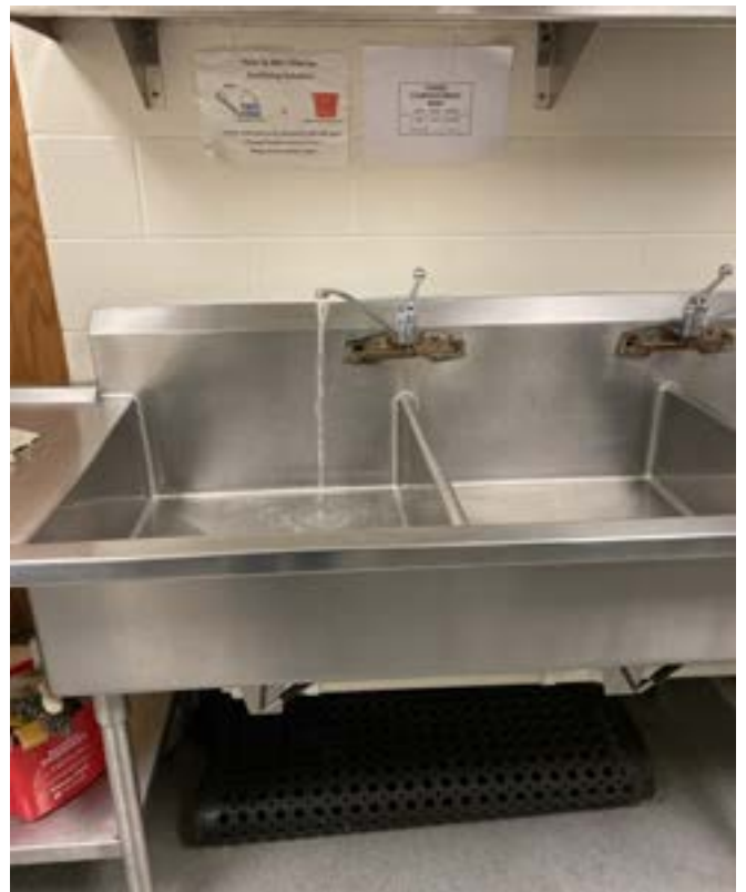
1/16/2024 - 9201-54 - Gateway Middle School - Kitchen-Four Bay Sink-Left
