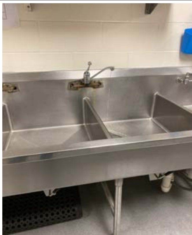
1/16/2024 - 9201-55 - Gateway Middle School - Kitchen-Four Bay Sink-Middle
