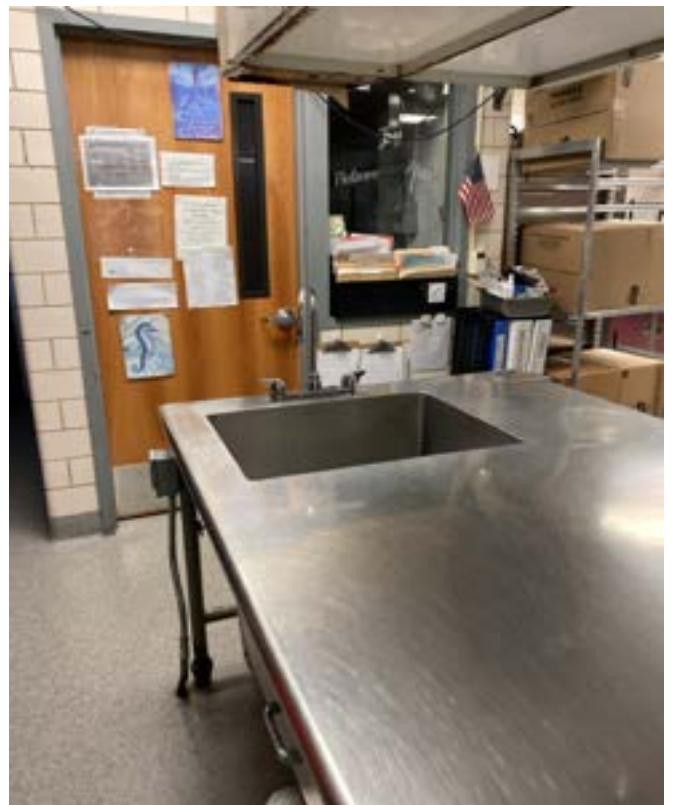
1/23/2024 - 2100-24 - Antioch Middle School - Kitchen-Middle Sink
