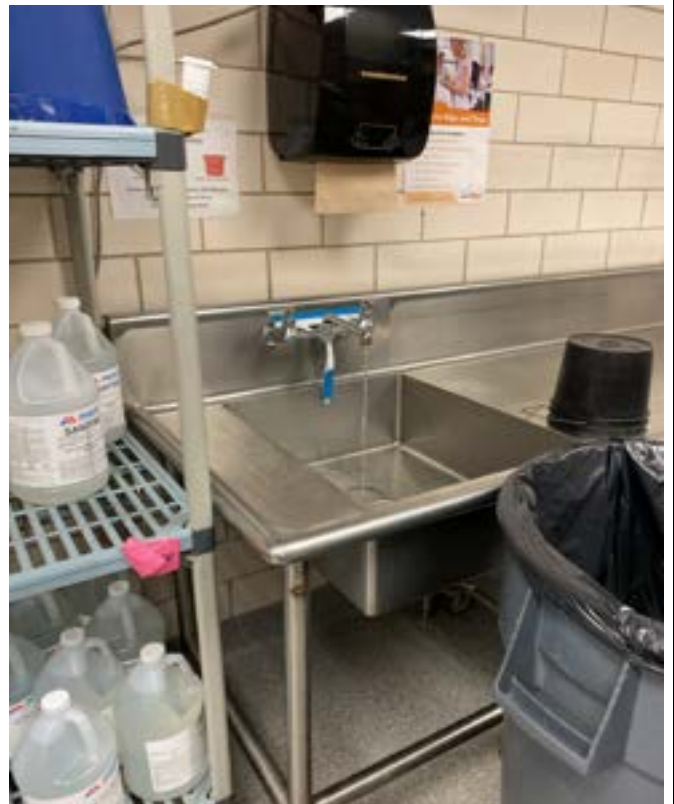
1/23/2024 - 2100-26 - Antioch Middle School - Kitchen-North Sink
