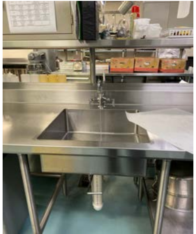
1/9/2024 - 3000-54 - Bell Prairie Elementary - Kitchen-West Sink
