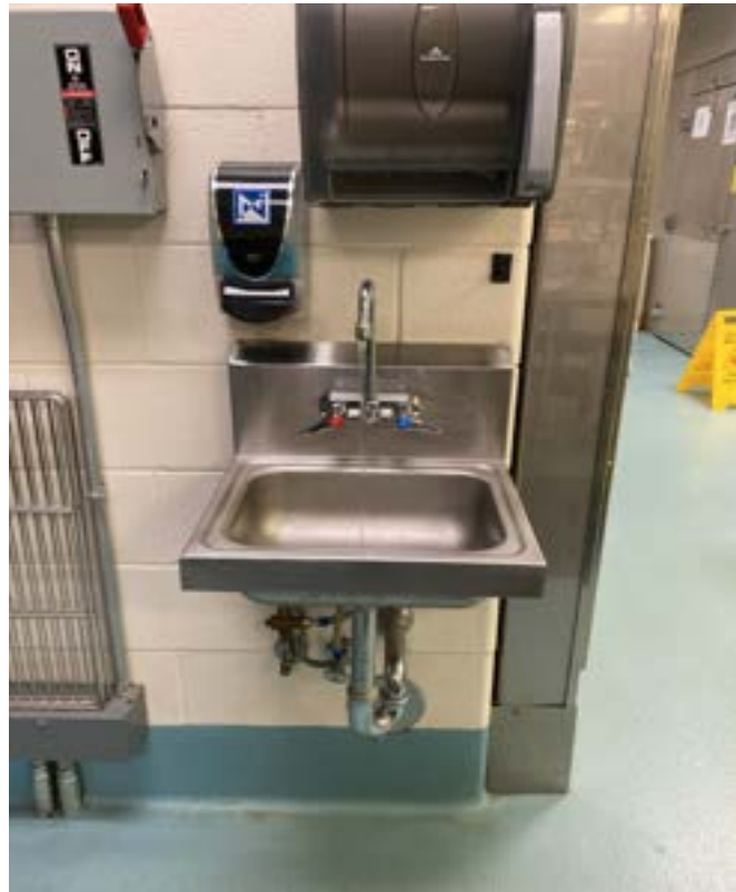
1/9/2024 - 3000-53 - Bell Prairie Elementary - Kitchen-West Handwashing
