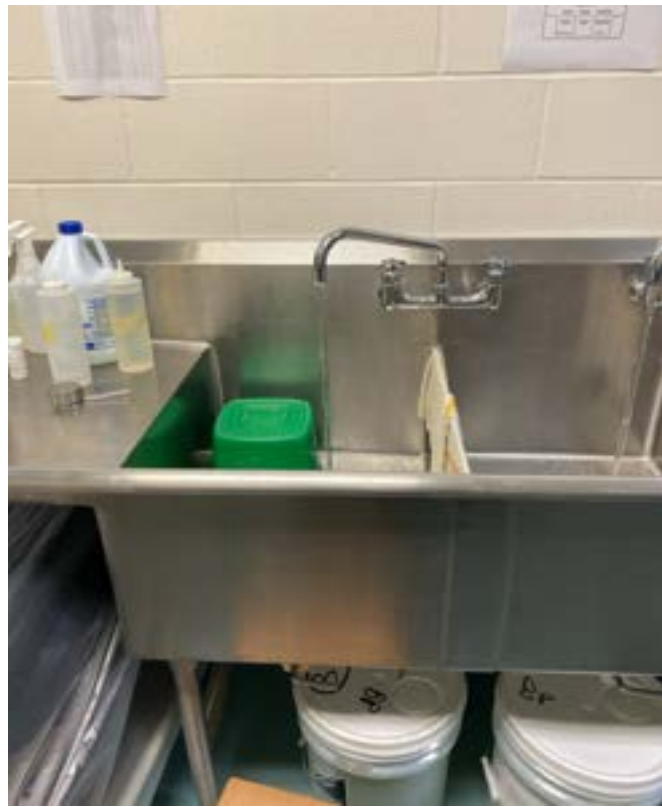
1/9/2024 - 3000-57 - Bell Prairie Elementary - Kitchen- Four Bay Sink-Left
