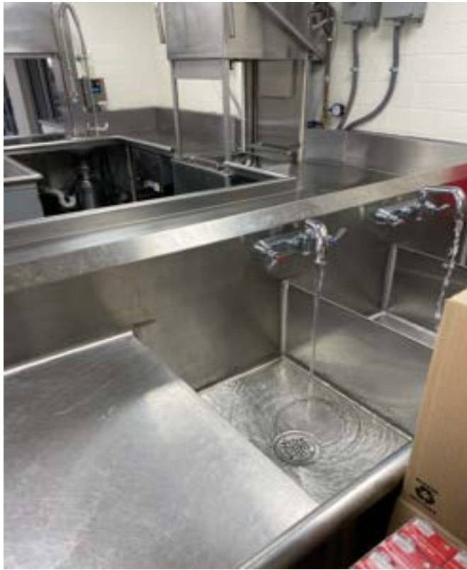
12/28/2023 - 4100-49 - Briarcliff Elementary - Kitchen-Northwest Sink-Left
