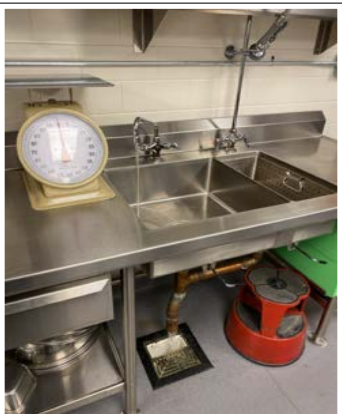
12/28/2023 - 4100-48 - Briarcliff Elementary - Kitchen-Northeast Sink
