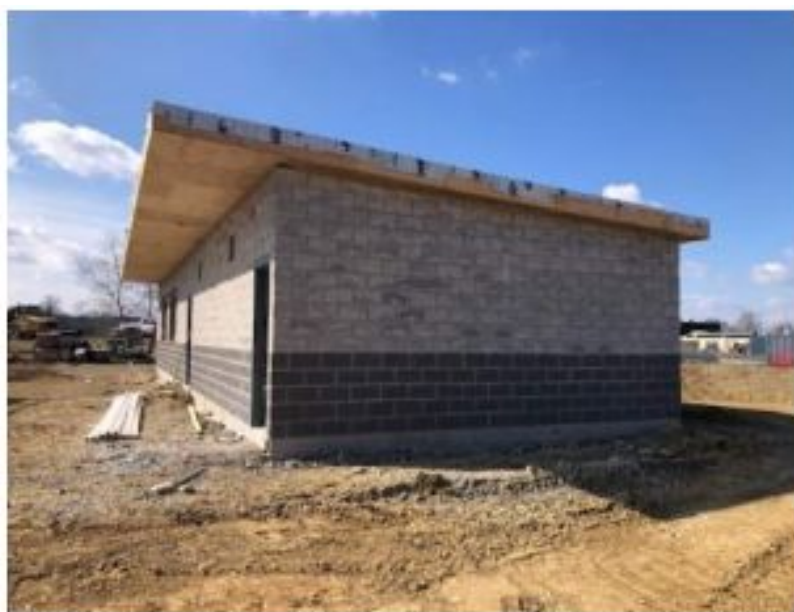
02.13.24 - Concessions Building, masonry and ice and water shield at roof are complete
