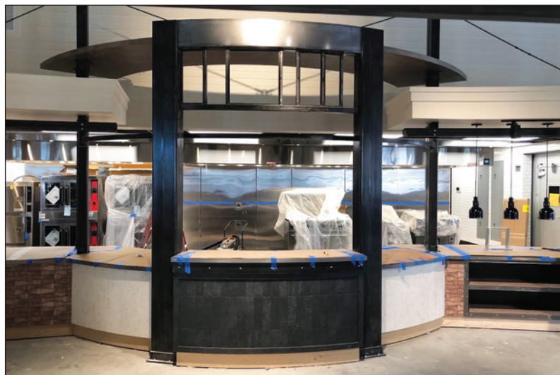
View of the central serving station. The larger kitchen and multiple serving areas will allow more variety in meal offerings.
