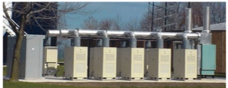
Microturbines are powered by natural gas and supply both electricity and ambient heat.
