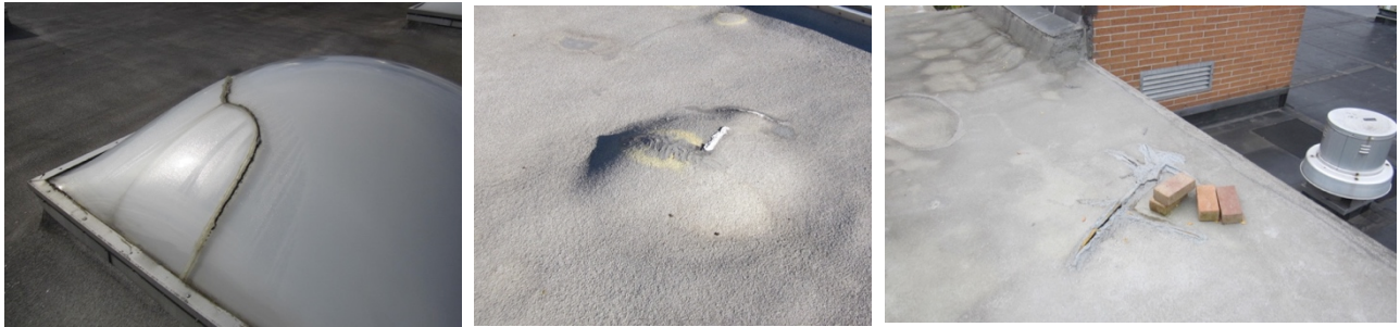
Roofs and skylights in all three schools (from left to right AHS, AMS and CRS)
