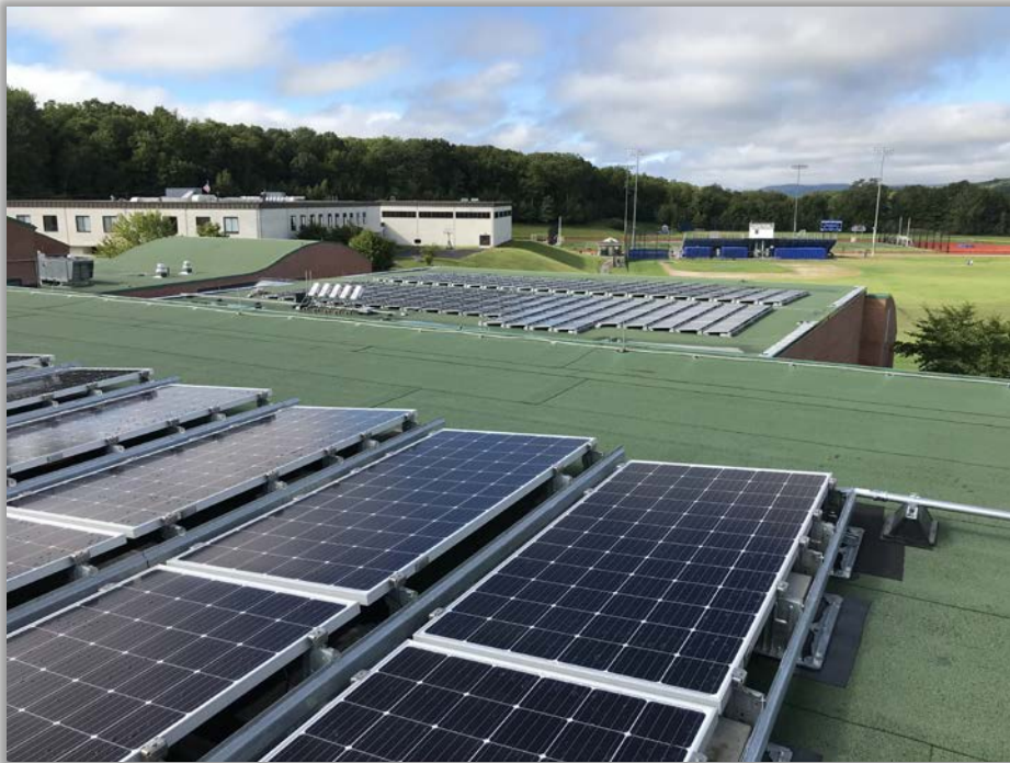
Example of Roof Top Solar
