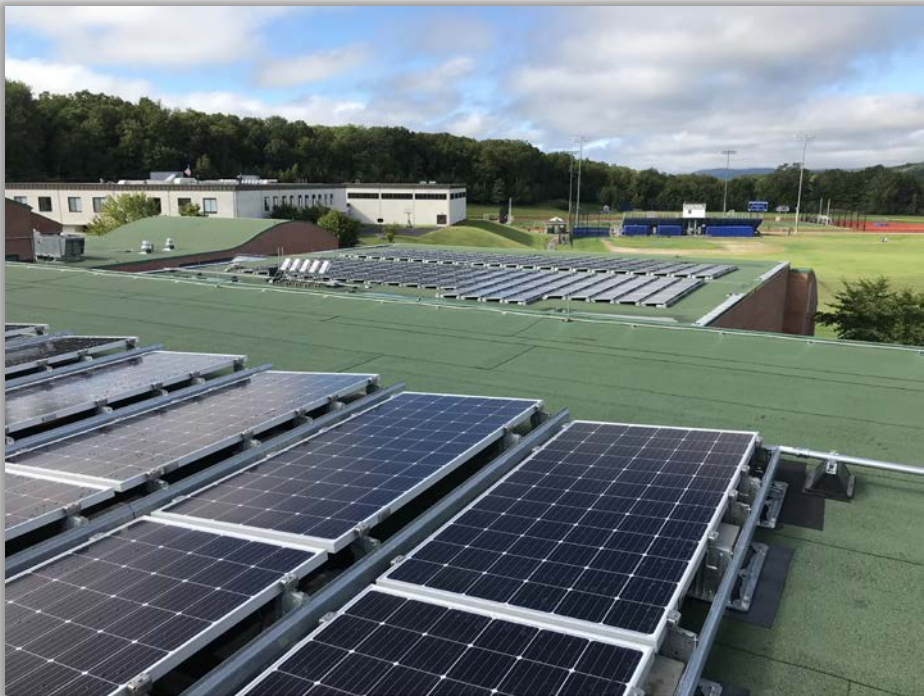
Example of Roof Top Solar
