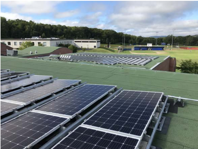
Example of Roof Top Solar
