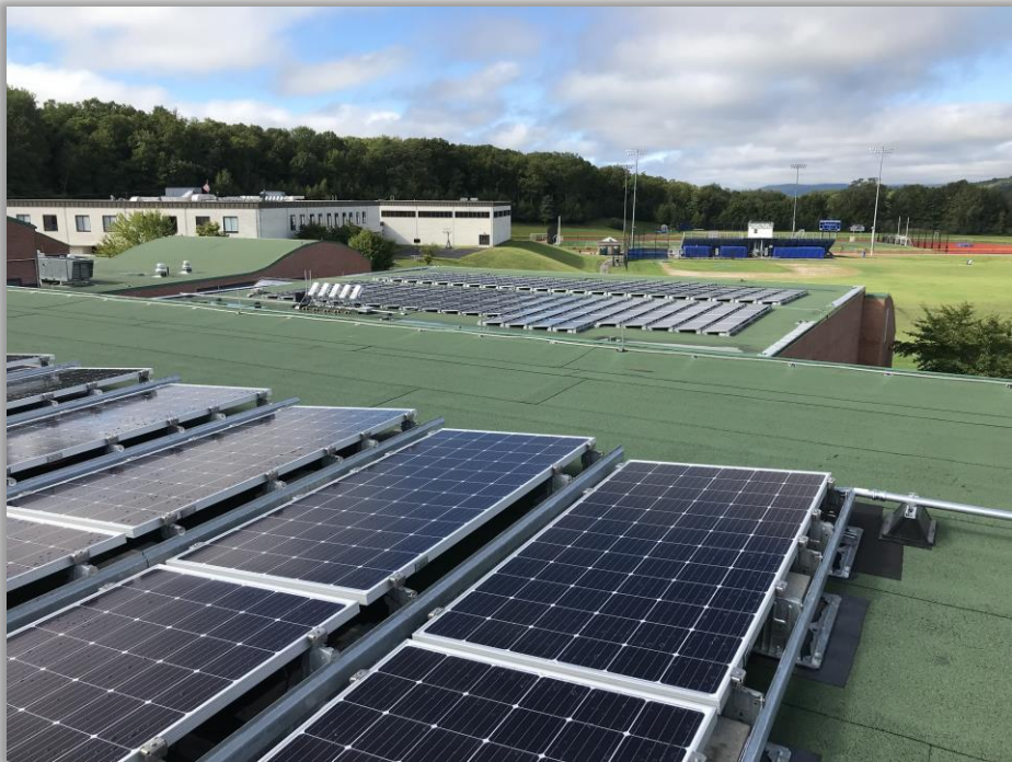
Example of roof top solar
