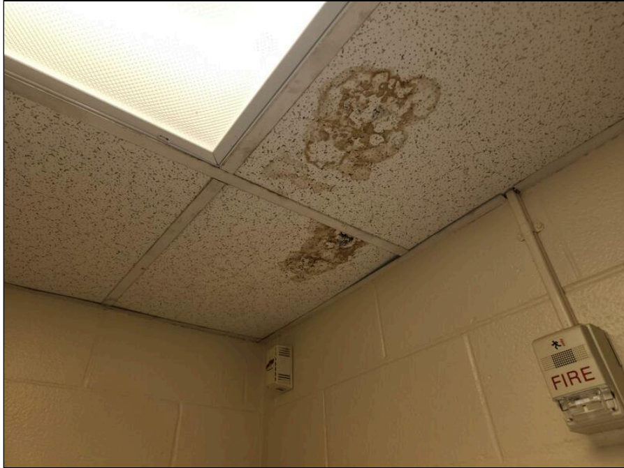
11 - Water and mold impacted ceiling tile in the Room 108 bathroom
