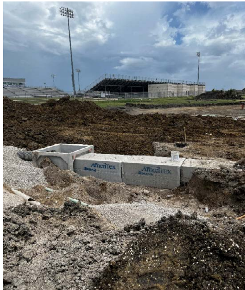
New student parking lot storm drains
