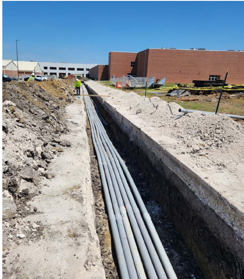
Electrical to multipurpose facility
