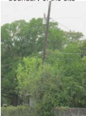
Photo 5 View of pole-mounted transformer on the northern boundary of the site
