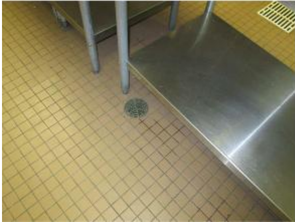
Photo 55 View of floor drain in the kitchen area of the cafeteria building
