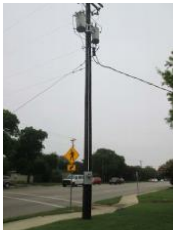
Photo 17 View of pole-mounted transformer on the western boundary of the site
