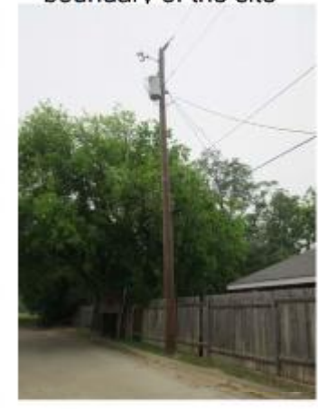
Photo 12 View of pole-mounted transformer on the eastern boundary of the site
