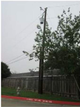
Photo 9 View of pole-mounted transformer on the eastern boundary of the site
