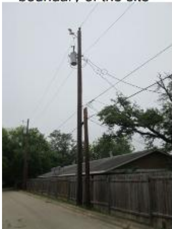
Photo 11 View of pole-mounted transformer on the eastern boundary of the site
