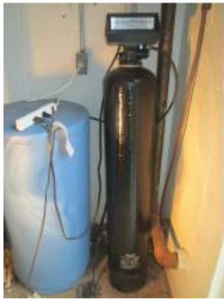
Photo 63 View of water softener system in the cafeteria building
