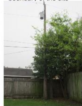
Photo 10 View of pole-mounted transformer on the eastern boundary of the site
