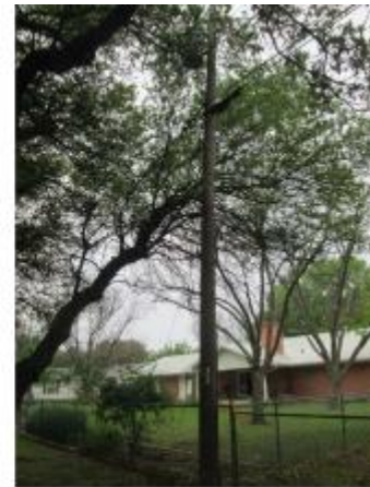
Photo 4 View of pole-mounted transformer on the northern boundary of the site
