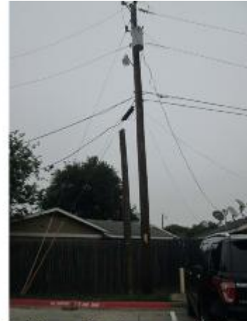
Photo 8 View of pole-mounted transformer on the eastern boundary of the site
