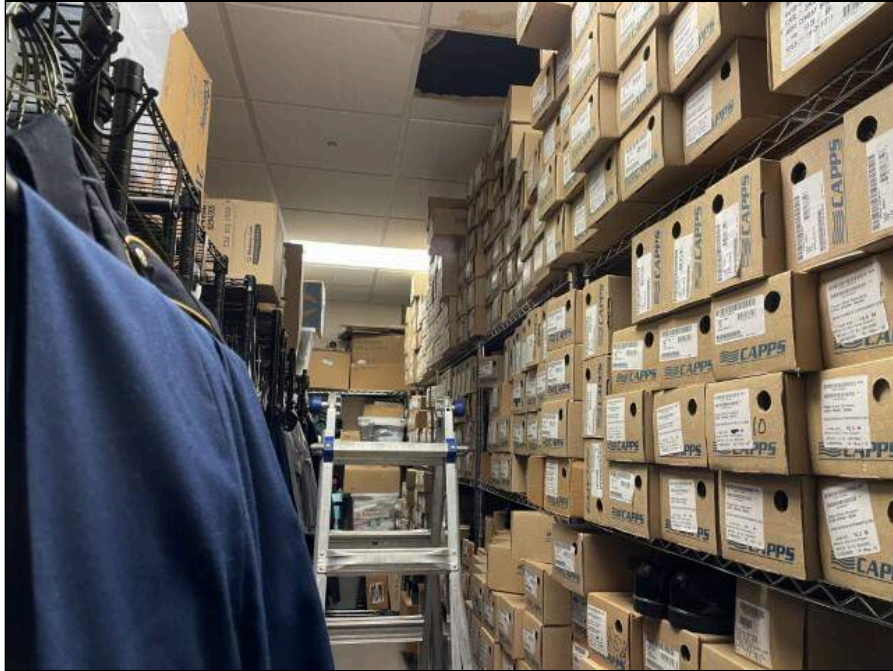
3 - Damaged and stained ceiling tiles in G-008B
