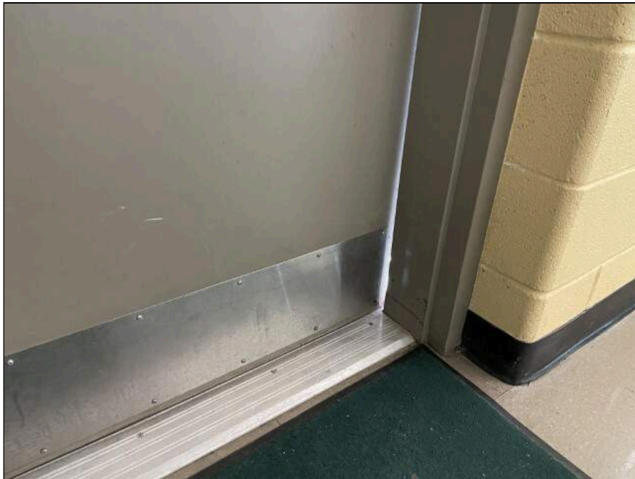
8 - Exterior door in G-007, poorly sealed
