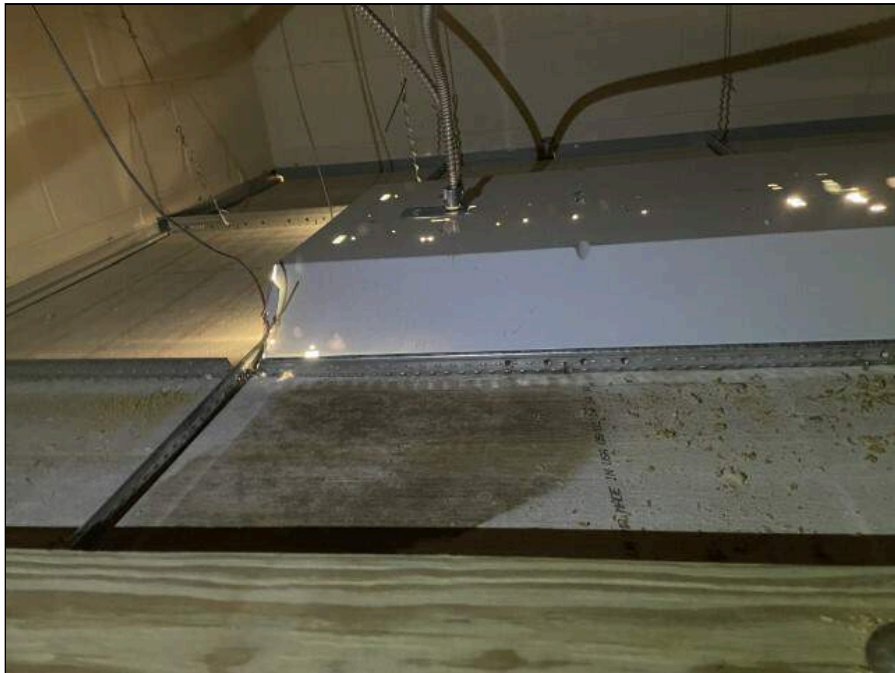
2 - Top of stained ceiling tile in G-008B
