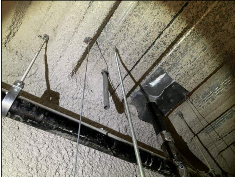
7 - Pipe affixed in roof, suspected source of moisture intrusion above ceiling tile in G-007
