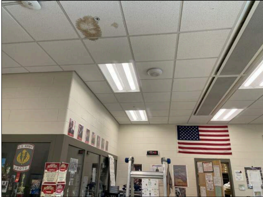
5 - Stained ceiling tiles in room G-007
