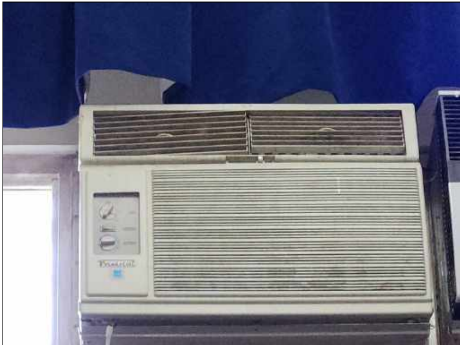
18 - Mold on a window mounted A/C unit in the Auditorium
