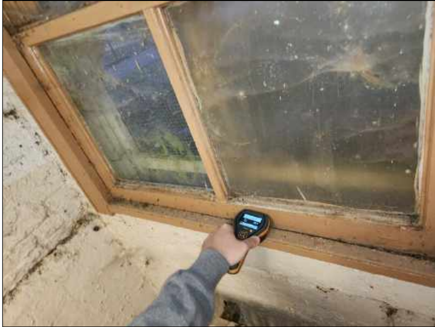
3 - Elevated moisture meter reading collected from a wood window sash in the basement of the original building
