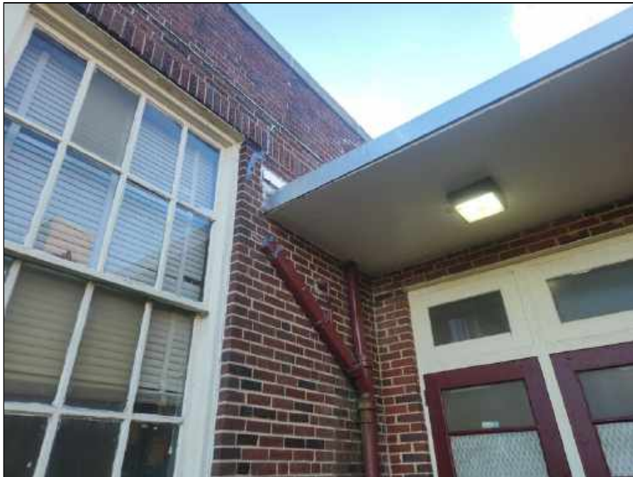
4 - Disconnected gutter outside room 14 likely causing water damaged plaster wall
