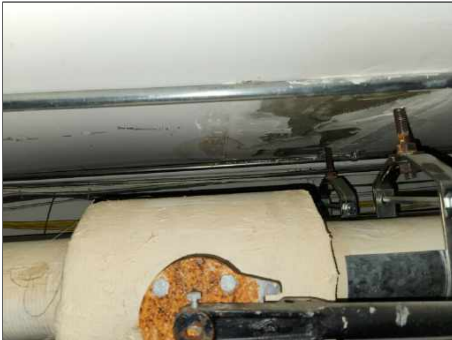
20 - Mold impacted plaster ceiling outside the electrical room
