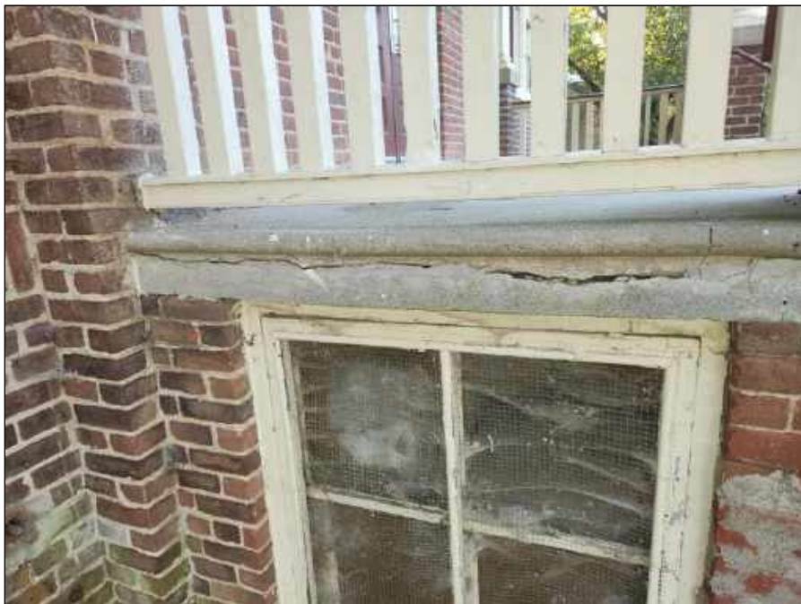
2 - Cracked concrete porch on the North side of the original building
