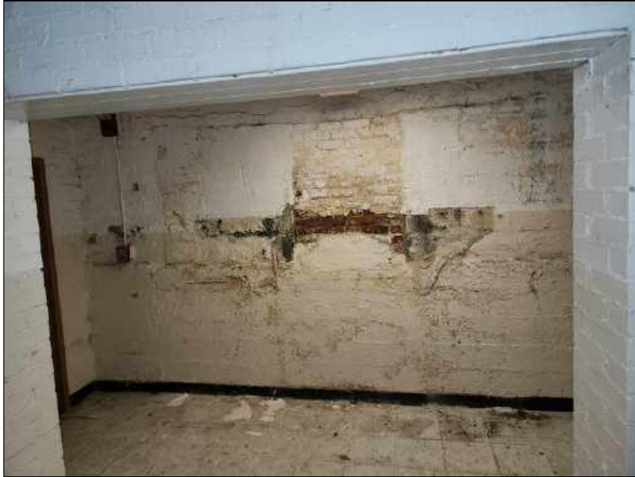
5 - Mold on the wall in the basement hallway
