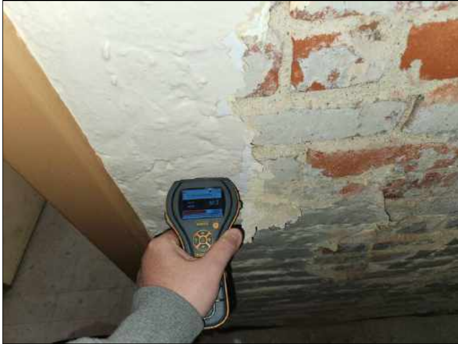
1 - Elevated moisture meter reading collected from plaster in the basement of the original building
