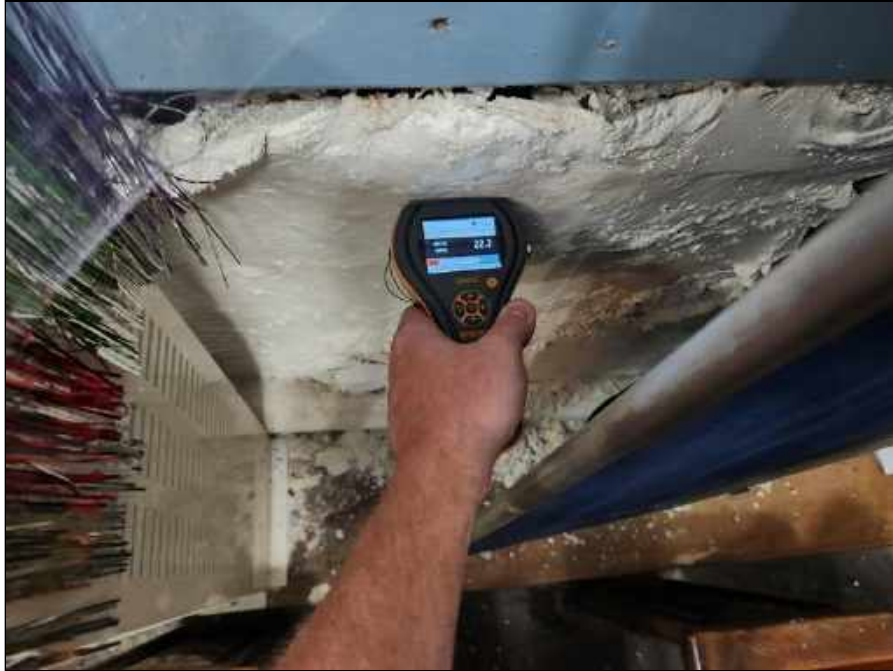
13 - Moisture damaged plaster wall in the Auditorium
