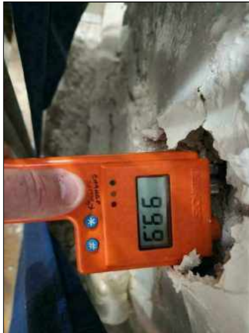
14 - Wet moisture meter reading collected from the damaged plaster wall
