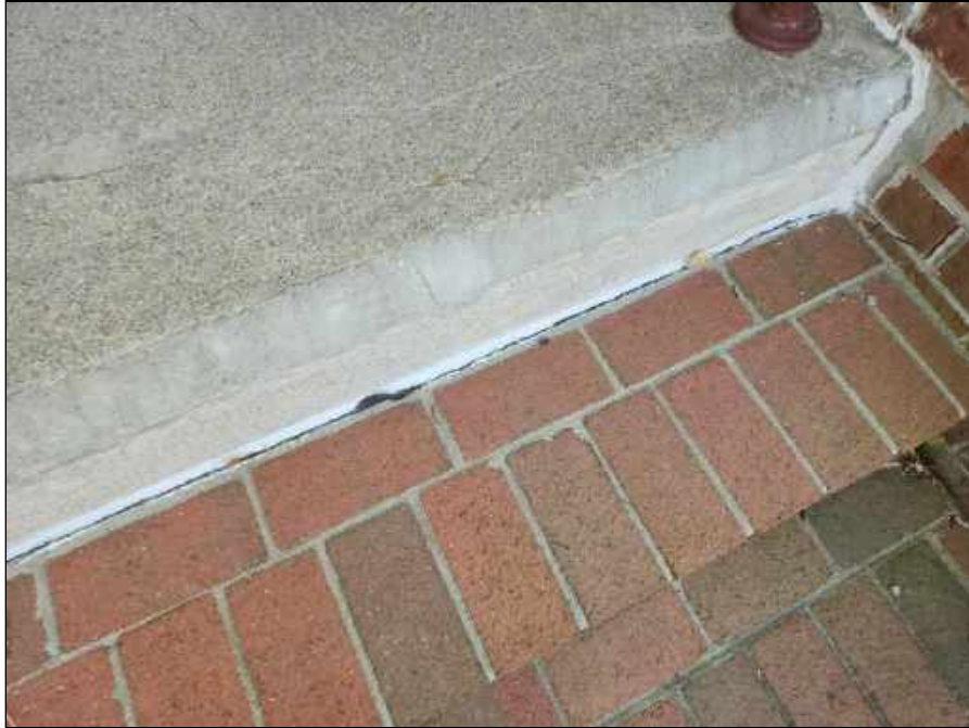
3 - Area where porch step is separating and likely a cause of water intrusion into the basement
