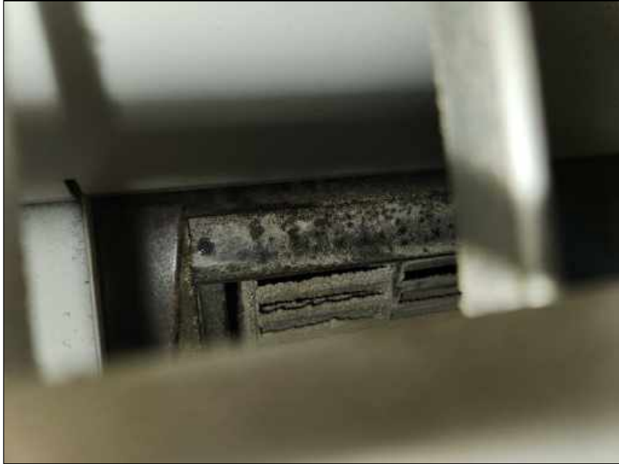
19 - Mold within the ceiling mounted fan coil in Room 10
