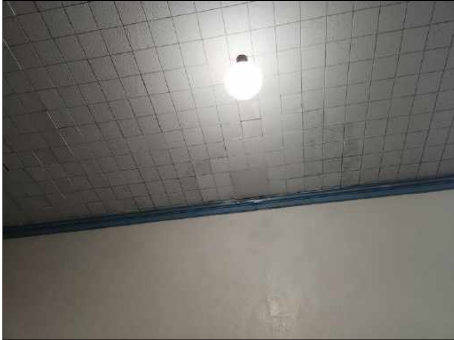
17 - Moisture impacted ceiling tiles and plaster wall in the Auditorium
