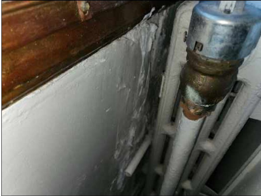
21 - Damaged plaster wall in Room 14
