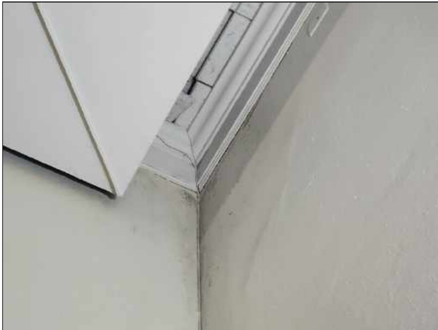
12 - Mold on the plaster wall - left section of the stage
