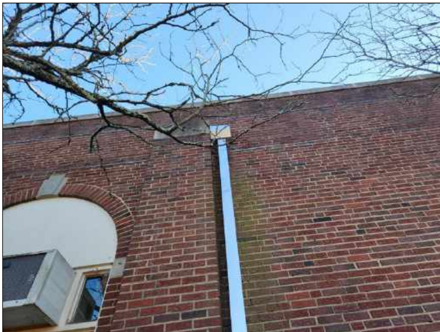
8 - Staining on the brick wall around the downspout indicating the water is running down the wall outside the Auditorium
