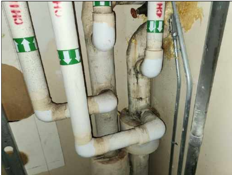
10 - Mold on pipe insulation in a pipe chase on the upper level of the original building
