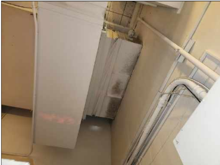
16 - Mold on an HVAC duct above the stage
