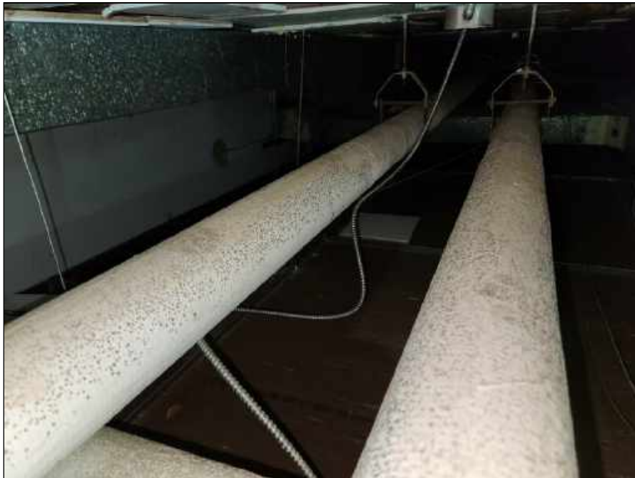
22 - Surface mold on pipe insulation above the ceiling in the South hallway
