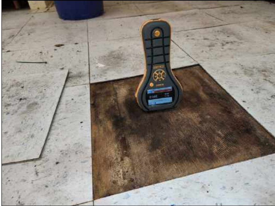
7 - Elevated moisture meter reading and mold on the sub-floor in Room 15 in the original building
