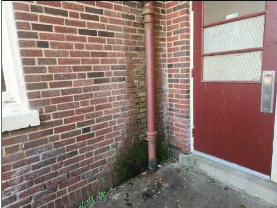
1 - Staining on the brick wall around the downspout indicating the water is running down the wall outside Room 14
