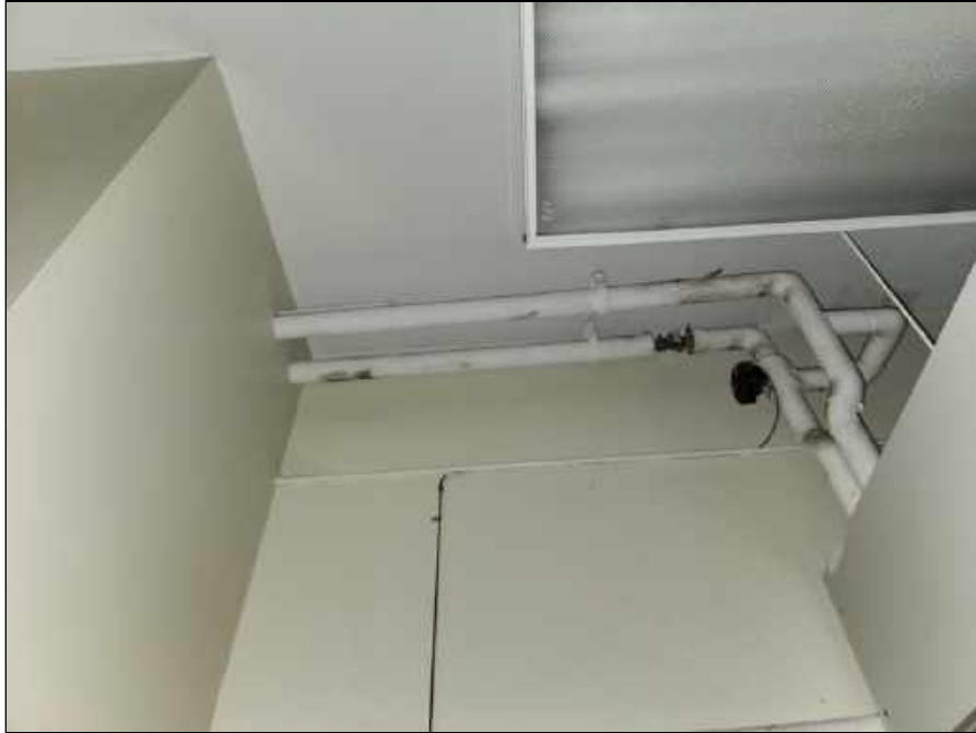
9 - Mold on pipe insulation in a room on the upper floor of the original building
