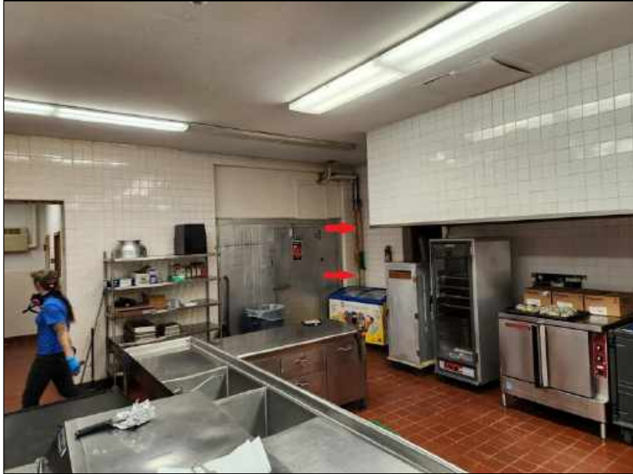
25 - Mold on pipe insulation in the kitchen
