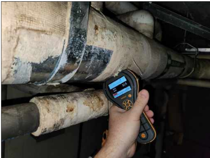
4 - Elevated moisture meter reading collected from pipe insulation in the basement of the original building
