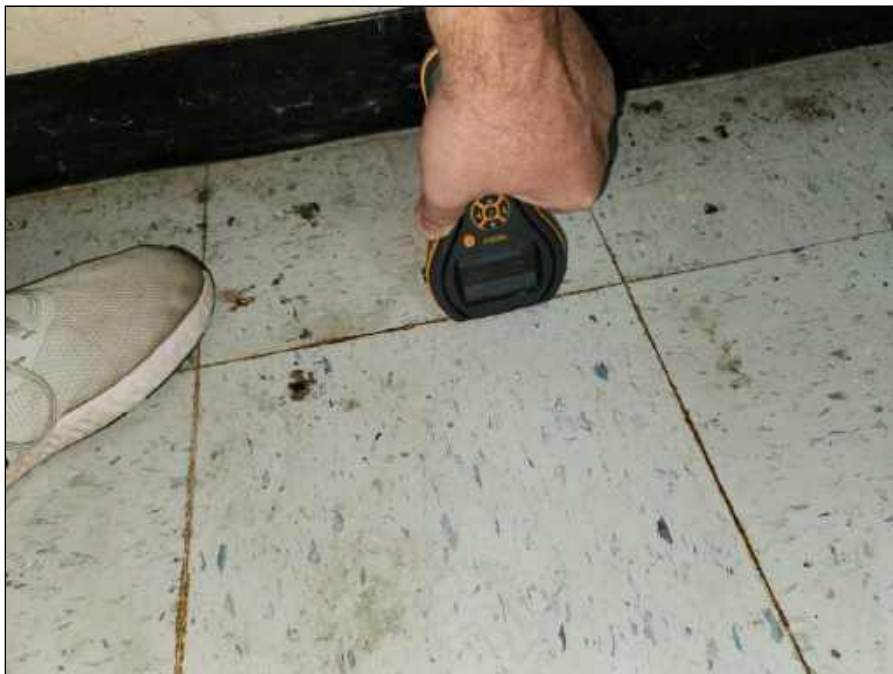
2 - Elevated moisture meter reading collected from flooring in the basement of the original building
