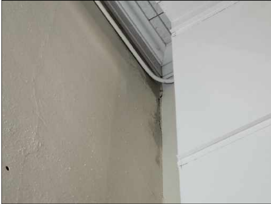
11 - Mold on the plaster wall - right section of the stage
