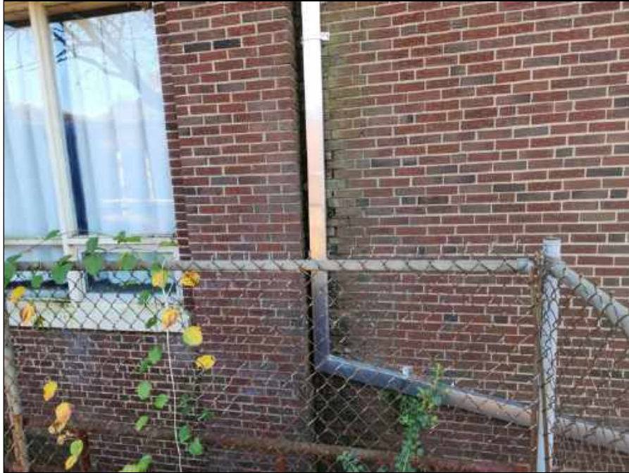
7 - Staining on the brick wall around the downspout indicating the water is running down the wall outside the Auditorium
