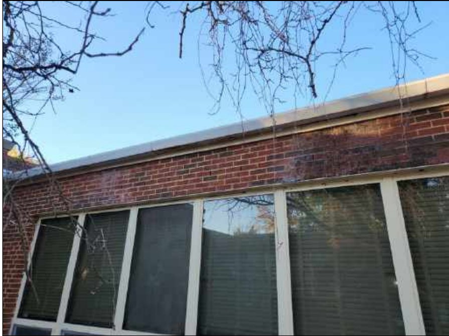
9 - Staining on the exterior wall in the courtyard outside Room 5
