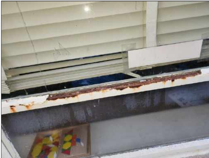
6 - Rusted window sash mullion and damaged window sash glazing on the South side of the building
