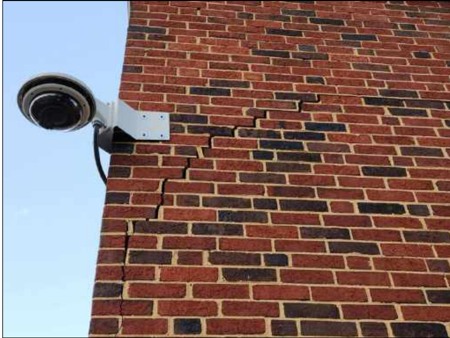
5 - Brick wall separating in the Southwest corner of the building outside room 9
