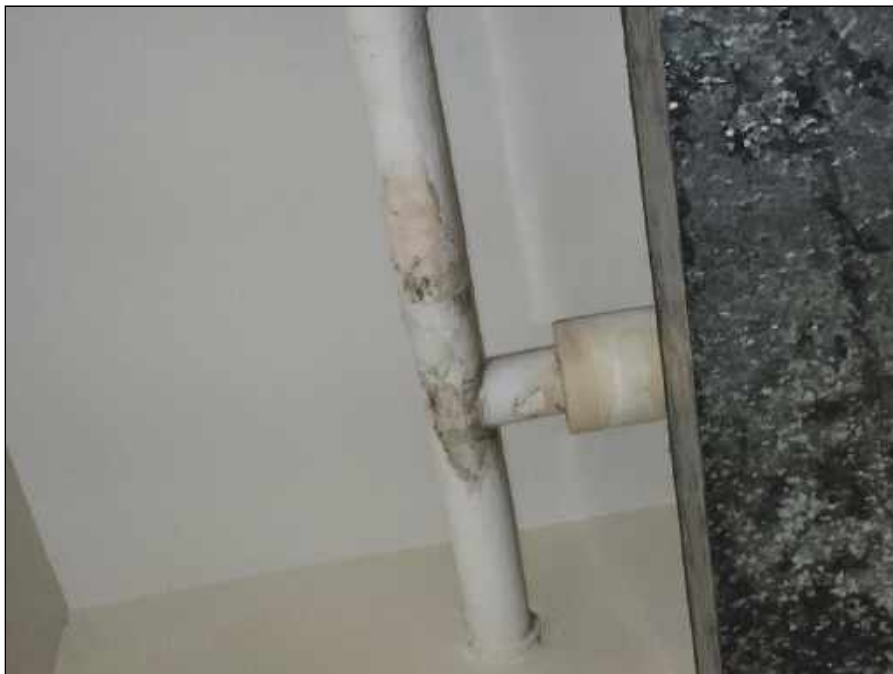
8 - Mold on pipe insulation in a room on the upper floor of the original building
