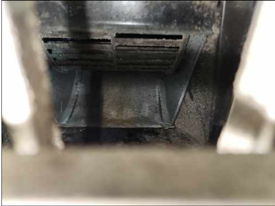
23 - Mold within the window mounted A/C unit in Room 9
