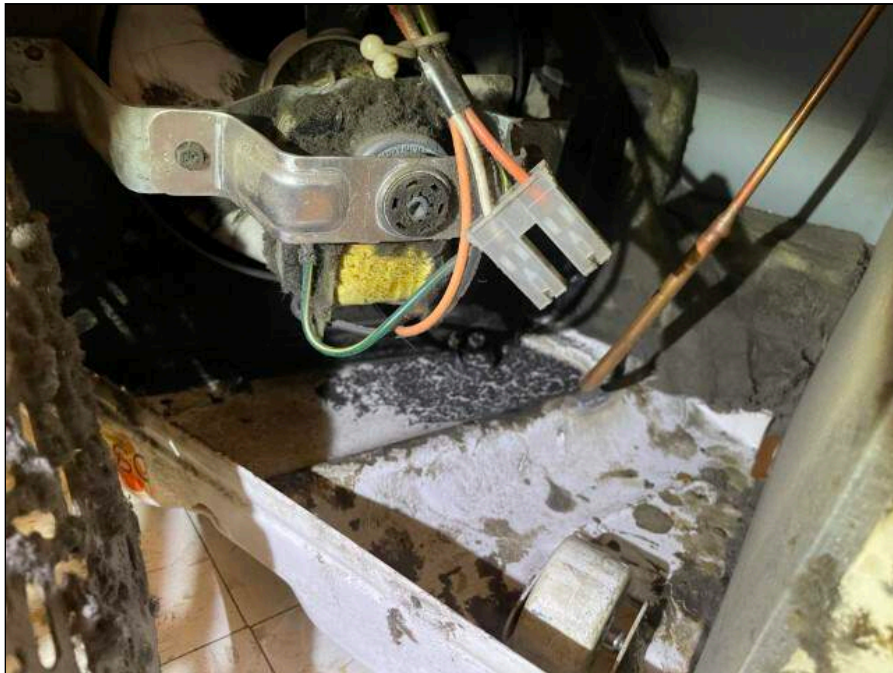
6 - Mold observed within the back of a refrigerator in Room 235
