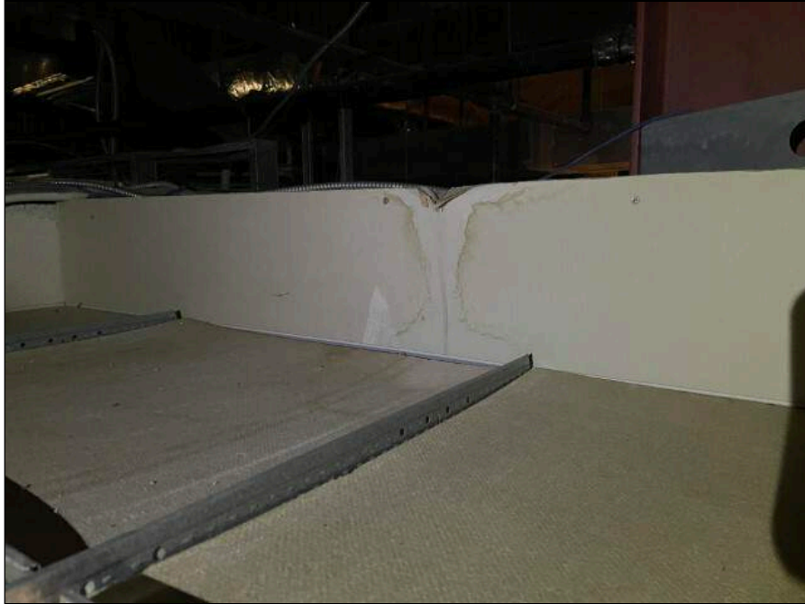
13 - Moisture Damaged Drywall Above the Ceiling in the NE Corner of the Media Center
