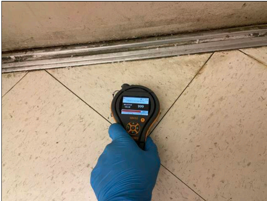
10 - Elevated Relative Moisture Meter Reading at the back door in Room 118
