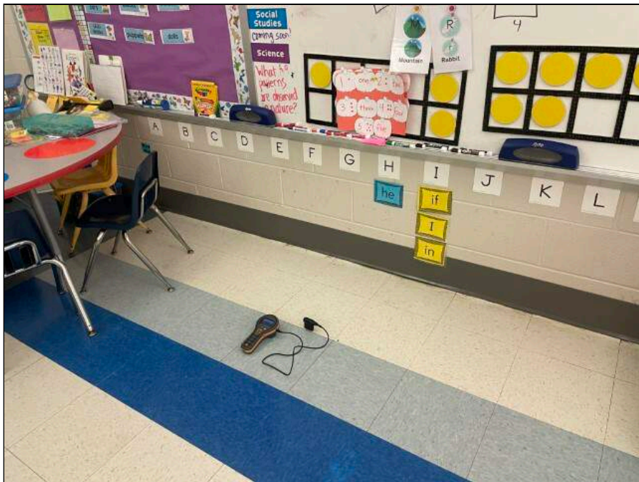
8 - Damaged Floor Tile Along the North Perimeter Wall in Room 105
