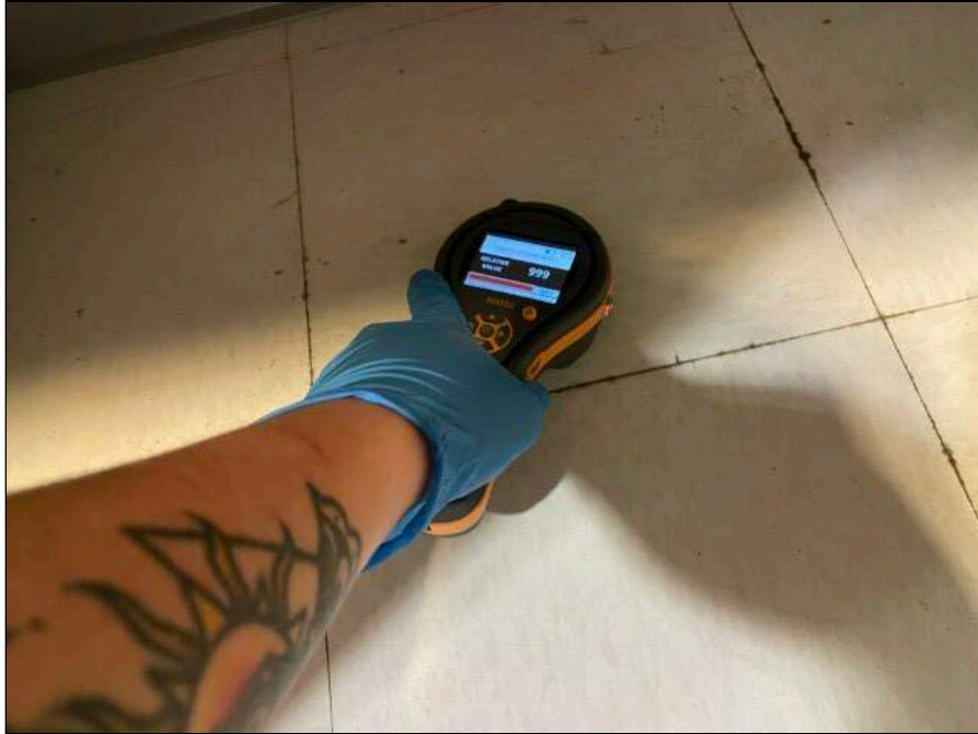
5 - Elevated Relative Moisture Meter reading Beneath the Sink in the Office Break Room
