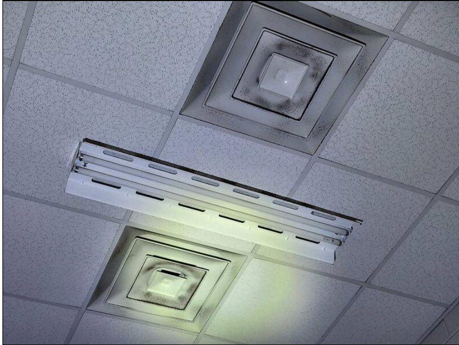
3 - Mold on the Diffusers in the Gym Equipment Storage Cage
