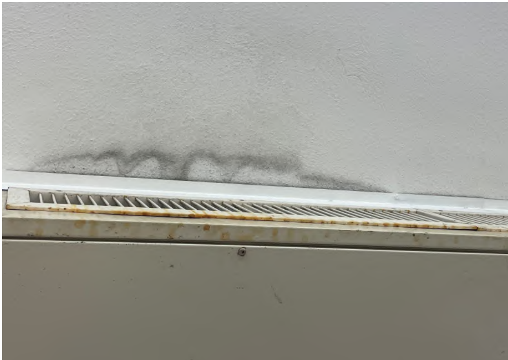
Photograph No. 2 Showing Typical Mold Impacted Ceiling Mounted HVAC Units & Moisture Staining
