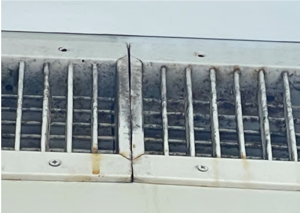
Photograph No. 1 Showing Typical Mold Impacted Ceiling Mounted HVAC Units
