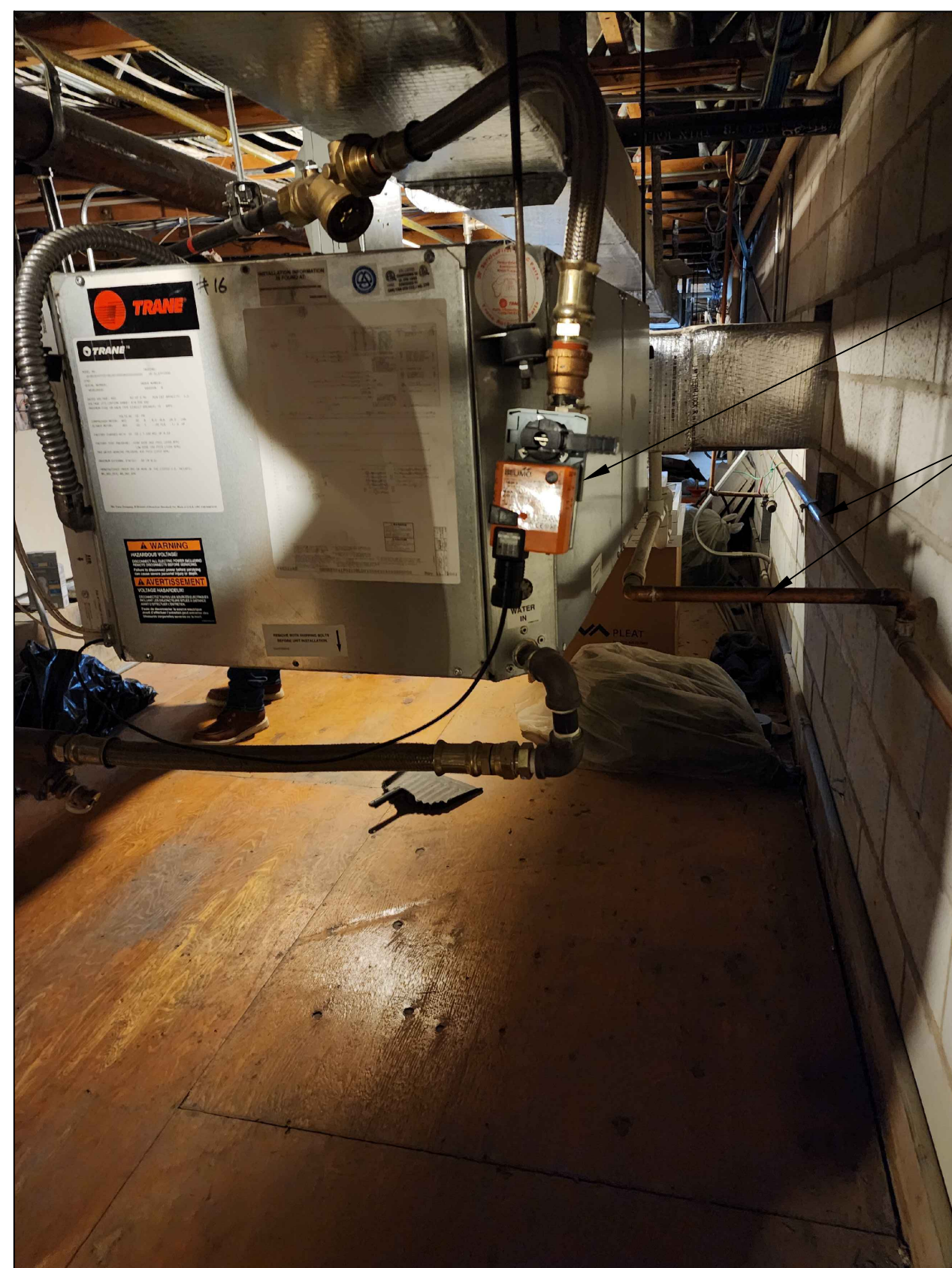
TYPICAL EXISTING HEAT PUMP
