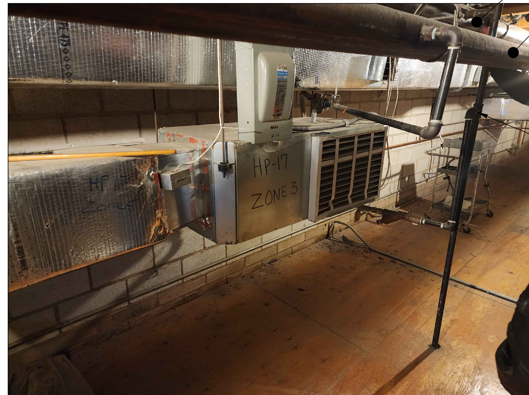
TYPICAL EXISTING HEAT PUMP
