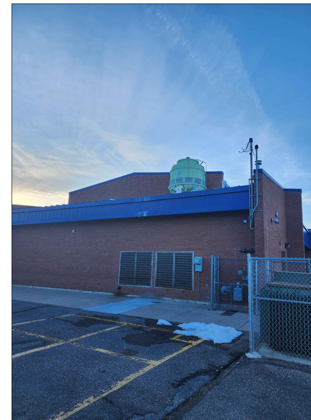
EXISTING COOLING TOWER
