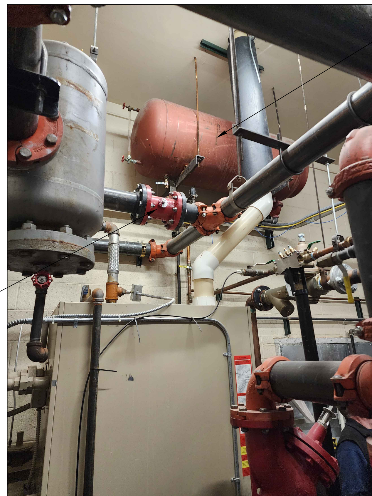
EXISTING MECHANICAL ROOM
