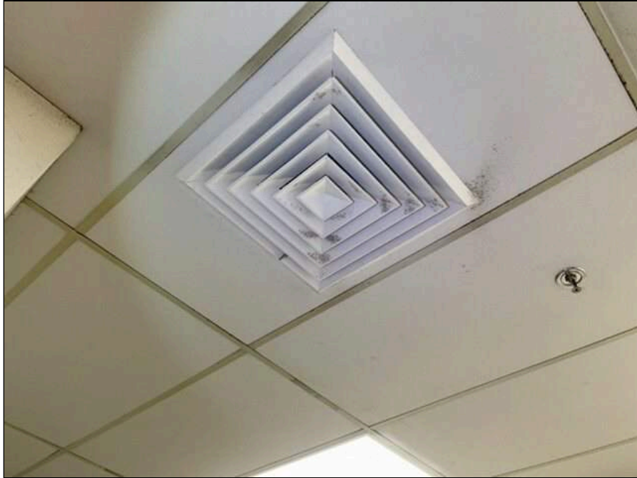
9 - View of Kitchen vent with heavy dust observed.
