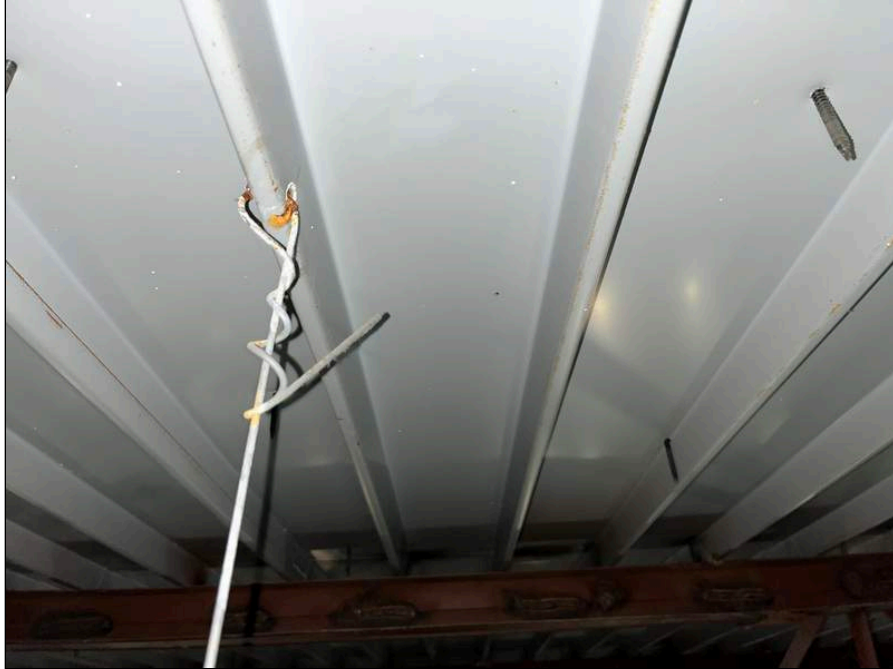
5 - View of ceiling tile wire hanger with moisture and rust observed where it goes through the ceiling deck.
