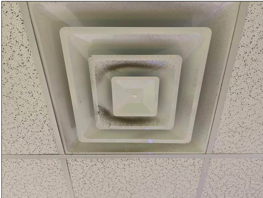
6 - View of supply vent with heavy debris observed.
