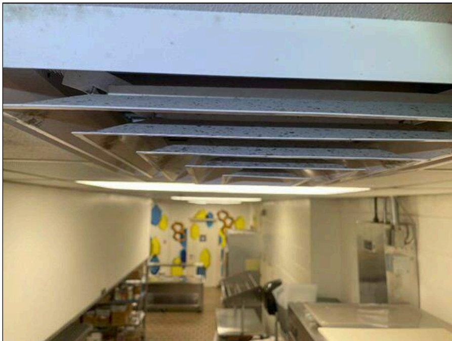
10 - Close view of of kitchen vent with suspect mold observed.
