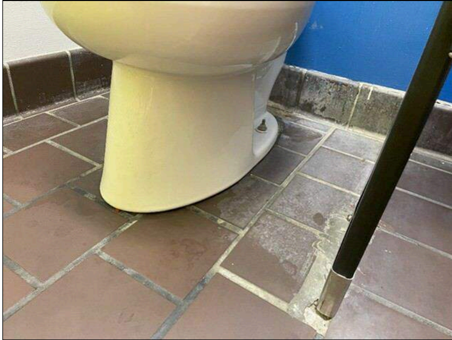
7 - View of bathroom with water staining observed.
