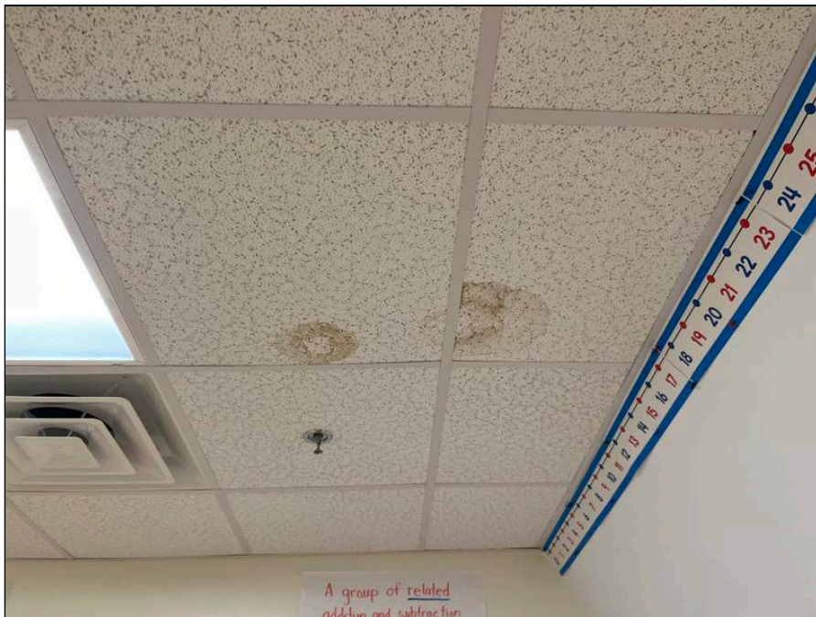
4 - General view of stained ceiling tile which were observed sporadically throughout the school
