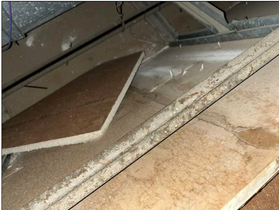
2 - View of rear side of the gypsum board which had water staining in room 110
