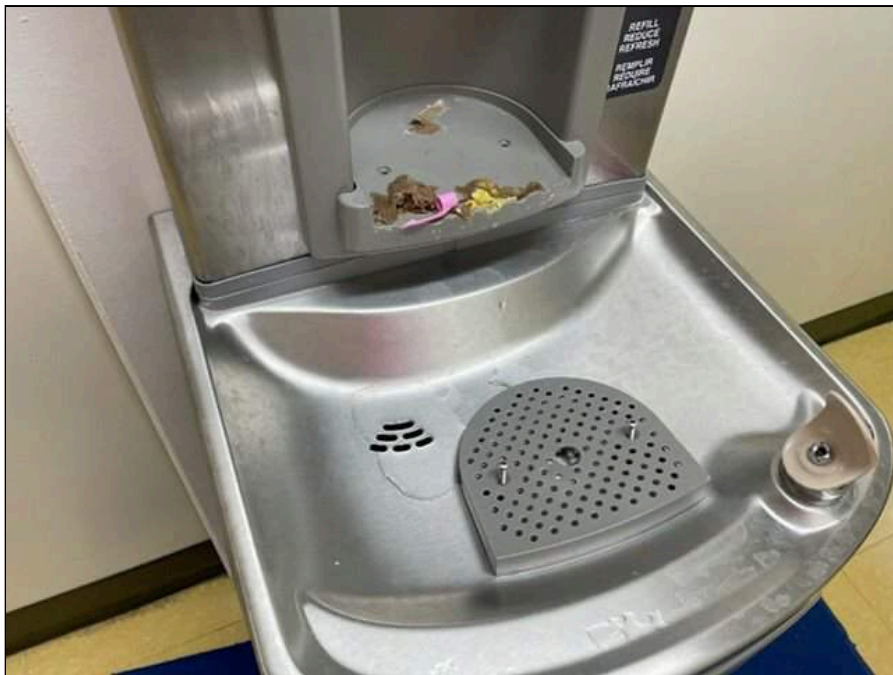
8 - View of bottle filler with debris and staining from overflow.
