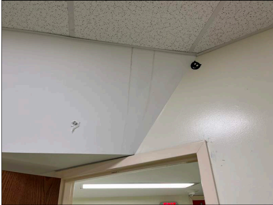
1 - View of water stain on the gypsum board located within room 110.
