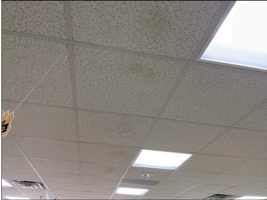
3 - General view of stained ceiling tile which were observed sporadically throughout the school
