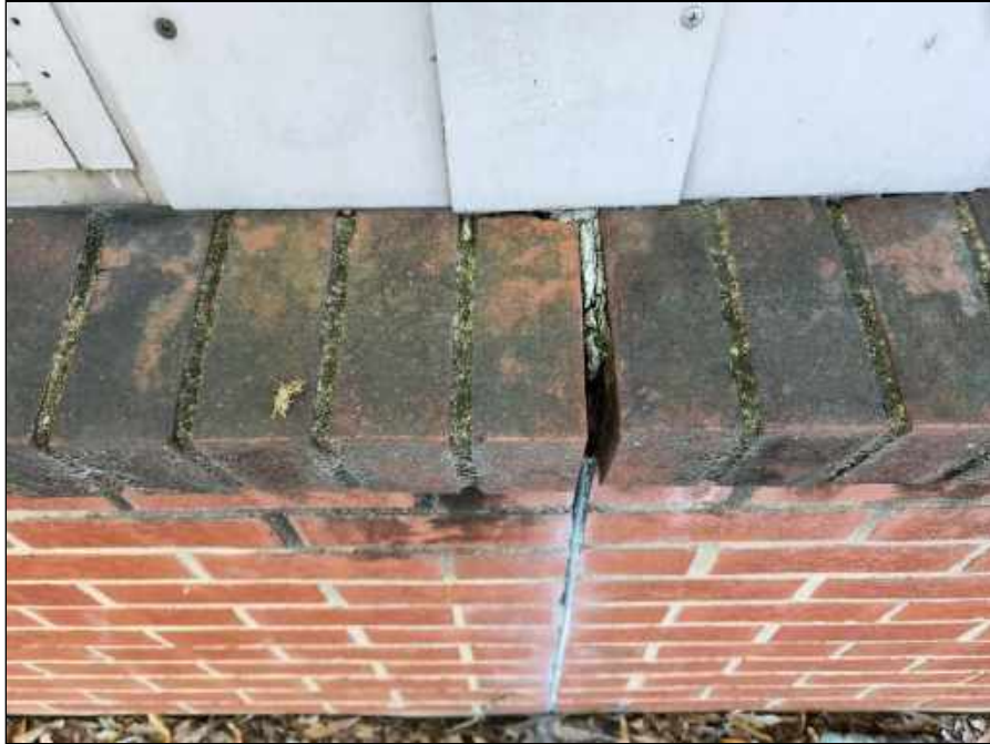
3 - Damaged Window Ledge Sealants
