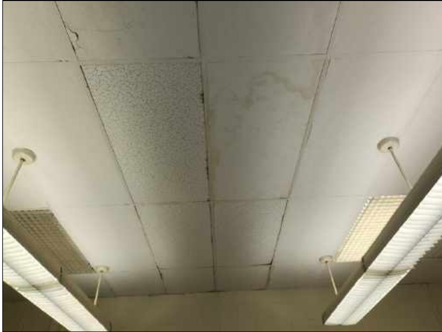
15 - Moisture Stained Ceiling Tiles in Room 108
