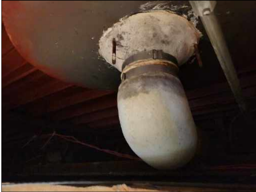
3 - Mold Impacted Roof Drain Collar and Mudded Elbow Above the Teacher's Lounge
