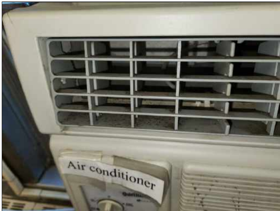
14 - Mold on the Window Mounted A/C Unit in Room 111
