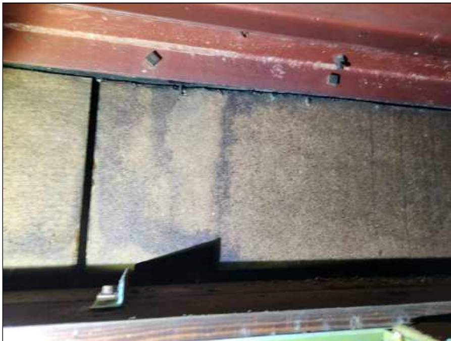
4 - Moisture Impacted Particle Board Soffit Materials in the Teacher's Lounge
