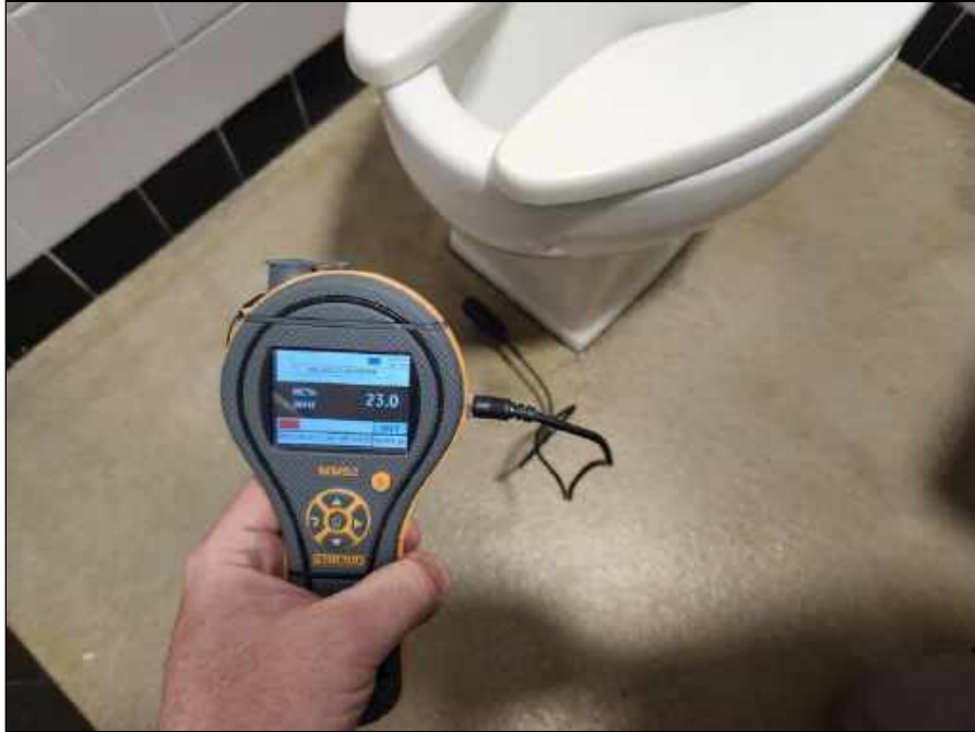
17 - Elevated Moisture Meter Reading Indicating Elevated Moisture Beneath the Sheet Flooring in the Room 105 Bathroom
