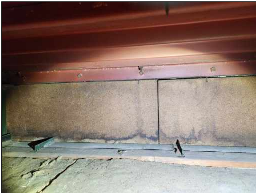
6 - Moisture Impacted Particle Board Soffit Material in Room 102
