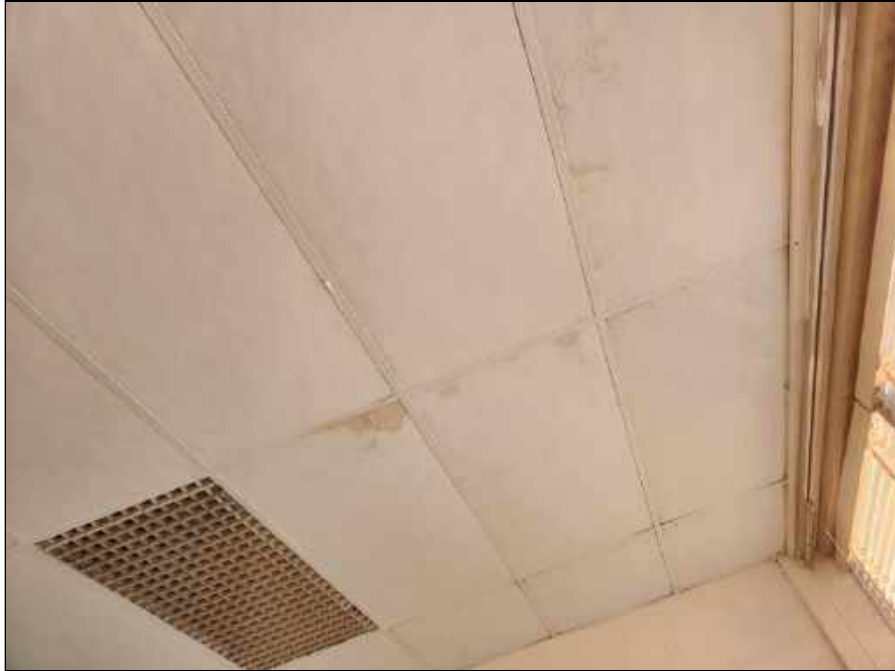
7 - Water Stained Ceiling Tiles in the Teacher's Lounge
