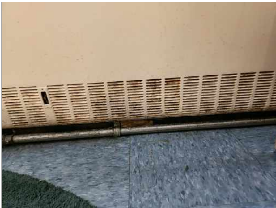
12 - Dust and Dirt Buildup on the Fan Coil Unit in the Teacher's Lounge
