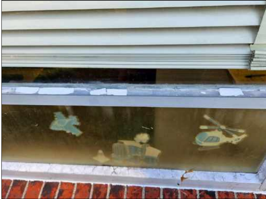
1 - Damaged Window Sash Glazing
