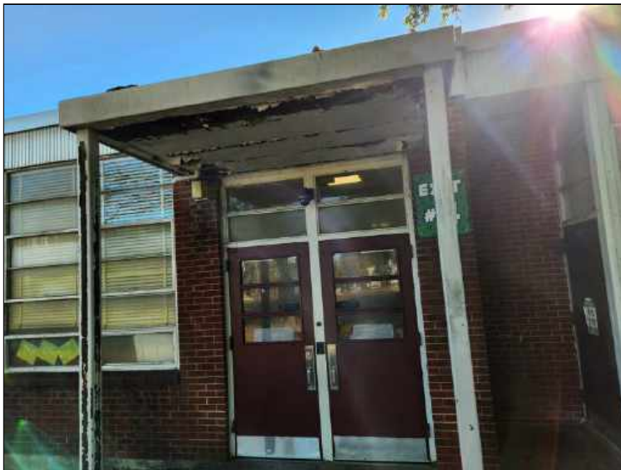
6 - Damaged Exterior Portico on the East Wing of the Building
