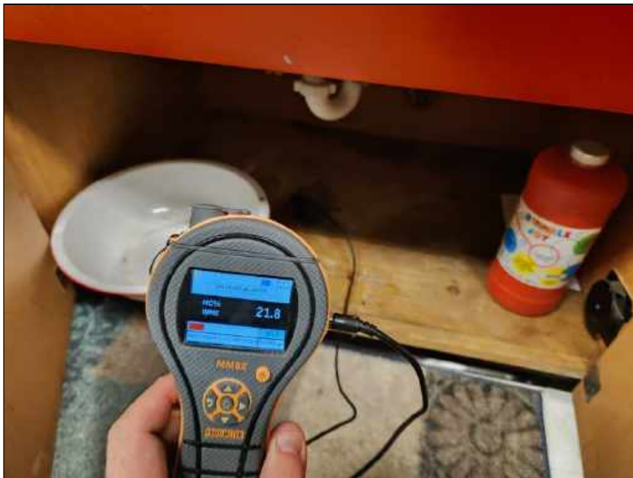
10 - Elevated Moisture Meter Reading in the Sink Vanity in the Office
