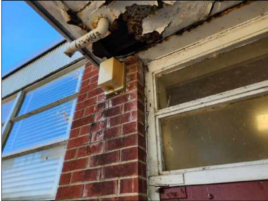
7 - Evidence of Moisture Intrusion Through the Portico Roof
