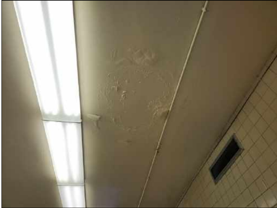
1 - Moisture Impacted Plaster Ceiling in the Kitchen
