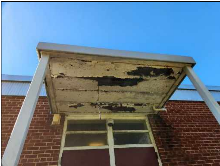
8 - Moisture Damaged Exterior Portico on the East End of the School
