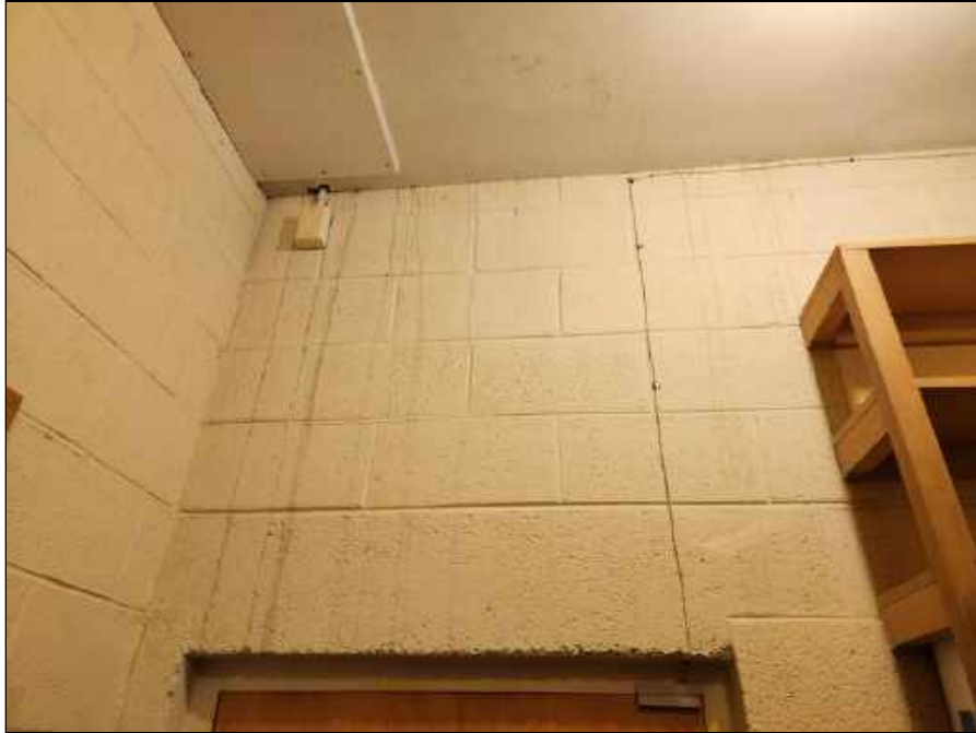
9 - Moisture Stained Plaster Ceiling in the Office
