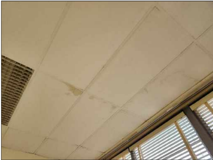
8 - Water Stained Ceiling Tiles in Room 100
