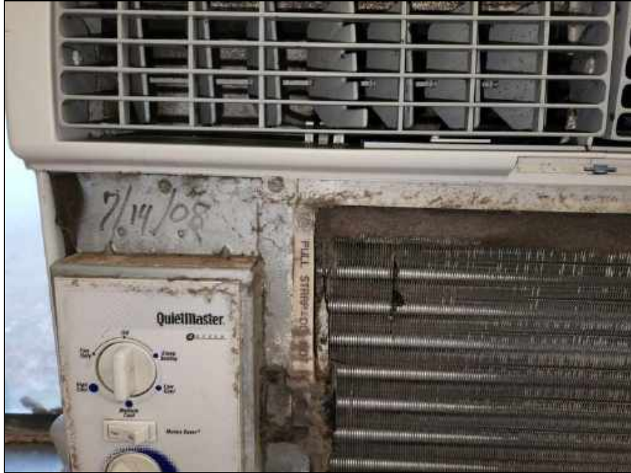
13 - Mold on the Window Mounted A/C Unit in Room 113
