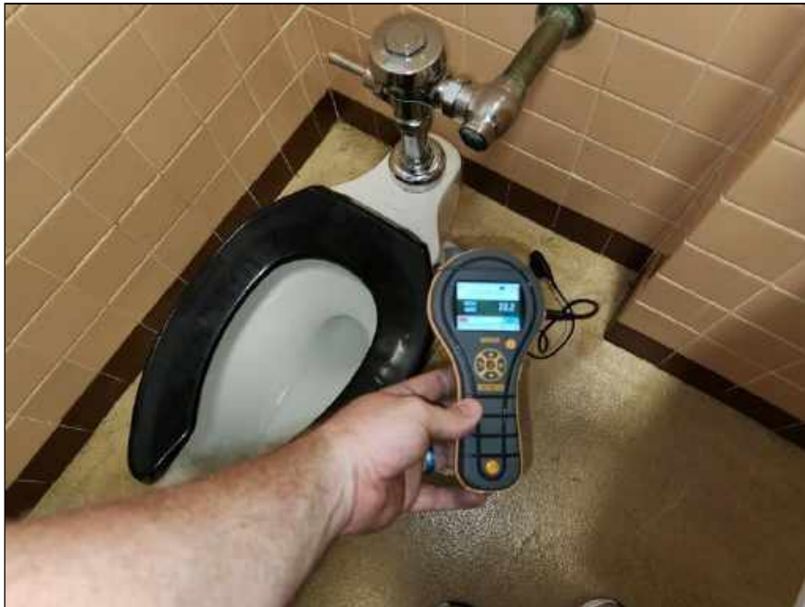
16 - Elevated Moisture Meter Reading Indicating Elevated Moisture Beneath the Sheet Flooring in the Room 110 Bathroom
