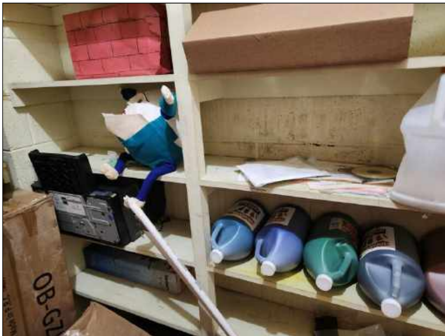
18 - Mold on the CMU Walls in the Book Room
