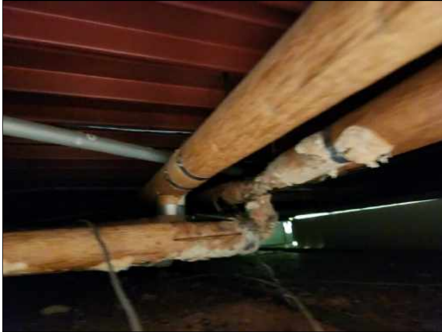
11 - Damaged Asbestos Containing Mudded Pipe Fitting Above the Nurse's Office
