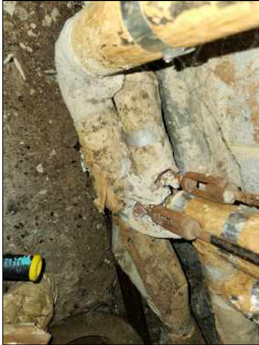
21 - Mold and moisture impacted pipe insulation and mudded elbows in the bathroom wet wall chase
