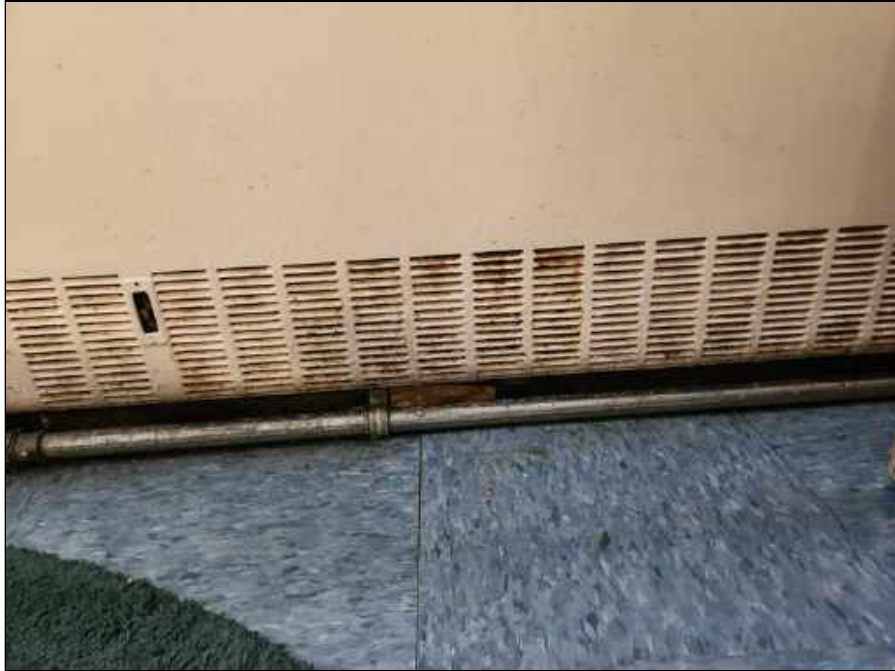
5 - Dust and Dirt Buildup on the Fan Coil Unit in Room 100
