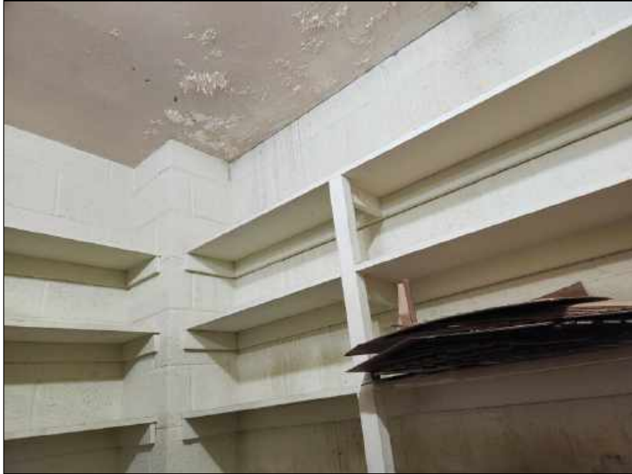
19 - Moisture Damaged Plaster Ceiling and Mold Impacted Materials in the Book Room
