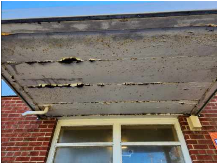
2 - Moisture Damaged Exterior Portico on the North Side of the Building
