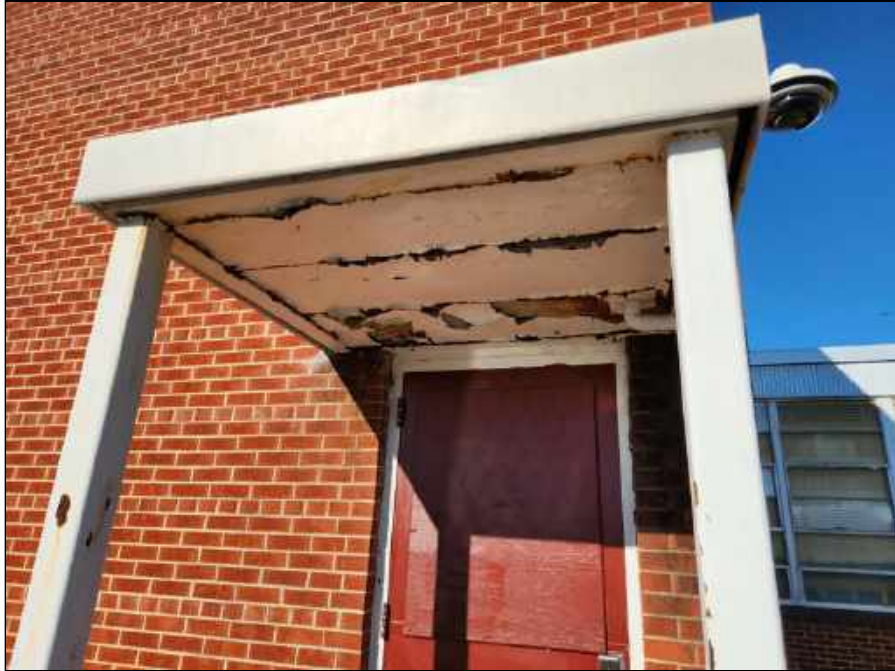
9 - Moisture Damaged Exterior Portico at the Cafeteria
