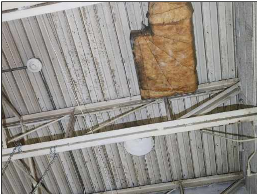
20 - Mold Observed on the Roof Deck in the Auditorium
