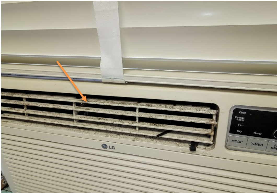
Photograph No. 2 Showing Visible Mold Growth - Office 101A
