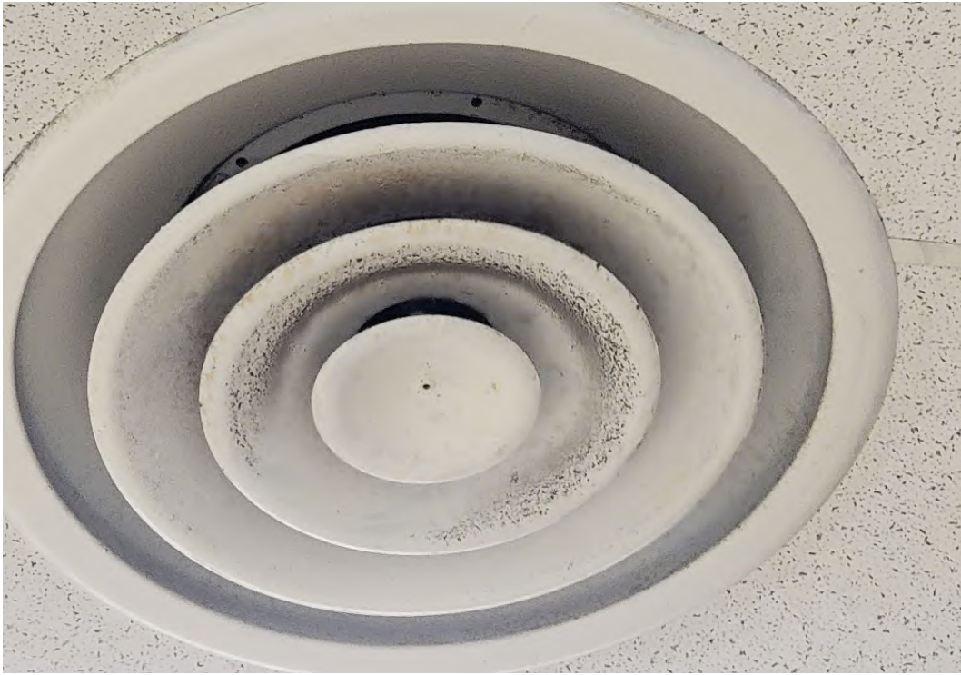
Photograph No. 3 Showing General Dust and Debris - Cafeteria
