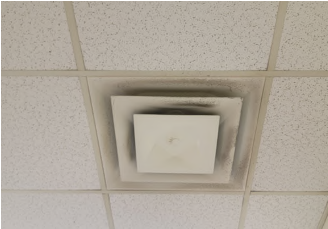
Photograph No. 4 Showing General Dust and Debris - Gym Hallway
