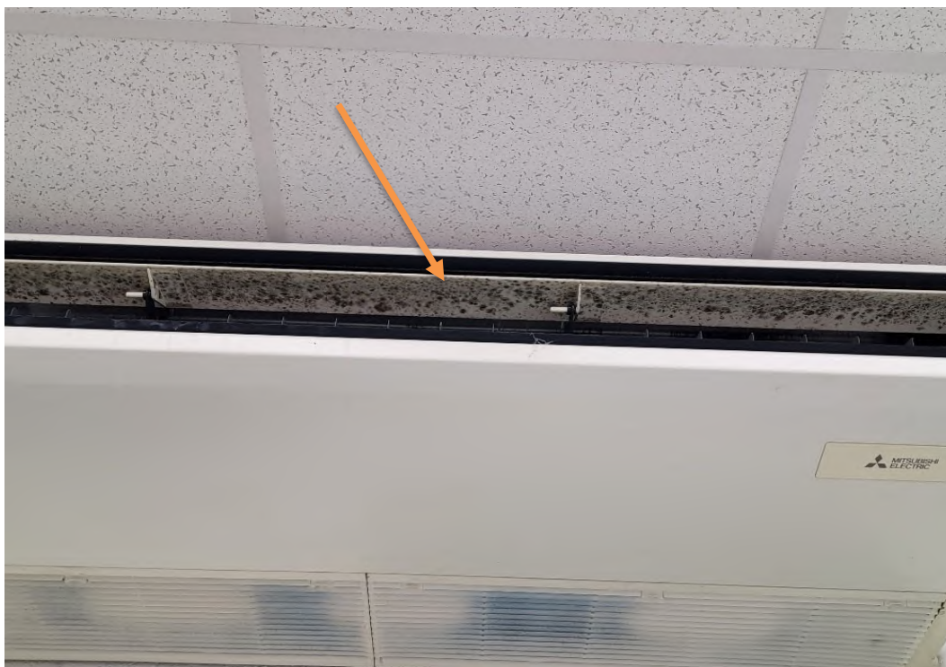
Photograph No. 5 Showing Visible Mold Growth on Ceiling Unit Vent - Classroom 104 Ceiling Unit Vent Not Sampled Due To Height
