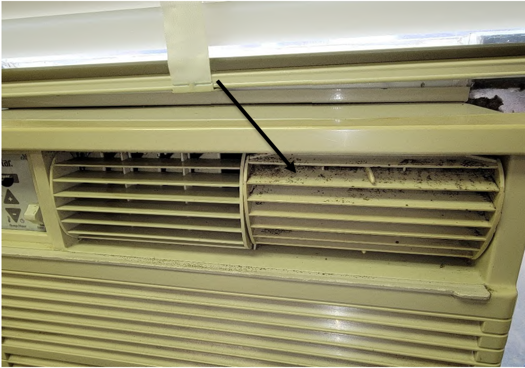
Photograph No. 1 Showing Visible Mold Growth - Office 101
