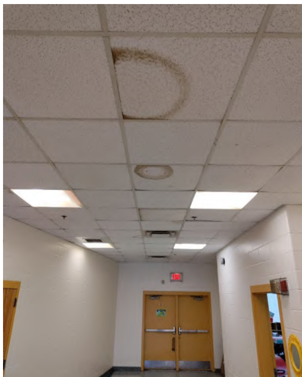
Photograph No. 6 Showing Multiple Stained Lay-In Ceiling Tiles - Gym Hallway
