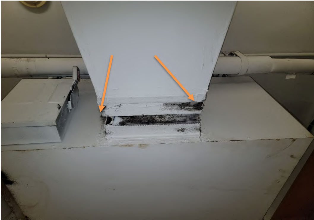
Photograph No. 3 Visible Mold Growth on Duct - Copy Room
