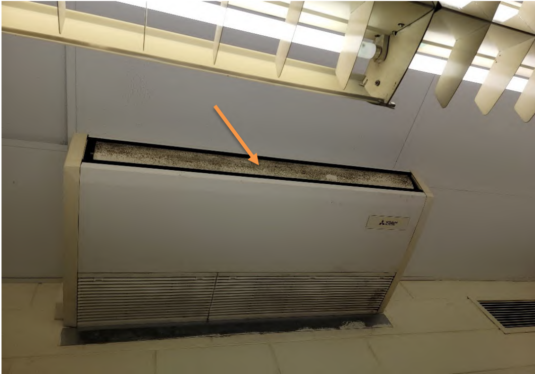
Photograph No. 1 Visible Mold Growth on Ceiling Unit - Classroom 11
