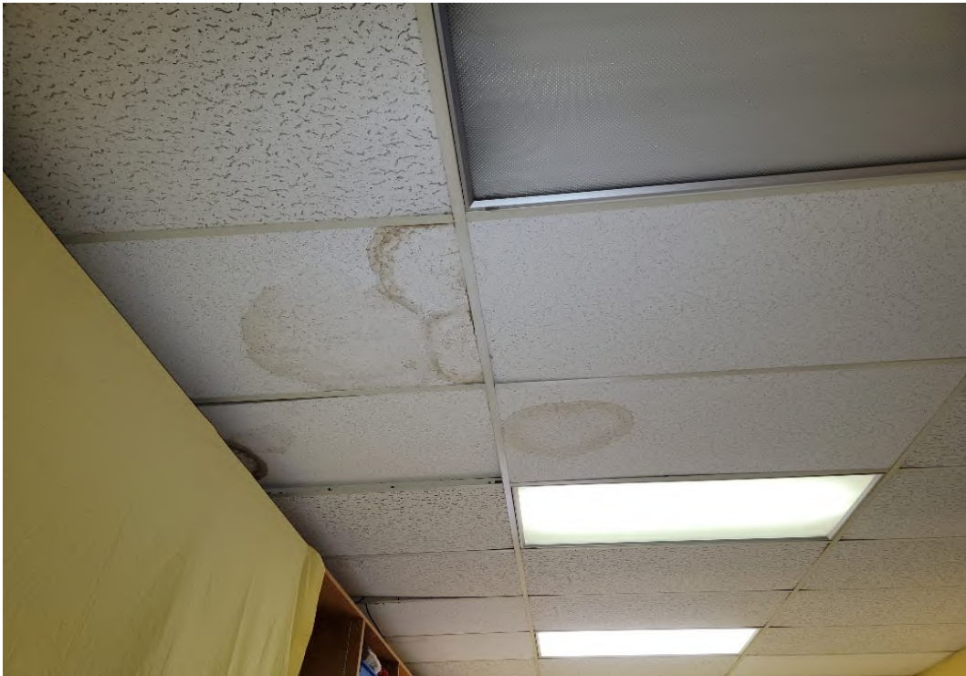
Photograph No. 4 Showing Multiple Stained Lay-In Ceiling Tile - Schools Psychologist
