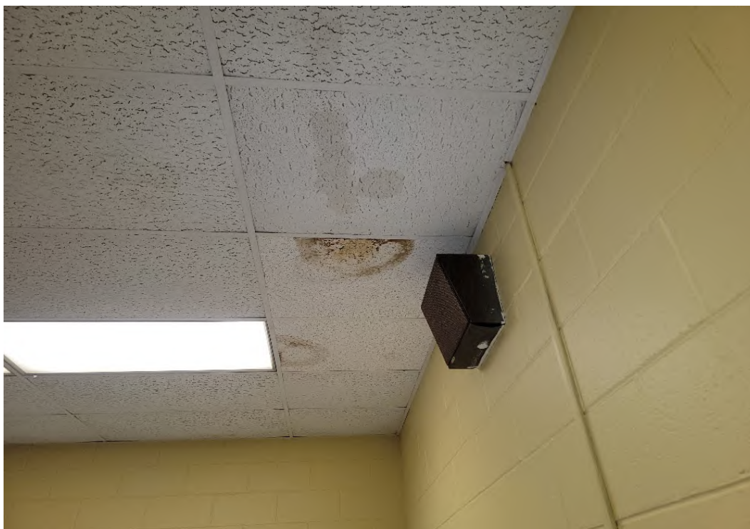
Photograph No. 5 Showing Multiple Stained Lay-In Ceiling Tile- Teachers Room Ceiling Not Sampled Due To Height
