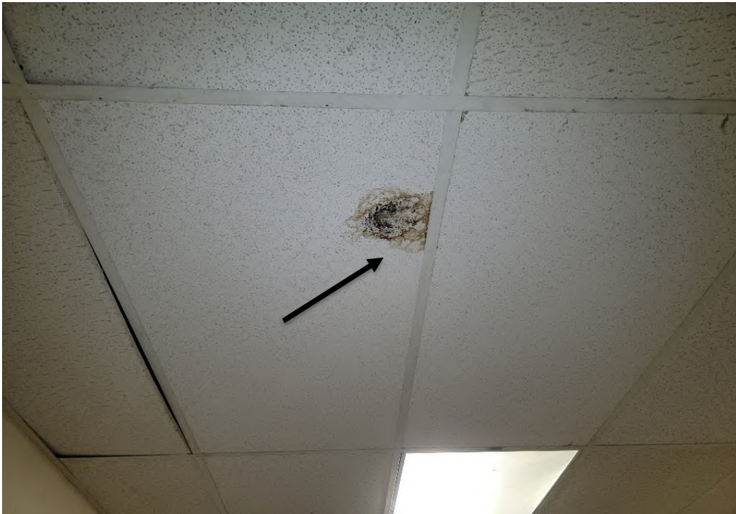
Photograph No. 2 Stachybotrys on Lay-In Ceiling Tile - Hallway
