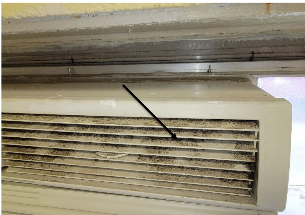
Photograph No. 6 Showing Visible Mold Growth Window AC Unit Vent
