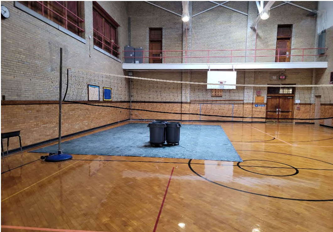
Photograph No. 8 Active Water Roof Leak - Gym
