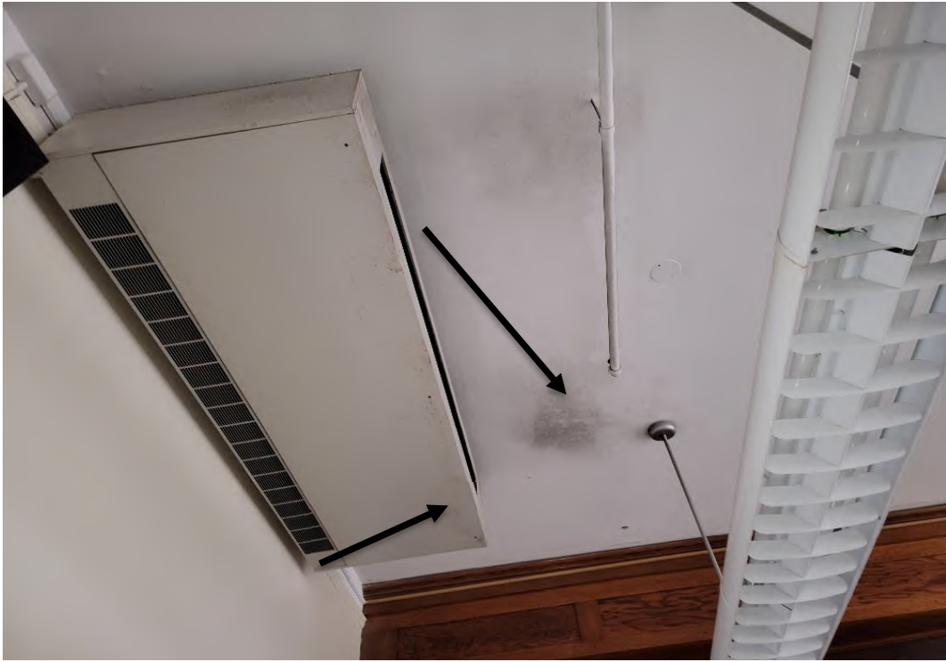
Photograph No. 7 Showing Visible Mold Growth on Unit and Ceiling - Classroom 204
