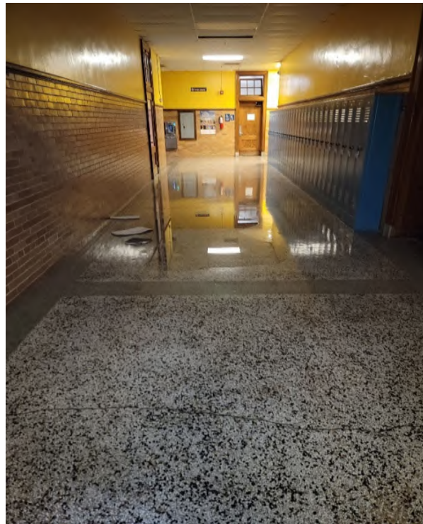
Photograph No. 10 Active Water Roof Leak - 2nd Floor Hallway
