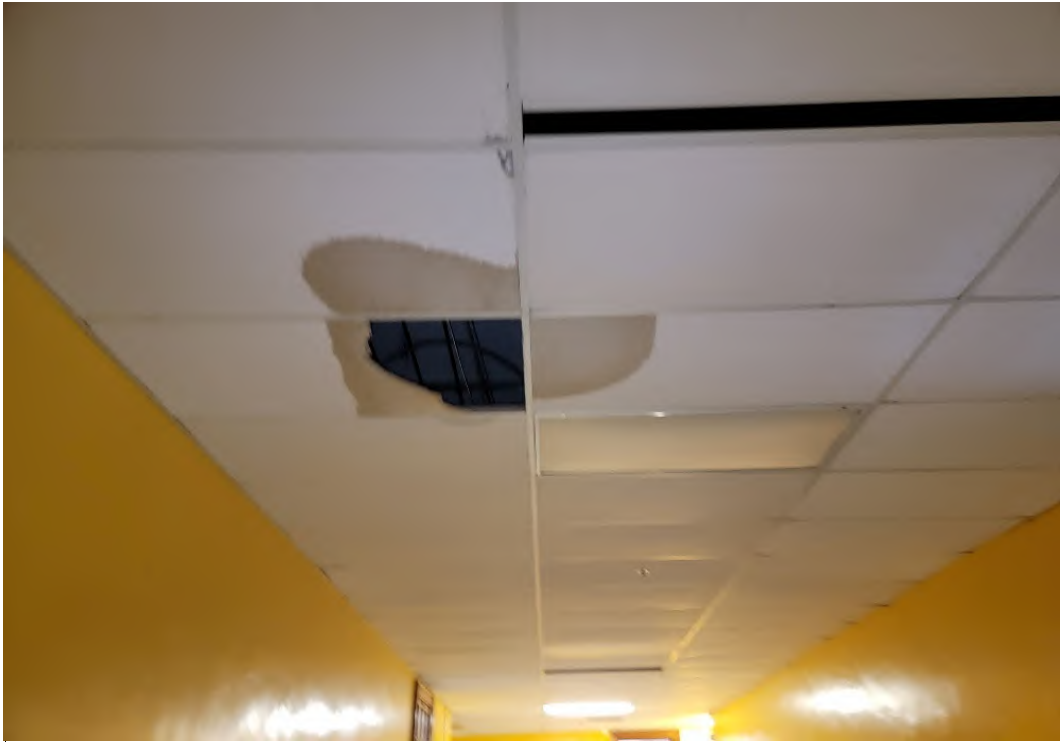
Photograph No. 11 Roof Leak - 2nd Floor Hall
