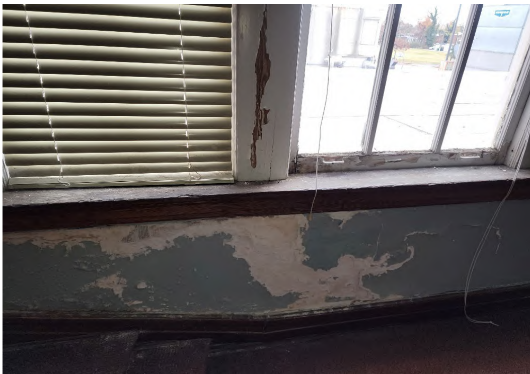
Photograph No. 5 Showing Wall Damage in Auditorium Ceiling Not Sampled Due To Height
