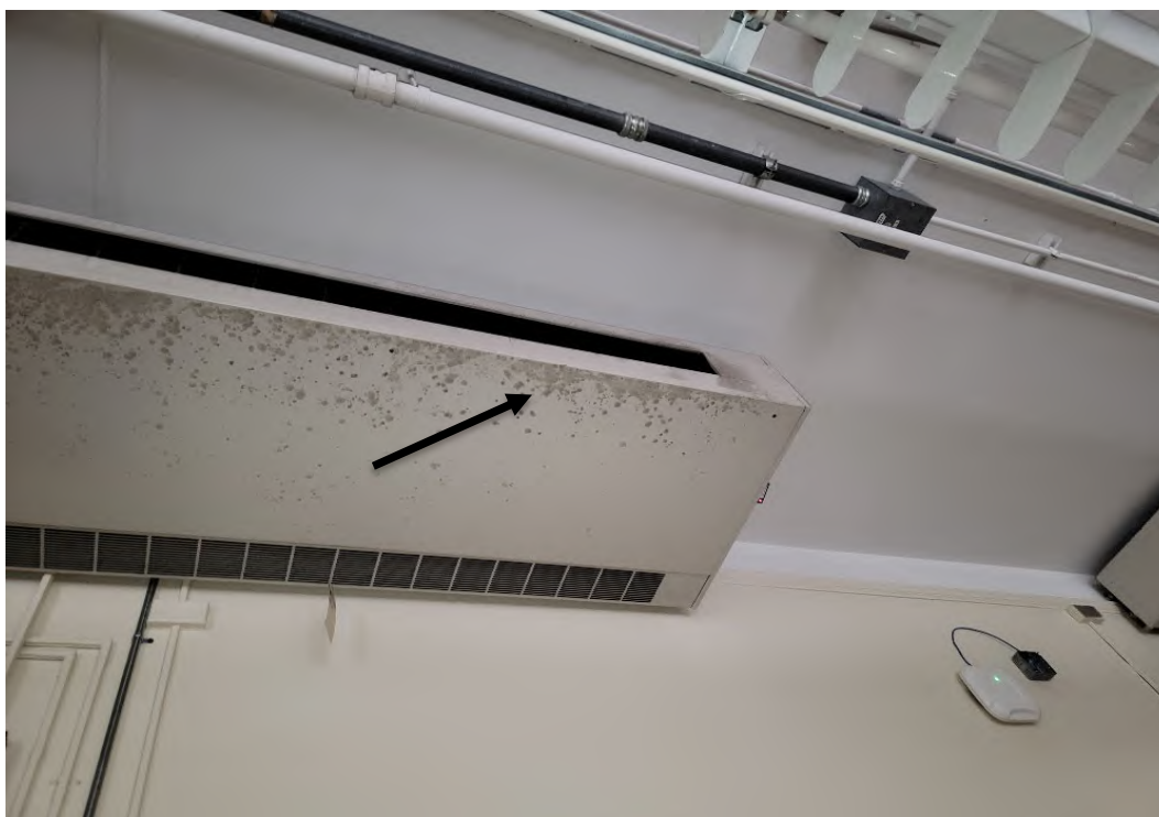
Photograph No. 6 Showing Visible Mold Growth in Classroom 208
