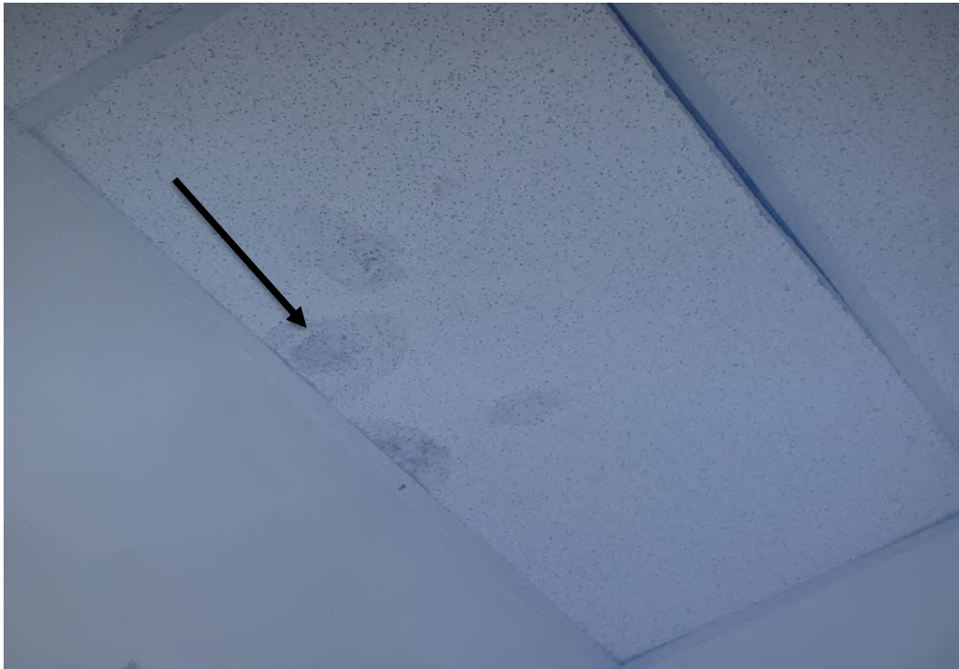
Photograph No. 16 Visible Stachybotrys Growth on Lay-In Ceiling Tile - Classroom 314
