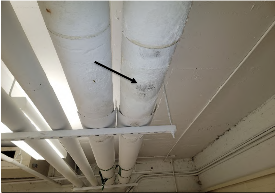
Photograph No. 15 Visible Mold Growth on Pipes - Classroom 115
