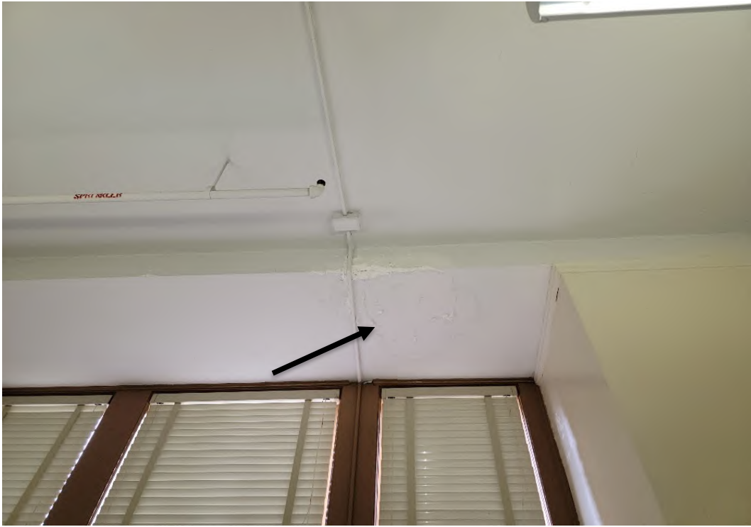
Photograph No. 3 Showing Ceiling Damage - Classroom 110A
