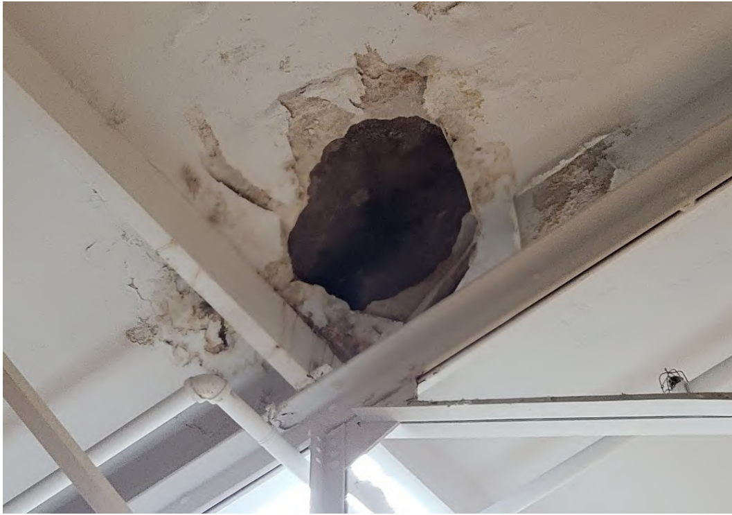
Photograph No. 9 Roof Leak - Gym
