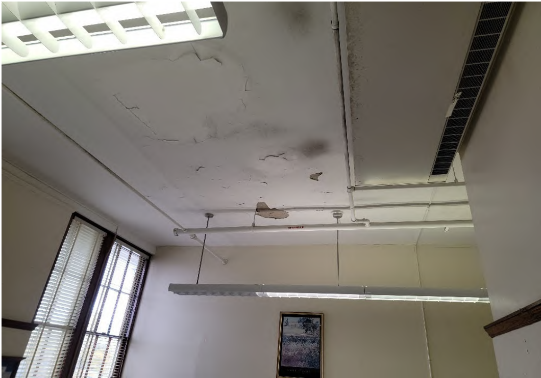
Photograph No. 12 Ceiling Damage - Classroom 306
