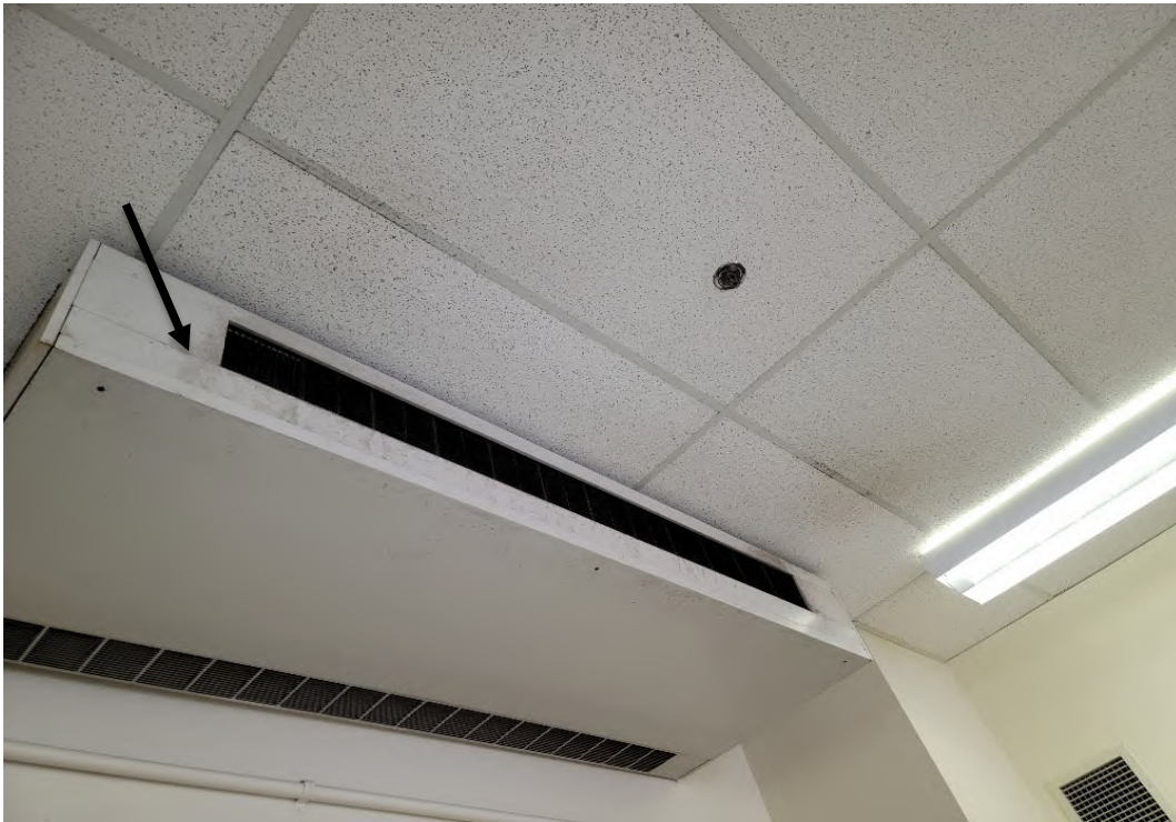
Photograph No. 4 Showing Visible Mold Growth - Classroom 209
