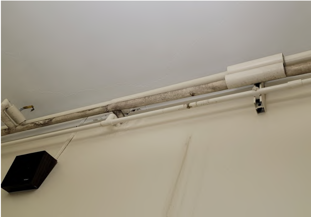
Photograph No. 17 Visible Mold Growth on Pipes - Classroom 310A
