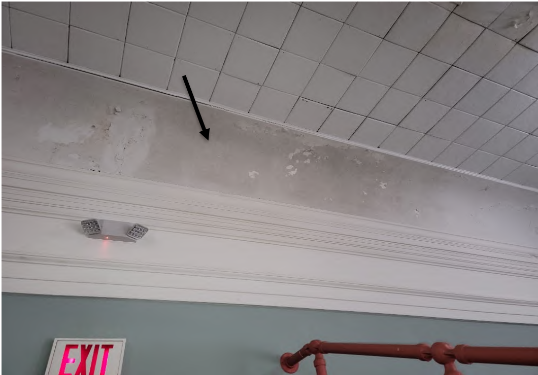
Photograph No. 18 Visible Mold Growth on Wall - Auditorium Balcony
