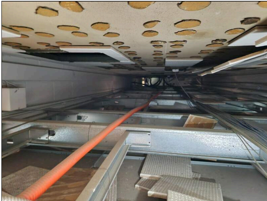
6 - Delaminating 1'x1' ceiling tiles above the main hallway
