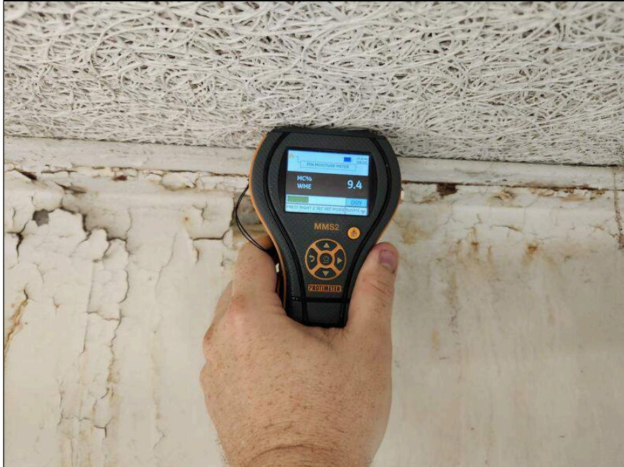
3 - Evidence of water intrusion on structural steel in B-106
