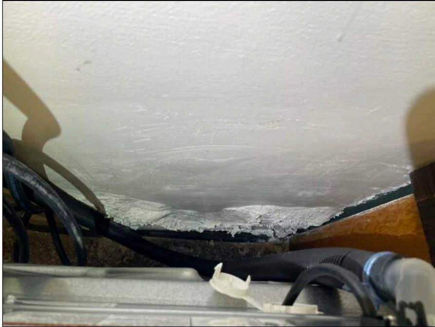
5 - Moisture damaged plaster wall behind the washing machines in Room A-8
