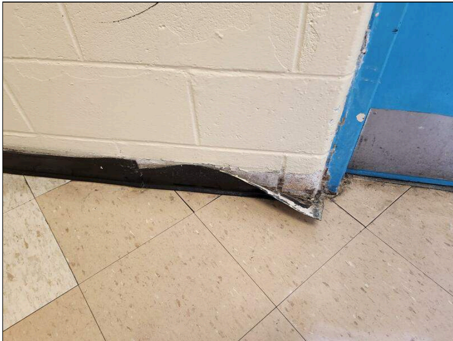
10 - Delaminating vinyl cove baseboard in the connector hallway
