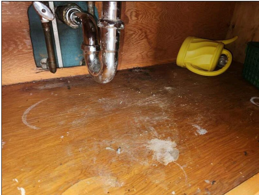
4 - Moisture and mold impacted sink cabinet in Room A-5
