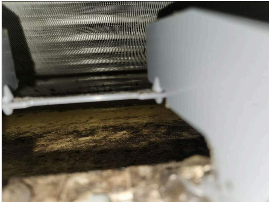
12 - Mold observed within the PTAC unit in Room 116
