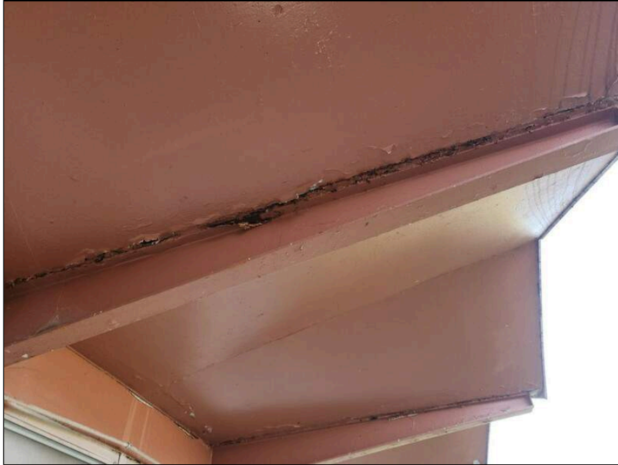
1 - Damaged roof support beam and soffit at B-Pod
