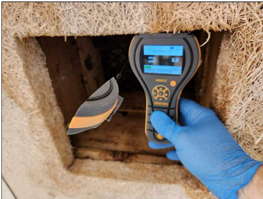
2 - Moisture stained tectum ceiling in B-106 Storage Room
