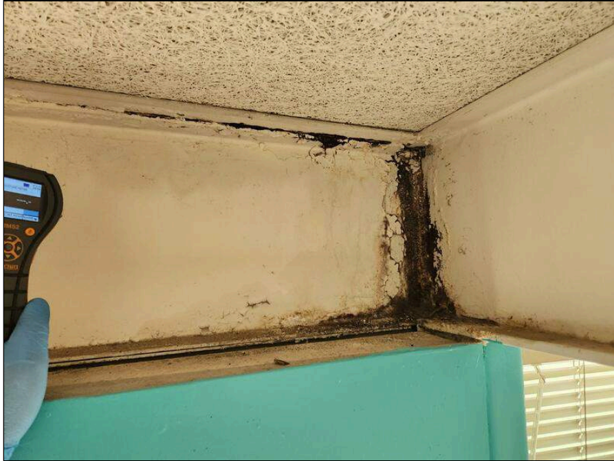
1 - Evidence of water intrusion and suspect mold on structural steel in B-105
