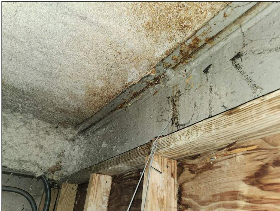
2 - Moisture impacted tectum ceiling and steel beam above the ceiling in the A-Pod connector Hall
