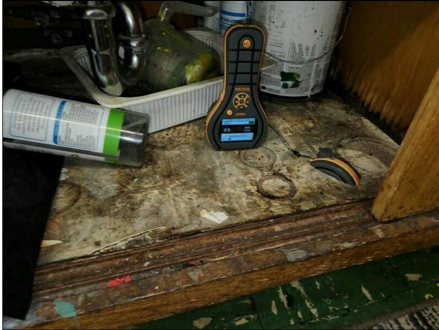
9 - Mold impacted sink cabinet in Room 102
