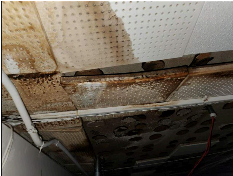
10 - Moisture damaged plaster ceiling in the main hallway
