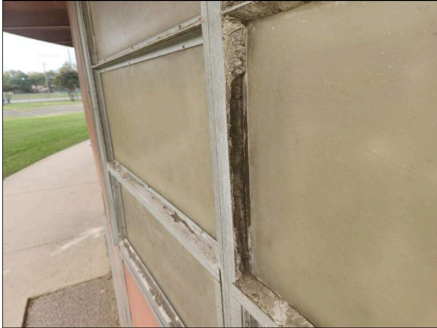
5 - Failing window sash glazing on the A-Pod
