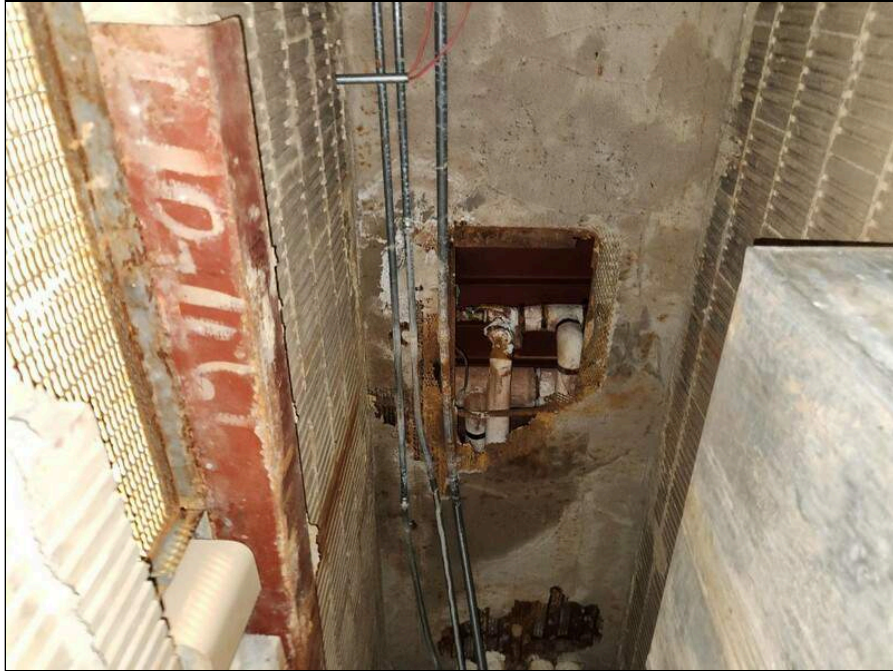
3 - Moisture damaged plaster ceiling within the hall bathroom - wet wall chase
