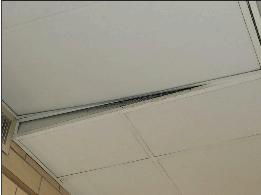
15 - Mold impacted ceiling tiles in the kitchen adjacent to an HVAC supply
