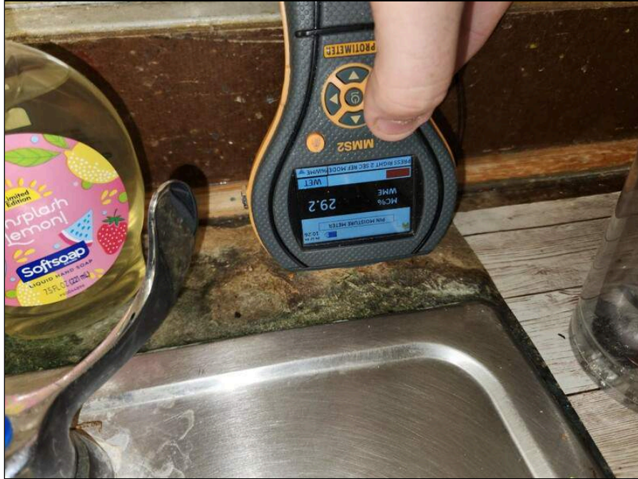
11 - Elevated moisture meter reading on the top of the sink in Room 119
