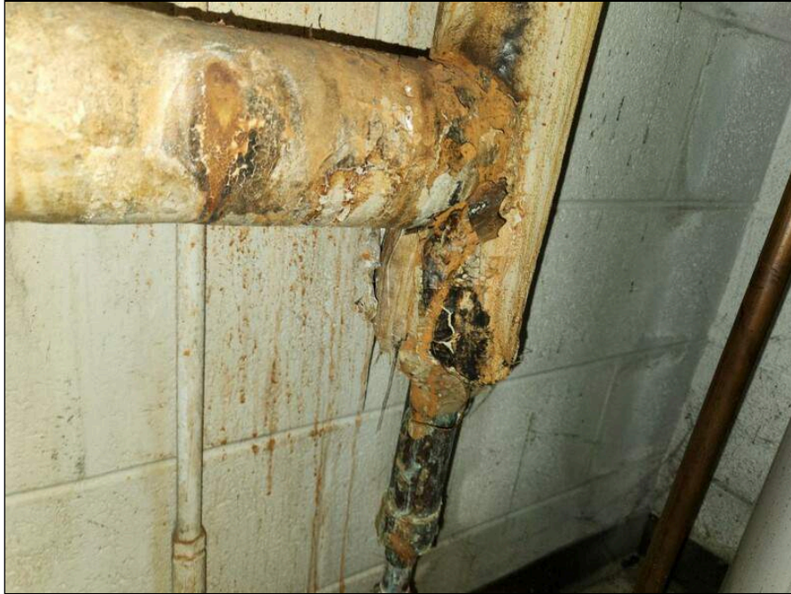
7 - Mold impacted pipe insulation in the HVAC Room
