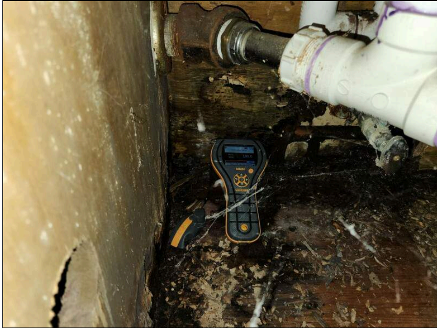
1 - Mold and evidence of an active water leak in the sink cabinet in Room 107
