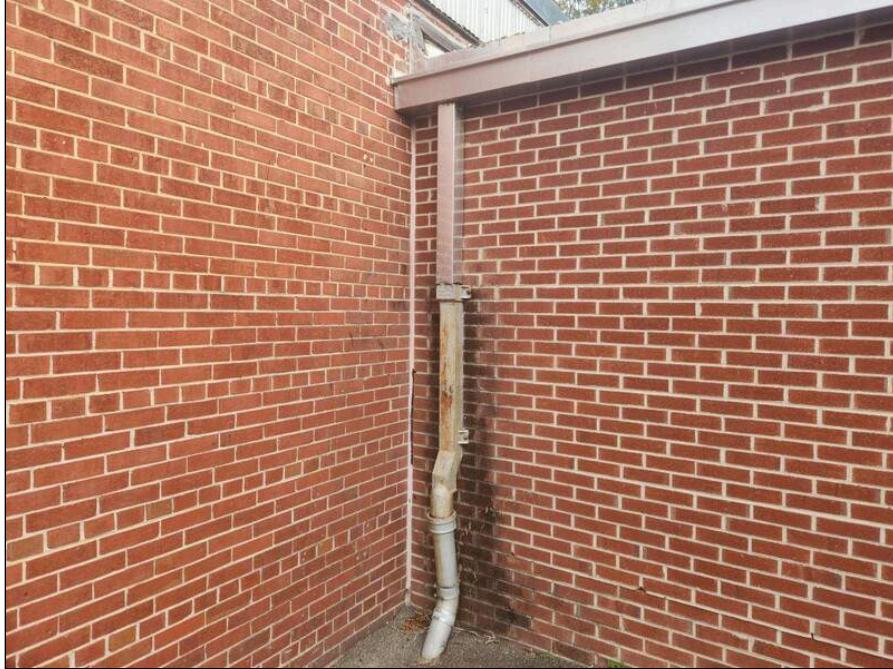
7 - Staining on the exterior brick outside the A-Pod connector
