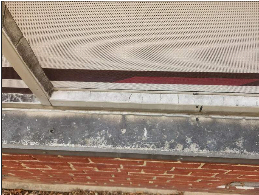
4 - Failing window sash glazing on the main building
