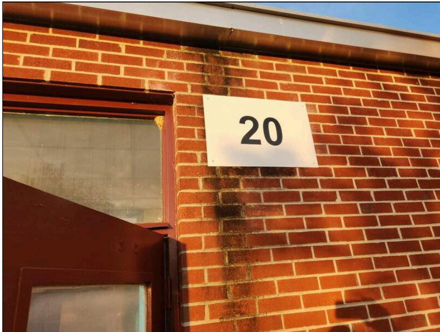
2 - Staining on the exterior brick outside the B-Pod connector hall
