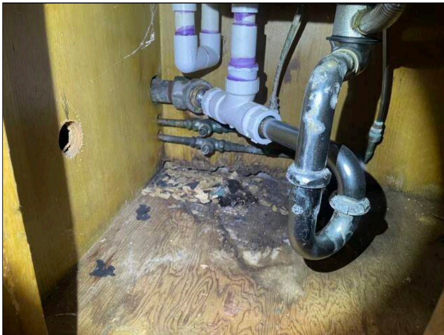
2 - Mold and moisture damaged sink cabinet in Room 109
