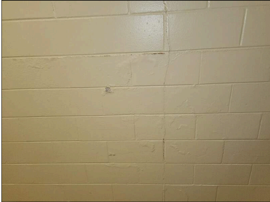
9 - Bubbling CMU block wall paint in the connector hall
