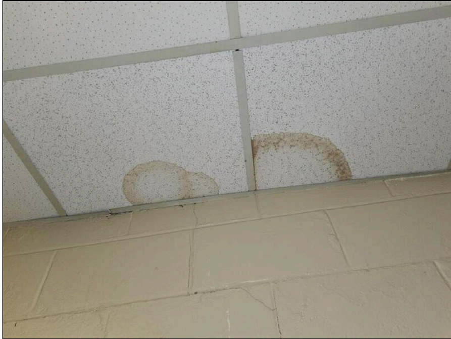
5 - Moisture stained ceiling tiles in the connector hall
