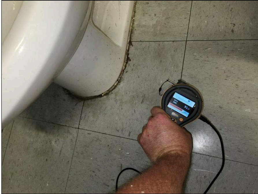
5 - Elevated moisture associated with the flooring around the toilet in the Clinic
