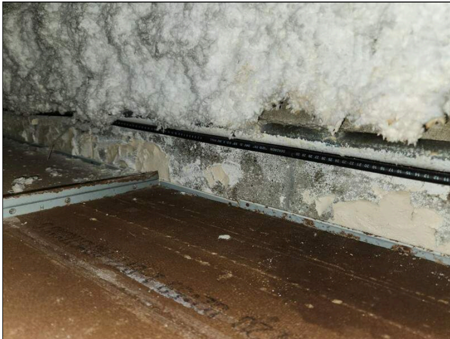
8 - Evidence of water intrusion of the CMU block wall above the ceiling in the connector hall
