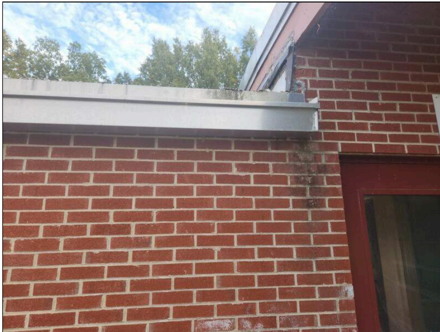
6 - Staining on the exterior brick outside the A-Pod connector
