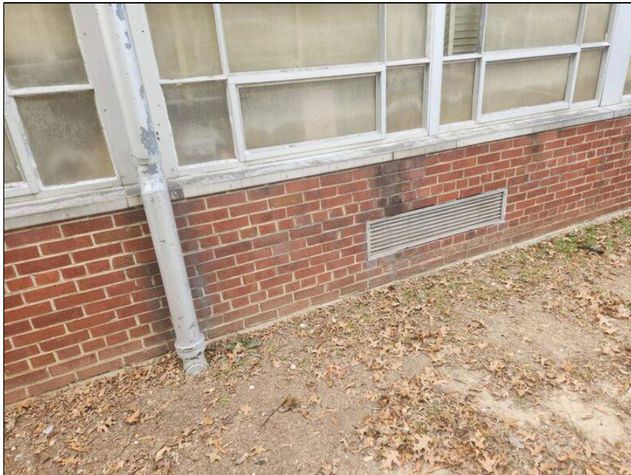
8 - Staining on the exterior brick outside room 102
