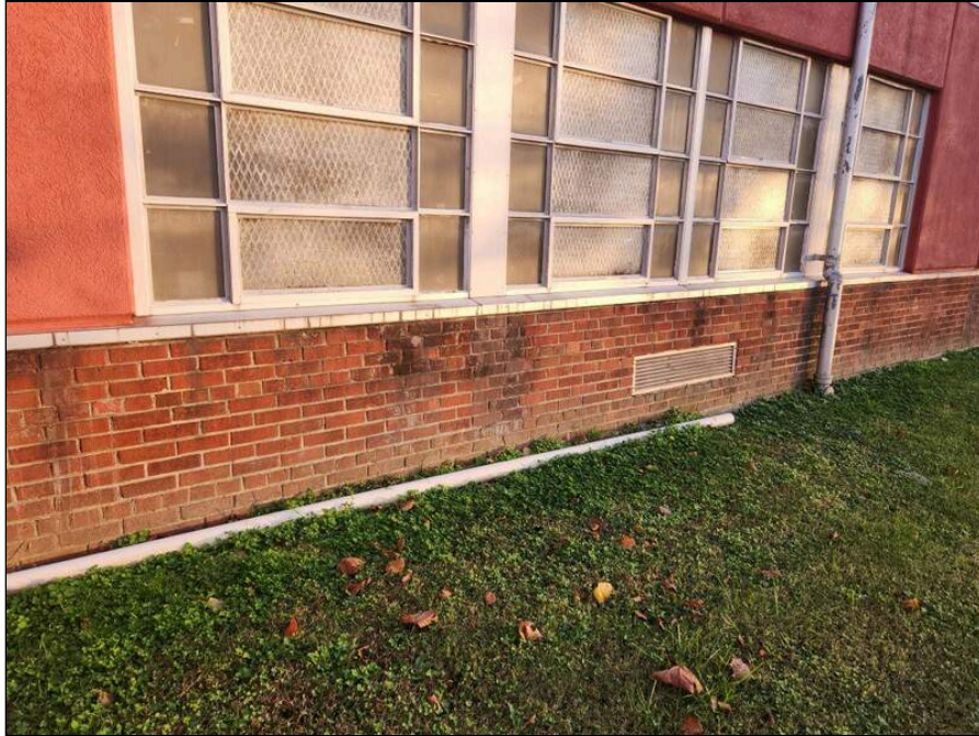
3 - Staining on the exterior brick outside Room 109
