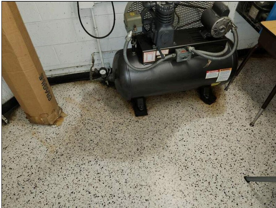
6 - Staining on floor associated with the compressor in the HVAC room
