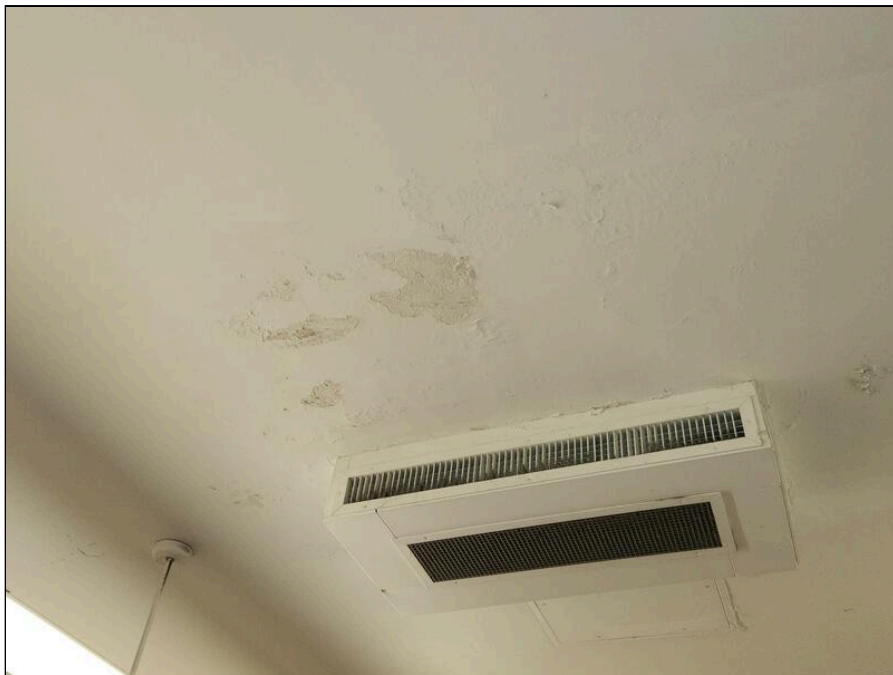
14 - Moisture and Mold impacted plaster ceiling and mold impacted ceiling PTAC unit in Room 113
