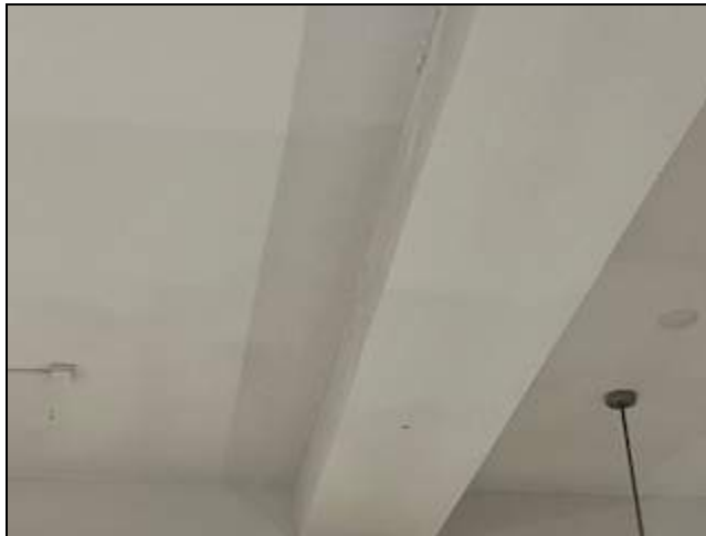
10 - View of damaged plaster bulk head in room 220 - possibly from pipe leaks.
