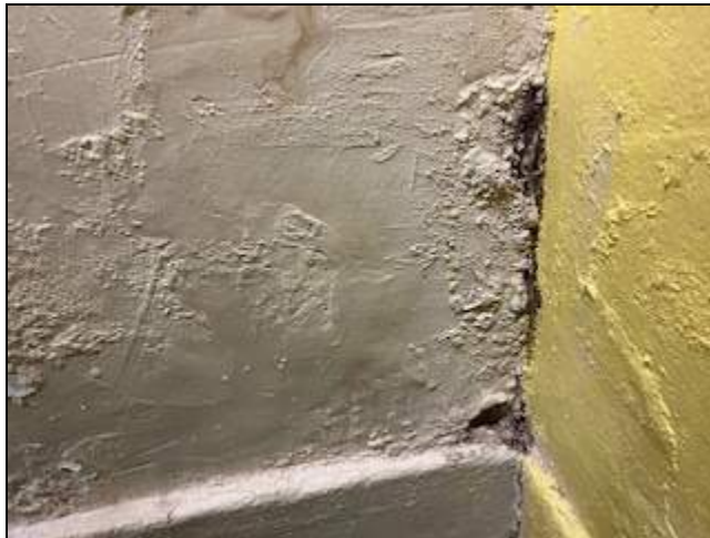
12 - View of damaged plaster in room B8 with visible mold observed.
