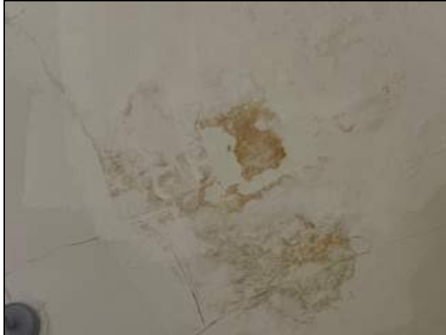
3 - Room 218 with water stained ceiling plaster; suspect mold observed.
