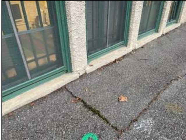
15 - View of exterior asphalt outside the basement room. ECS is unsure if this is outside room B8 where we observed active water intrusion and damaged plaster.
