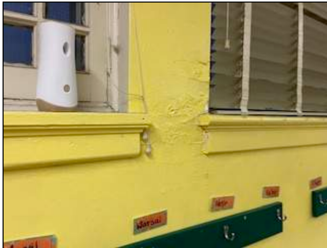
14 - View of water damaged plaster wall between the windows of room B7.
