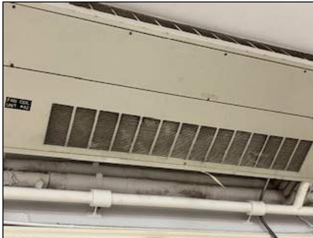
2 - General view of a ceiling mounted fan coil unit with heavy dust and suspect mold on vents.
