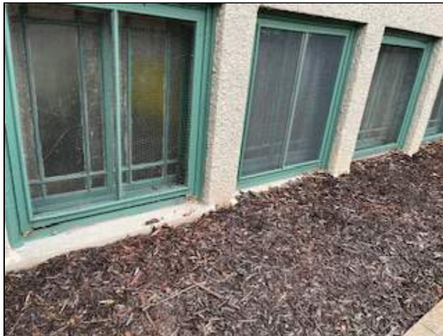
16 - View of mulch outside the basement room. ECS believes this may contribute to water intrusion if exterior water proofing is failing.
