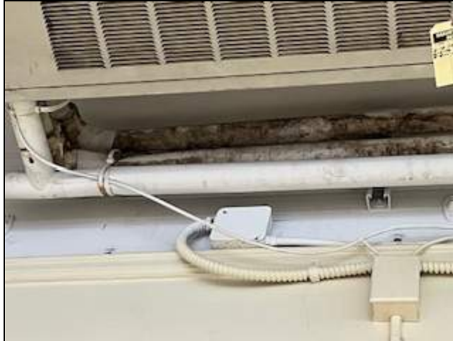
1 - General view of pipe with mold associated with a ceiling mounted fan coil unit.
