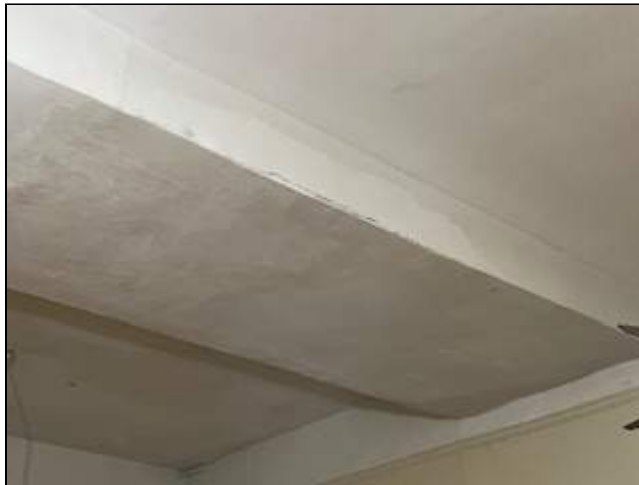
8 - View of the bulk head in the teachers lounge where it appears damage to the plaster has occurred from a possible pipe leak.
