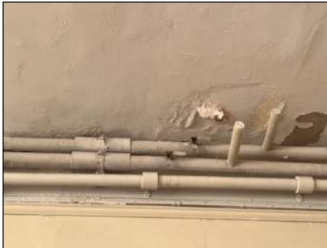
6 - View of room 211 ceiling showing water damage. ECS also observed a portion of the plaster on the floor below ceiling plaster.
