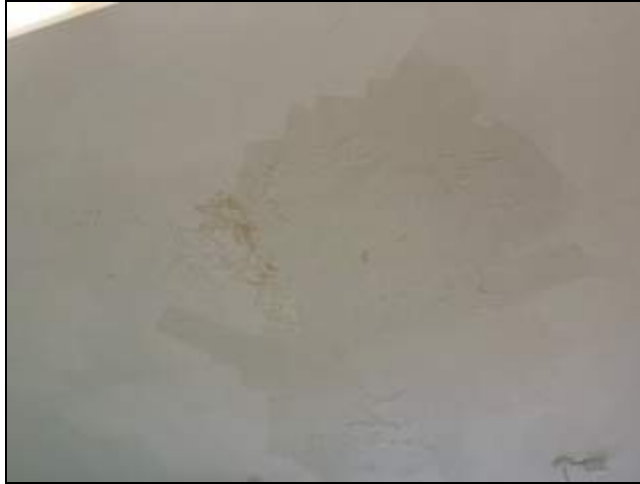
5 - View of room 217 ceiling with damaged plaster and water staining.
