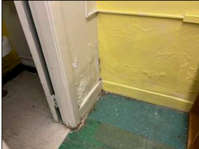
11 - View of damaged plaster in room B8 possibly from water intrusion from the exterior.
