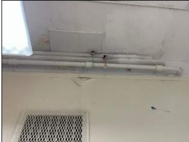
9 - View of room 222 with water damaged and stained ceiling plaster.
