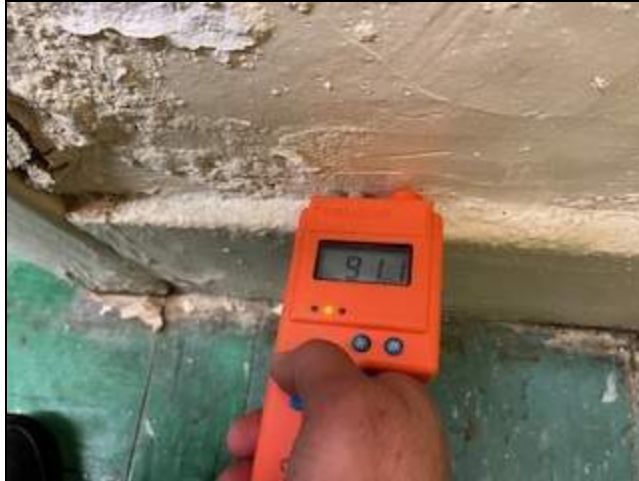
13 - View of moisture reading of the plaster wall in B8 showing elevated moisture levels.
