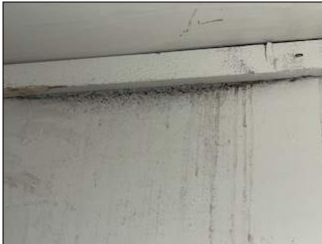
4 - View of plaster wall in the closet of room 218 with visible mold.
