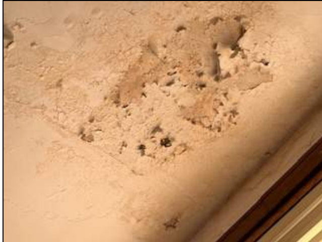
7 - View of room 211 ceiling showing water damage. ECS also observed a portion of the plaster on the floor below the damaged plaster.
