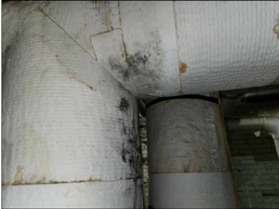
47 - Mold on pipe insulation in the boiler room
