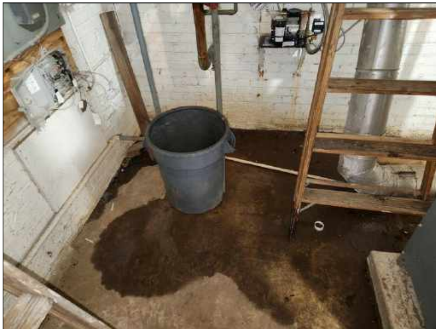
44 - Leaking pipe causing standing water on the floor of the boiler room
