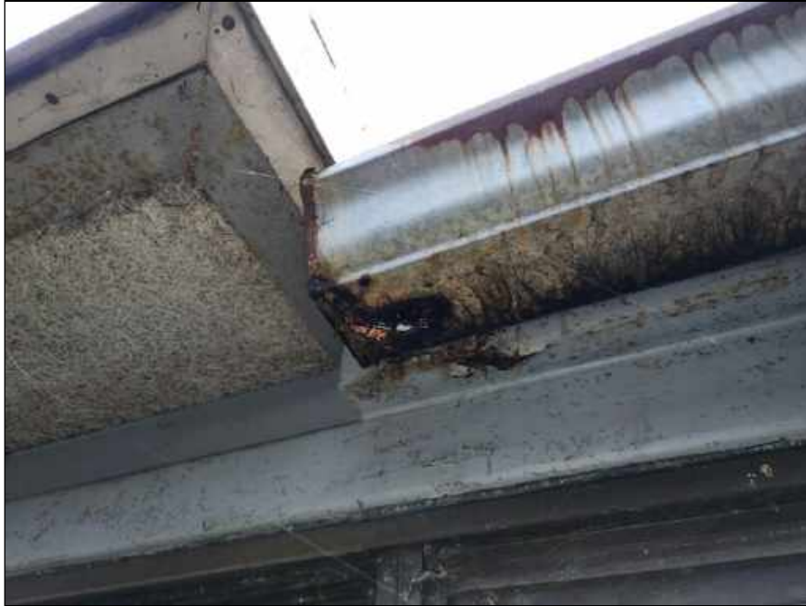
5 - Damaged gutter causing moisture intrusion on the tectum ceiling in the connector hallway
