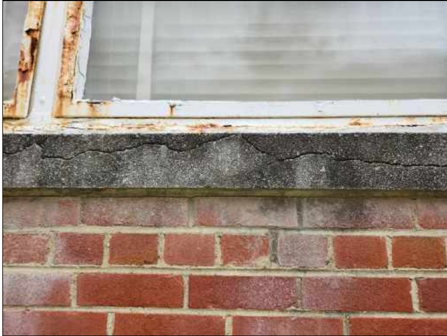
3 - Damaged window ledge at an Auditorium window
