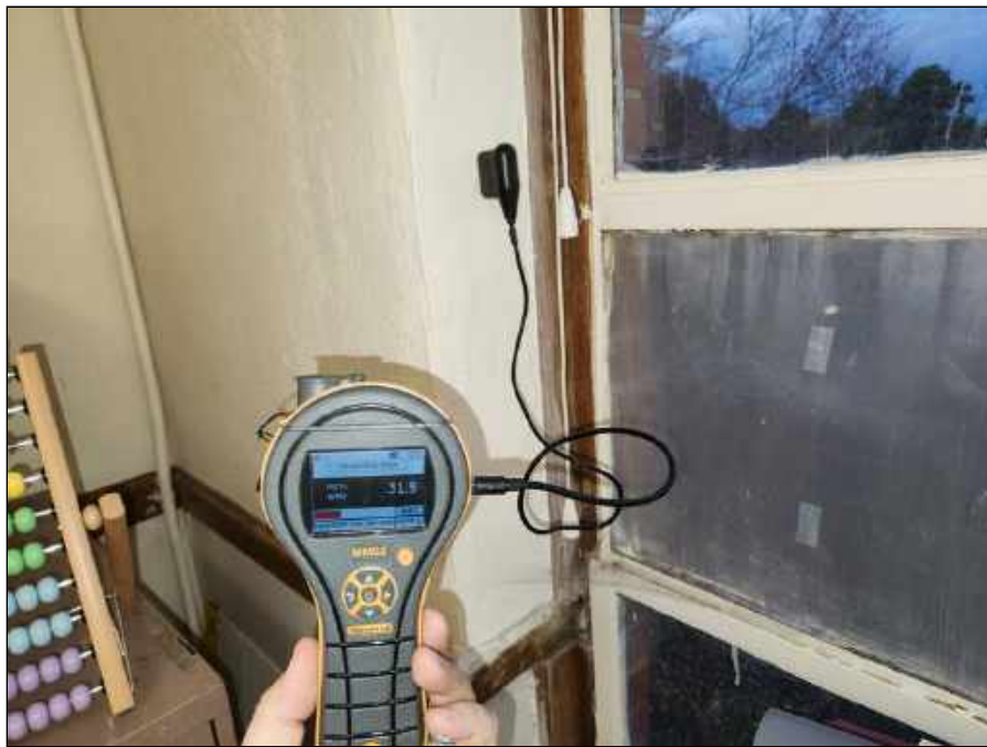
36 - Elevated moisture meter reading collected from the wall in Room 217
