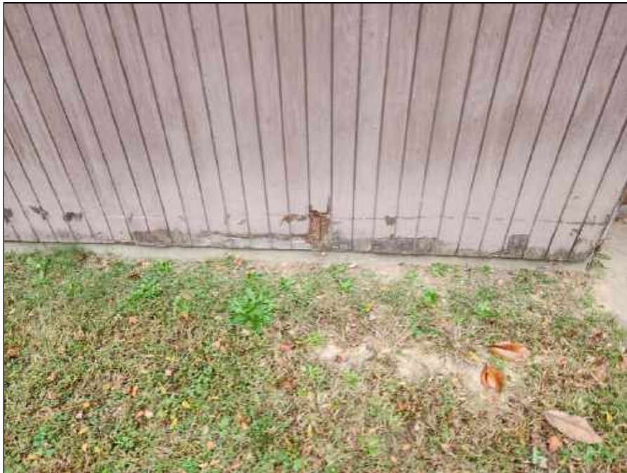
6 - Damaged exterior wood wall panels
