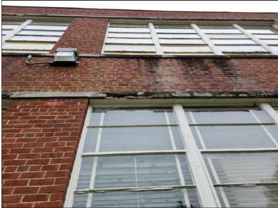
11 - Damaged window ledges on the North side of the building
