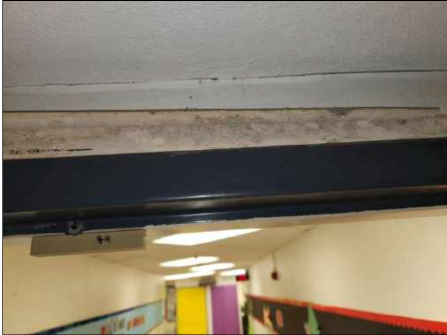
1 - Mold impacted drywall at the entrance to the pod classrooms
