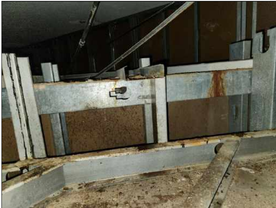
20 - Mold and moisture impacted drywall and framing above the Library hallway
