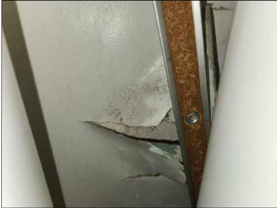
3 - Mold and moisture impacted plaster wall behind piping in Room 101
