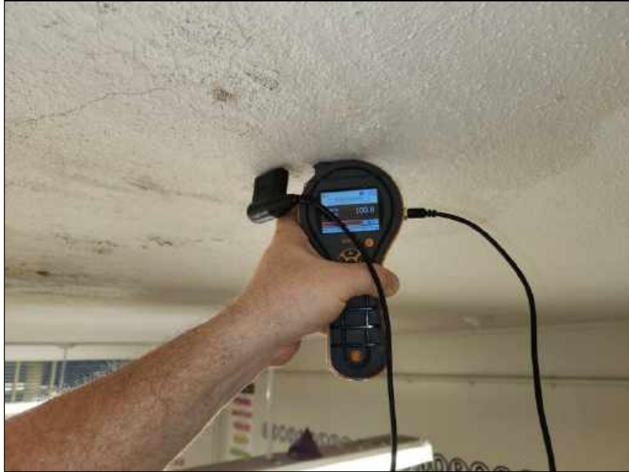
35 - Elevated moisture meter reading indicating that the plaster ceiling is saturated and an active moisture source may be present above the ceiling in Room 218
