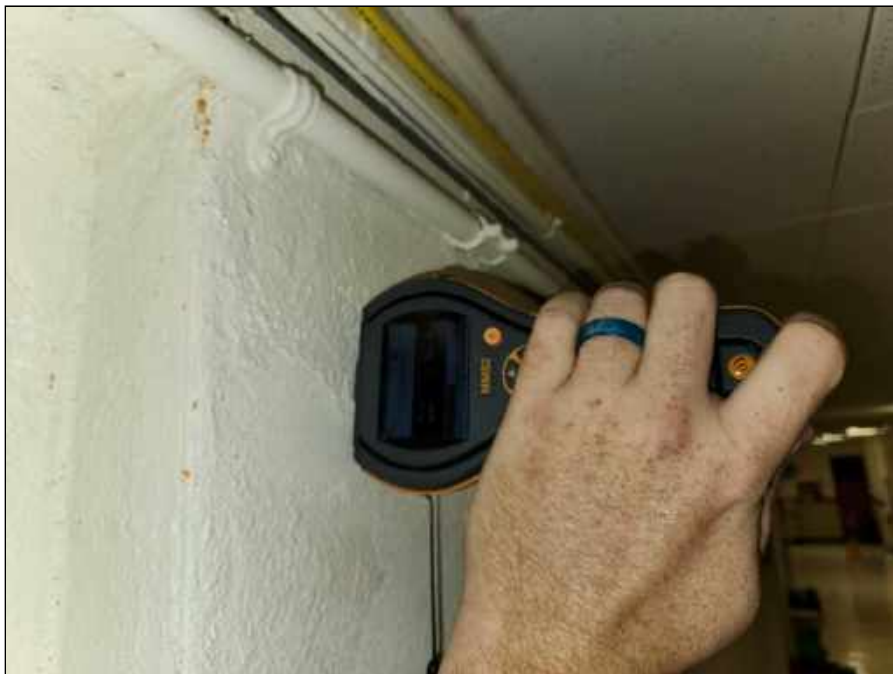
38 - Elevated moisture meter reading collected from a plaster wall in the hallway across from Room 110
