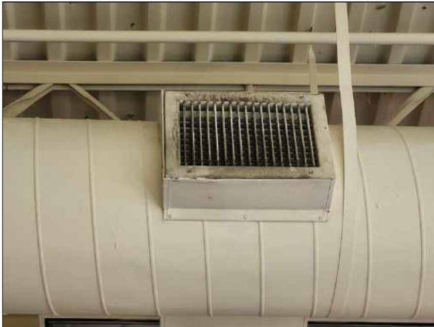
24 - Mold observed on the HVAC supply vents on the main trunk in the library
