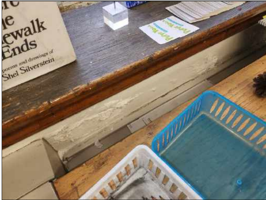
11 - Moisture damaged plaster wall in Room 108
