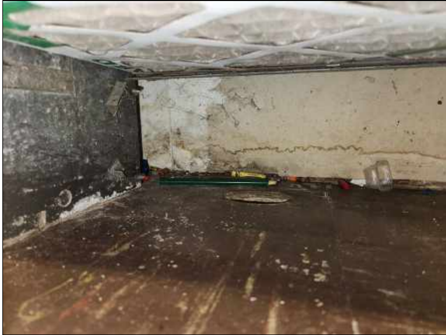
5 - Suspect mold on the plaster wall beneath the fan coil
