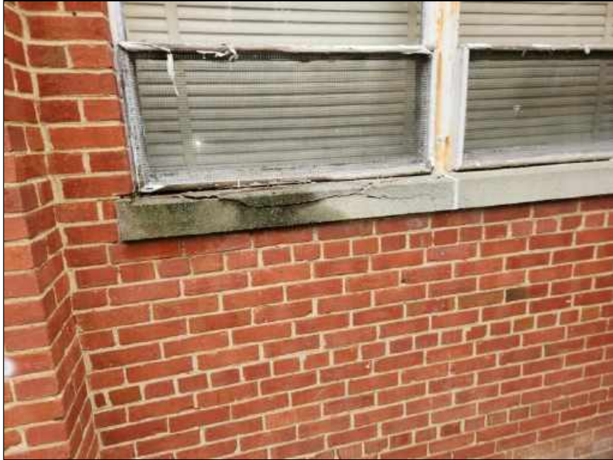
5 - Damaged window ledge at a Cafeteria window
