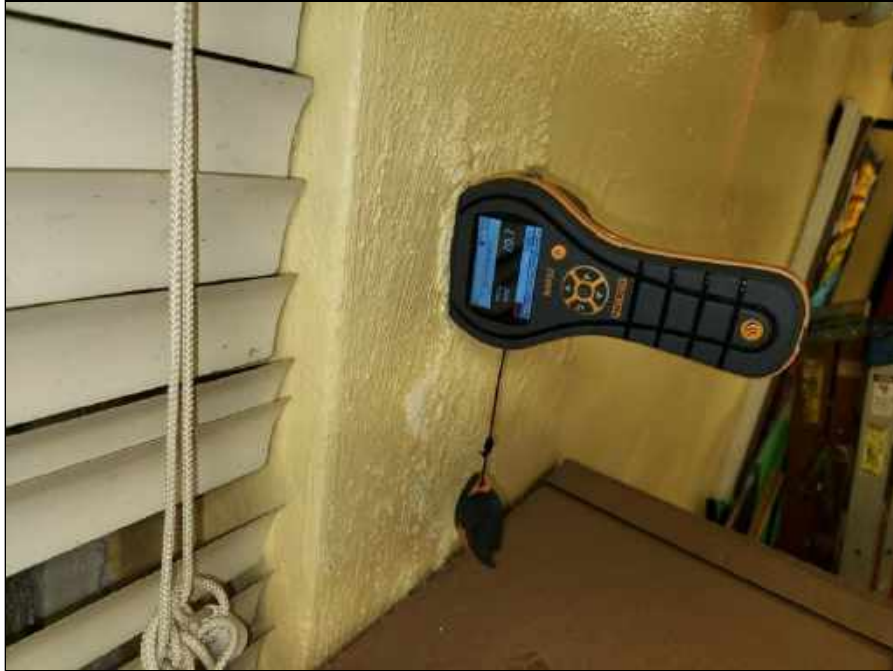
27 - Elevated moisture meter reading collected from a plaster wall in the cafeteria
