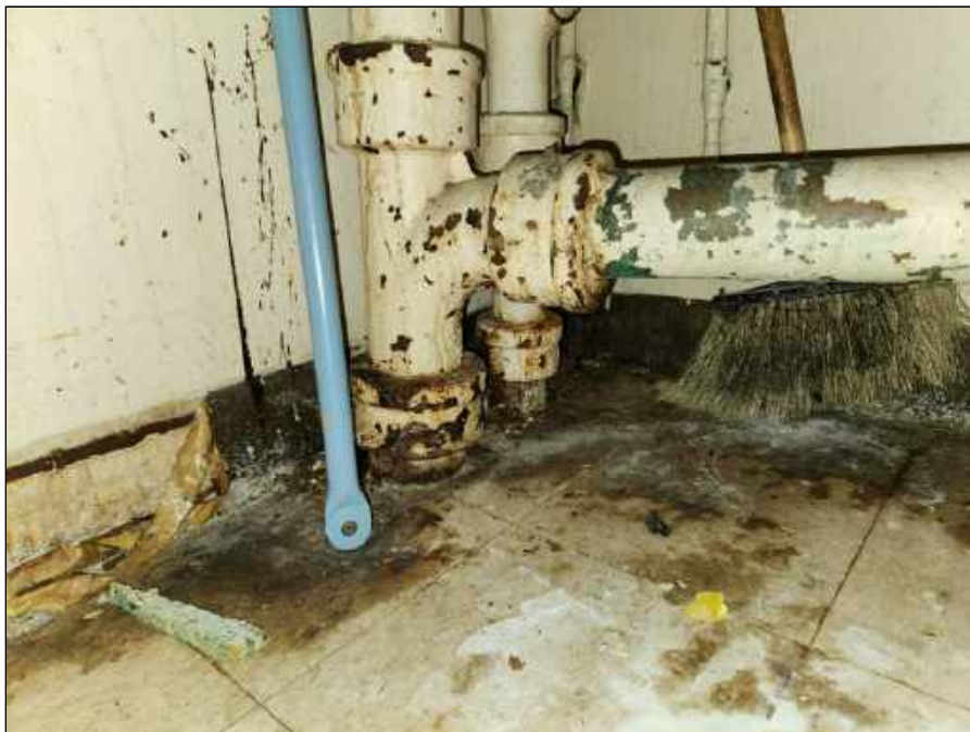
4 - Mold on floor tiles and the base of the plaster wall in the janitor's closet
