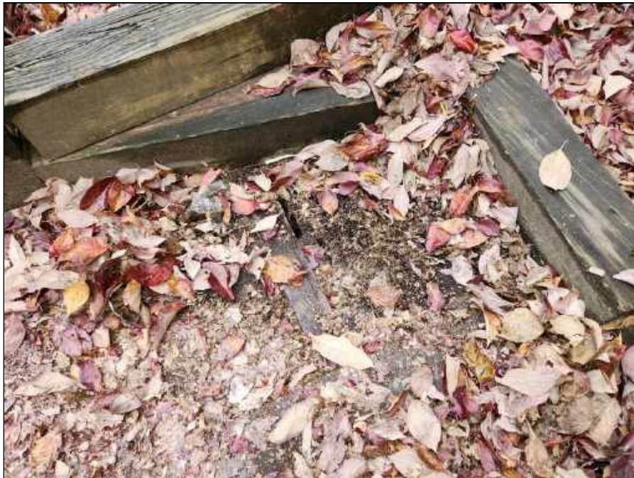
8 - Clogged storm water drain in the courtyard
