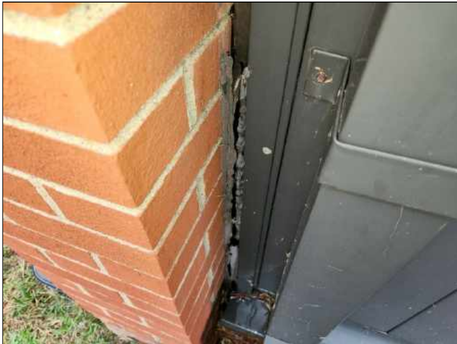
4 - Damaged sealants associated with the exterior metal wall panels outside Room 126
