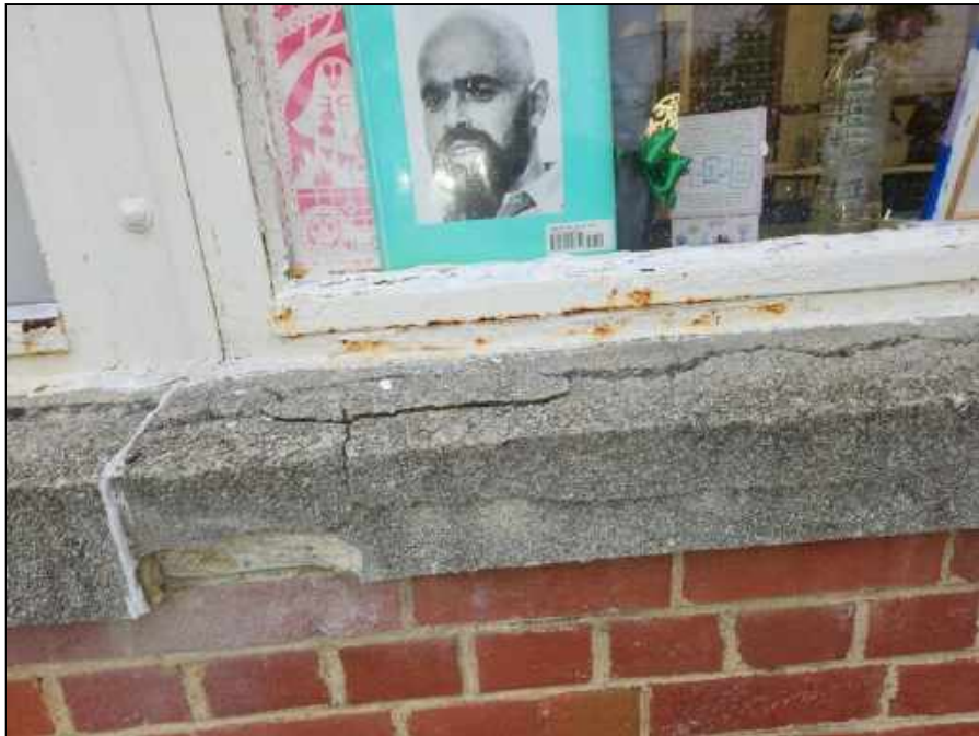
10 - Damaged window ledge on the East side of the building
