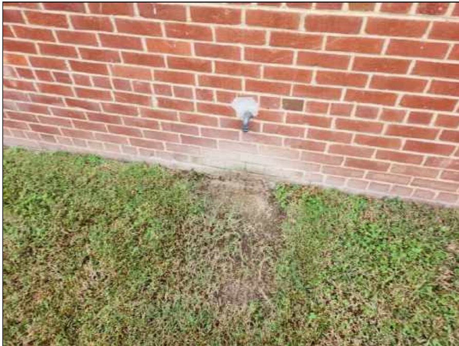
12 - Drain on the East side of the building draining against the foundation
