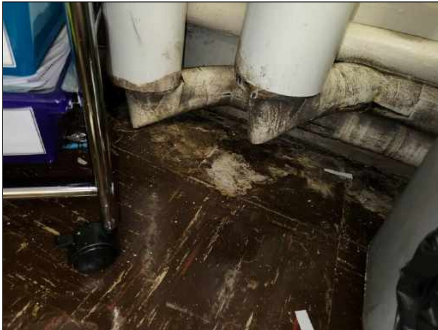
10 - Mold on pipe insulation in Room 102
