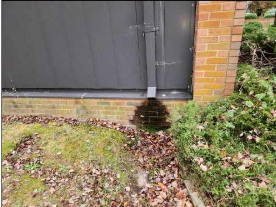
13 - Downspout draining against the foundation outside the main office
