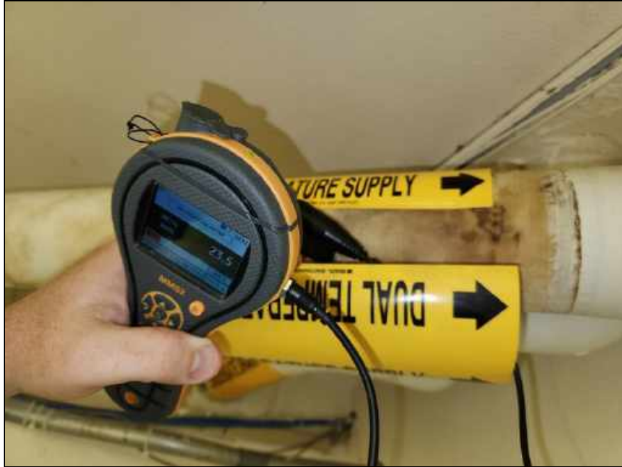
17 - Mold and moisture impacted pipe insulation in the room beside Room 111
