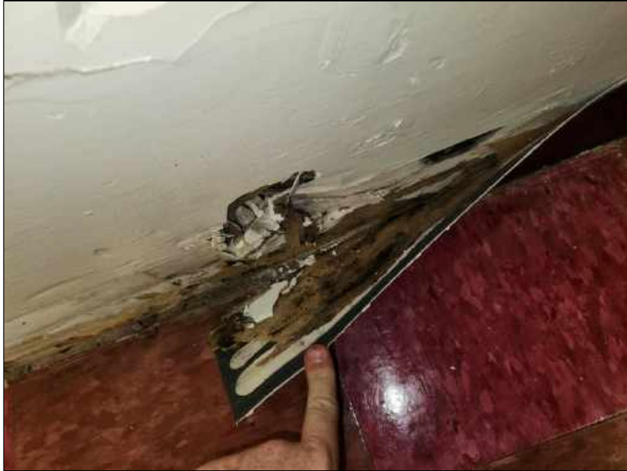
49 - Mold and moisture impacted drywall in Room 126 - the Music Room
