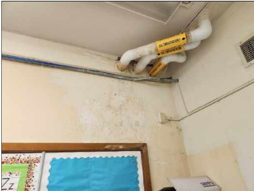
16 - Moisture damaged plaster wall observed in room beside Room 111 on 10-18-23
