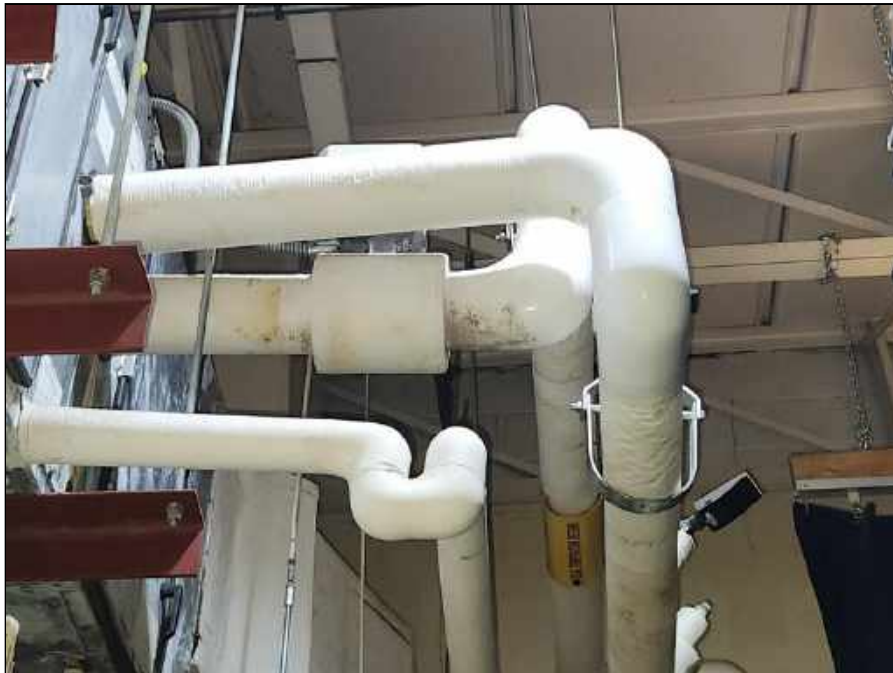
42 - Mold on pipe insulation by stage (right)
