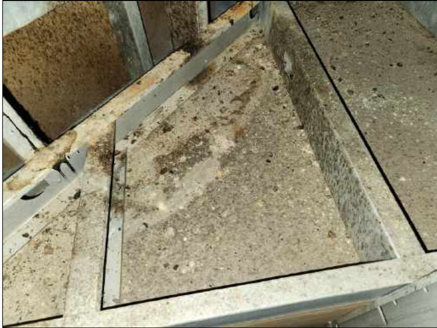
19 - Mold and moisture impacted drywall and framing above the Library hallway
