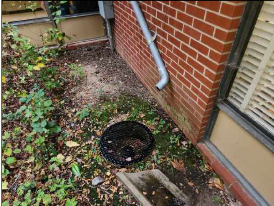
1 - A downspout draining against the foundation
