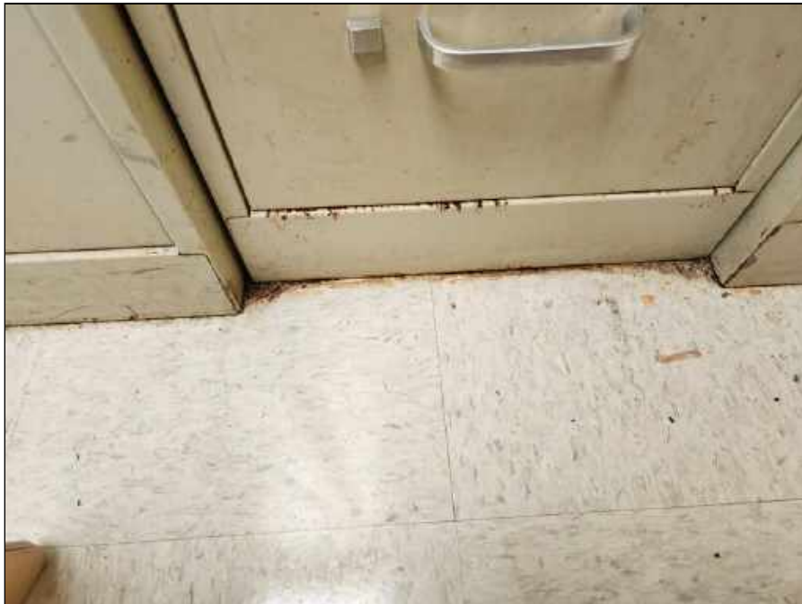
32 - Mold on the floor and rust at the base of a file cabinet in the Nurse's office
