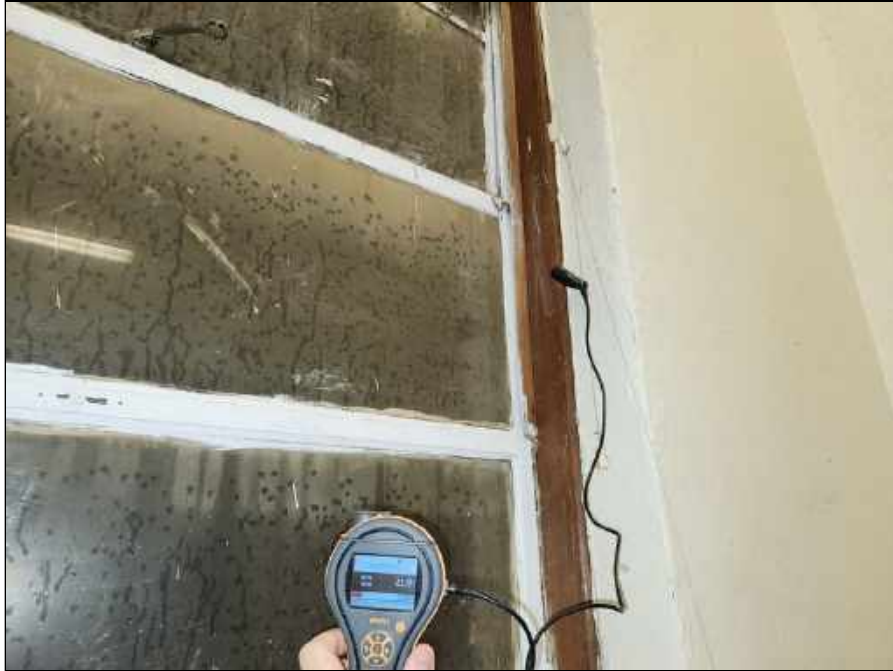
37 - Elevated moisture meter reading collected from the plaster wall in the stairwell by Room 110
