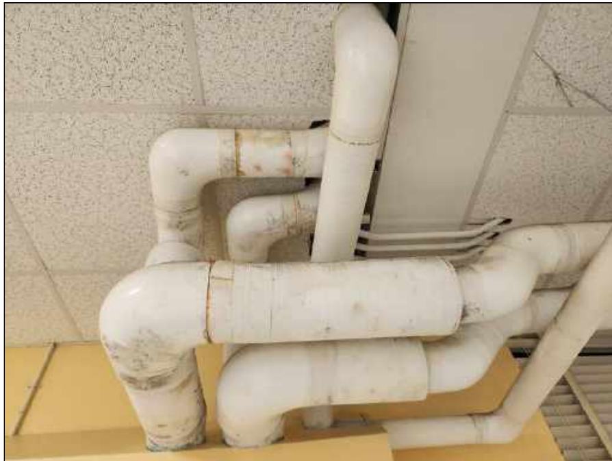
26 - Moisture and mold impacted pipe insulation in the cafeteria
