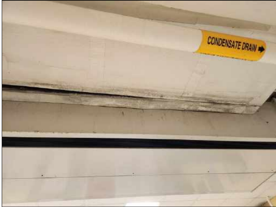
25 - Mold on HVAC duct board in the cafeteria
