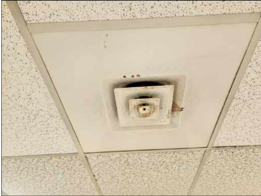
31 - Rusting on HVAC supply diffuser in the Nurse's office
