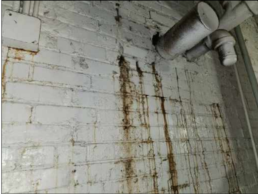
45 - Water leaking from holes in the back wall of the boiler room
