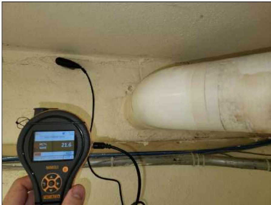
18 - Elevated moisture meter reading collected from the plaster wall around piping in the room beside Room 111
