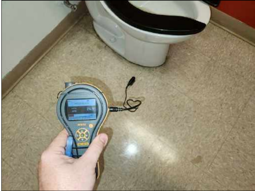
29 - Elevated moisture reading indicating elevated moisture beneath the flooring in the Nurse's bathroom
