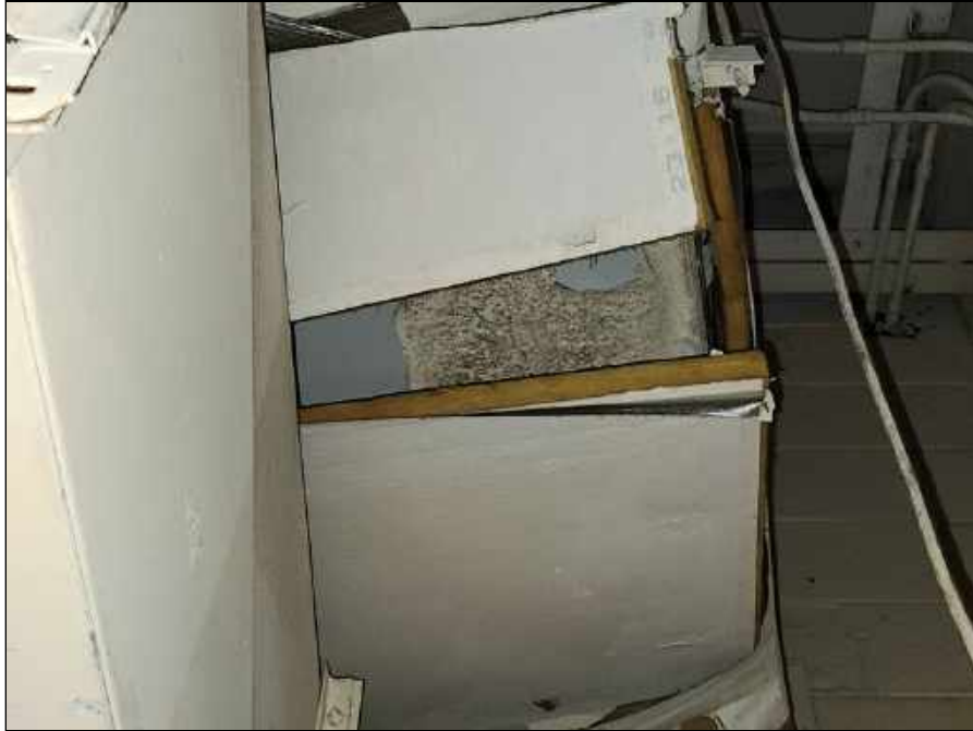
41 - Mold on HVAC duct insulation adhesive by the stage (left)
