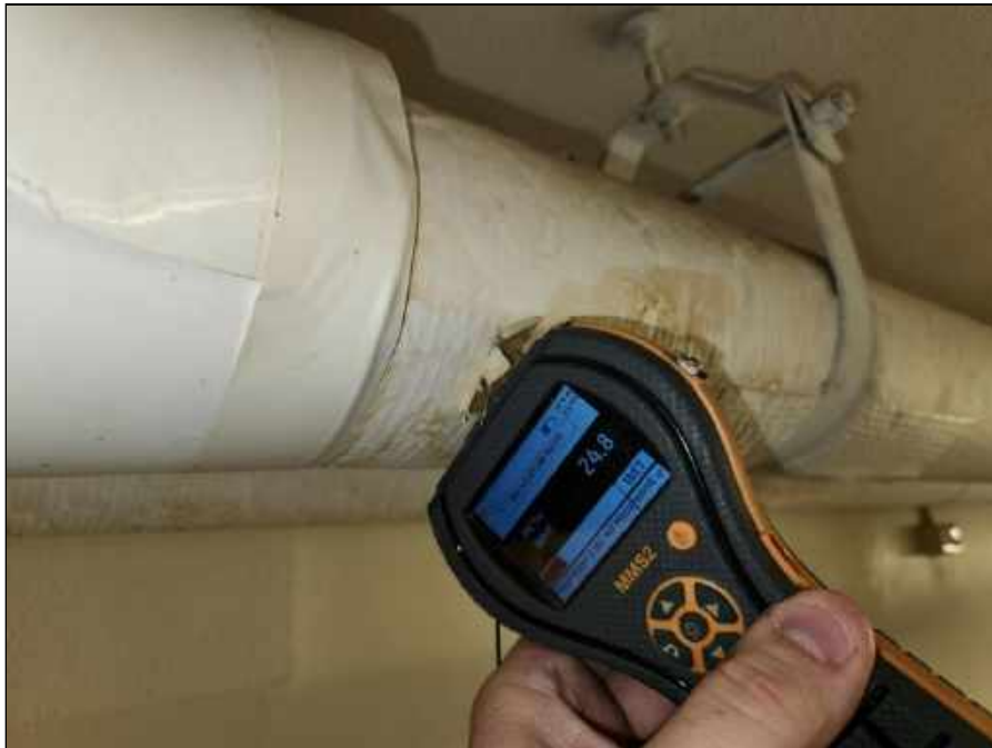
8 - Elevated moisture meter reading collected from pipe insulation in Room 102
