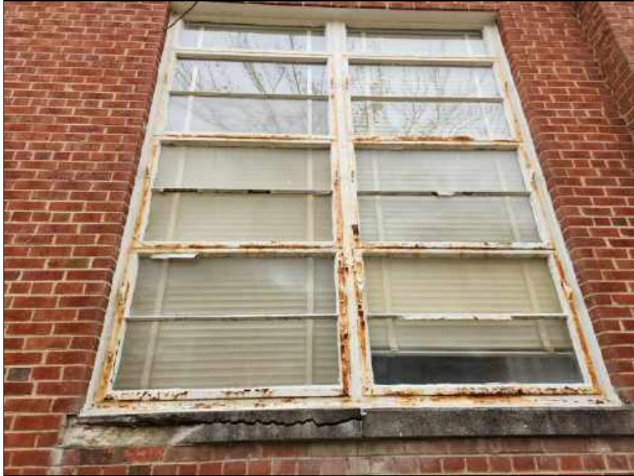
1 - Rusted window frame and damaged window ledge at an Auditorium window
