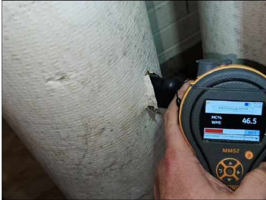
43 - Elevated moisture meter reading collected from pipe insulation - by stage (right)
