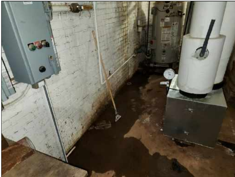
46 - Standing water on the floor of the boiler room caused by water leaking from the wall (exterior)
