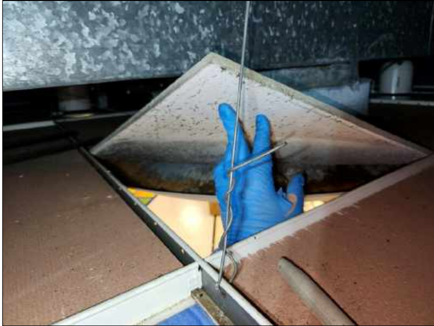
3 - Mold impacted ceiling tiles above the large HVAC supply vent in classroom 103 and evidence of moisture accumulation within the vent
