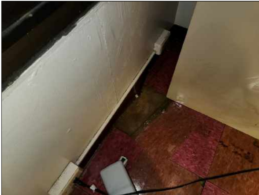
50 - Moisture damaged drywall and water on the floor in Room 126
