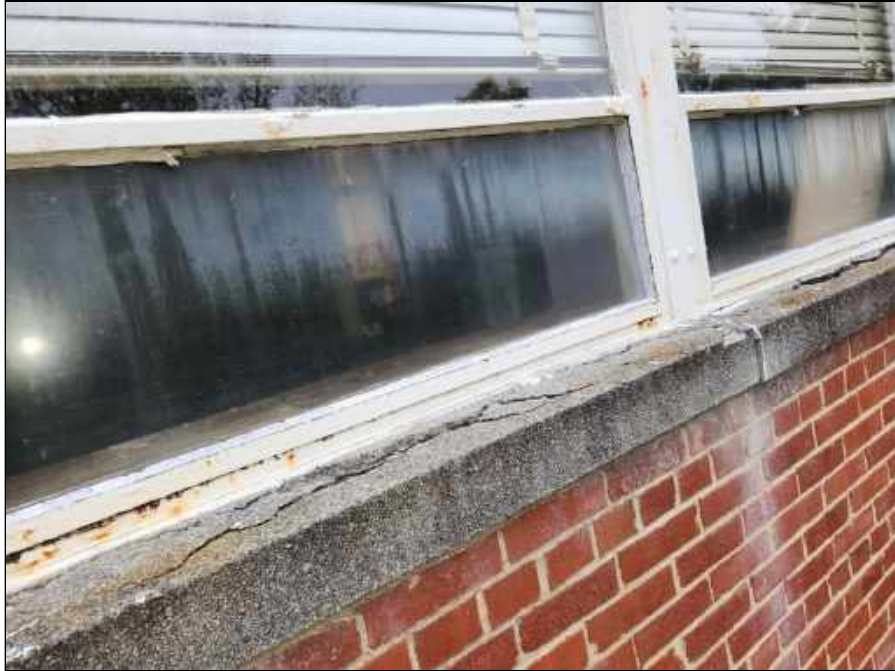
9 - Damaged window ledge on the East side of the building
