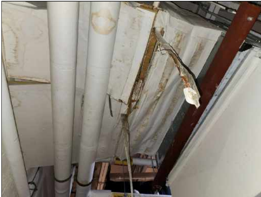
40 - Moisture stained HVAC duct insulation by the stage (right)
