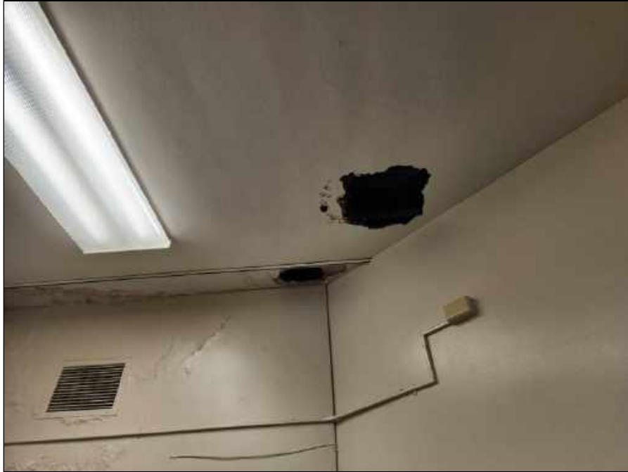
13 - Moisture damaged plaster ceiling observed in Room 111 observed on 10-18-23
