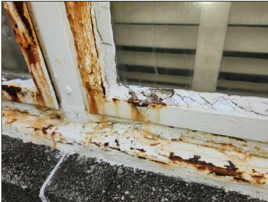
2 - Damaged window glazing at an Auditorium window
