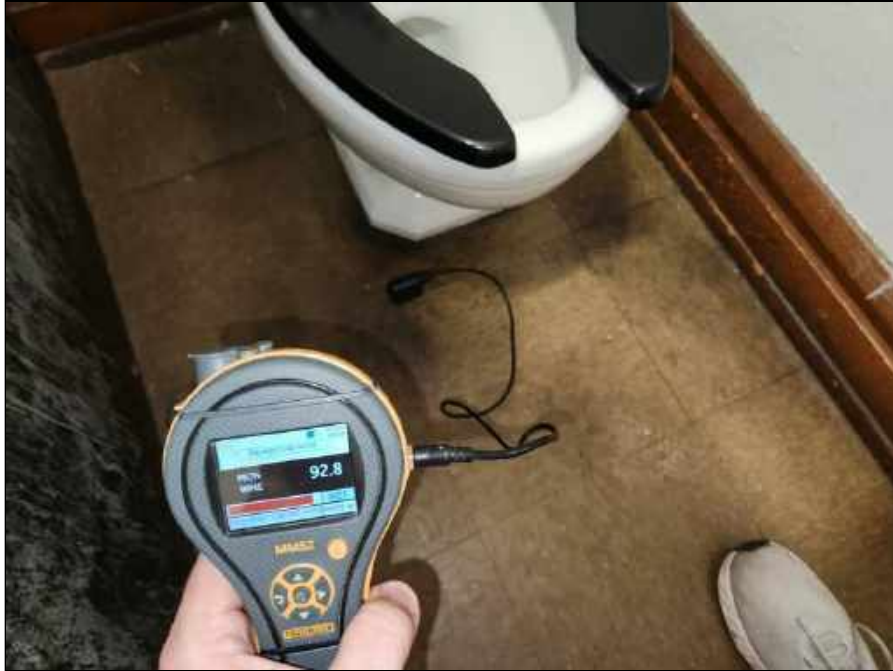
33 - Elevated moisture meter reading in the 2nd floor office between 219 and 220 indicating moisture is trapped beneath the floor tile
