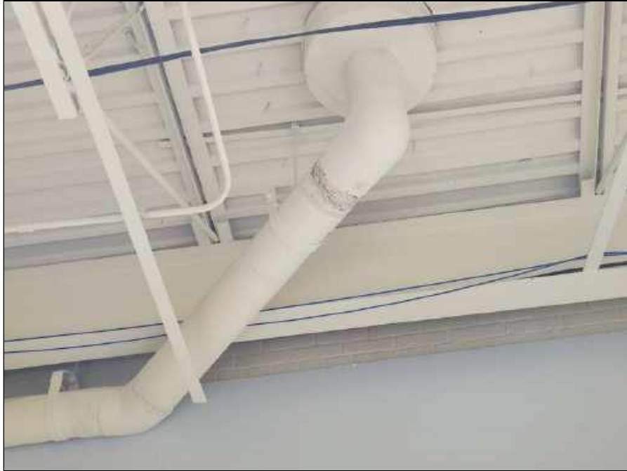
23 - Mold observed on roof drain pipe insulation in the library
