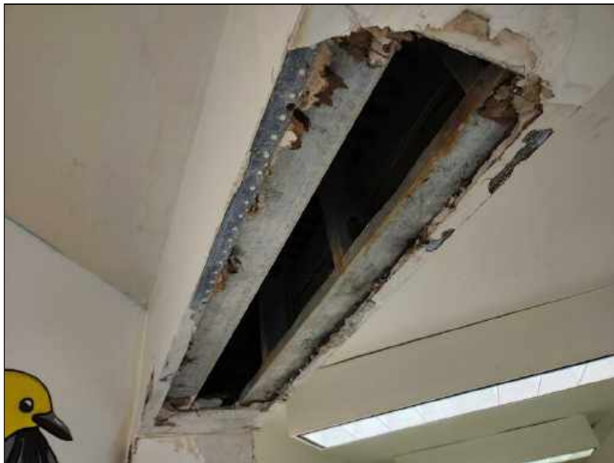
12 - Moisture damaged drywall observed in library hallway on 10-18-23
