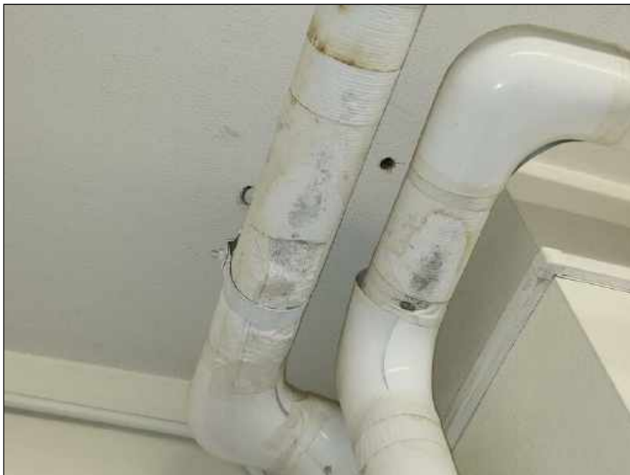
2 - Mold on pipe insulation in Room 101
