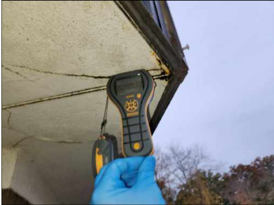
7 - Damaged soffit and elevated moisture meter reading
