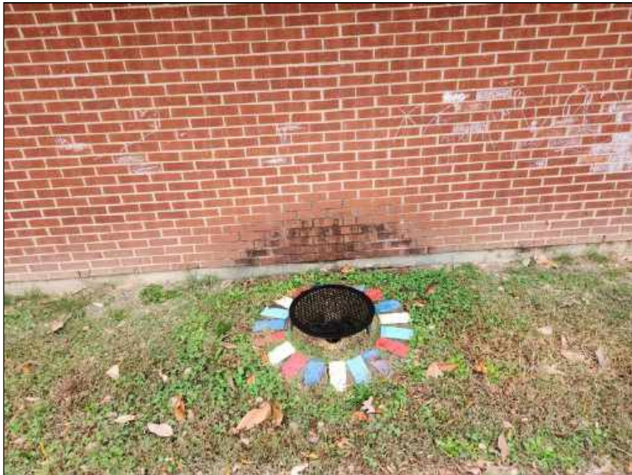
4 - A downspout draining against the foundation
