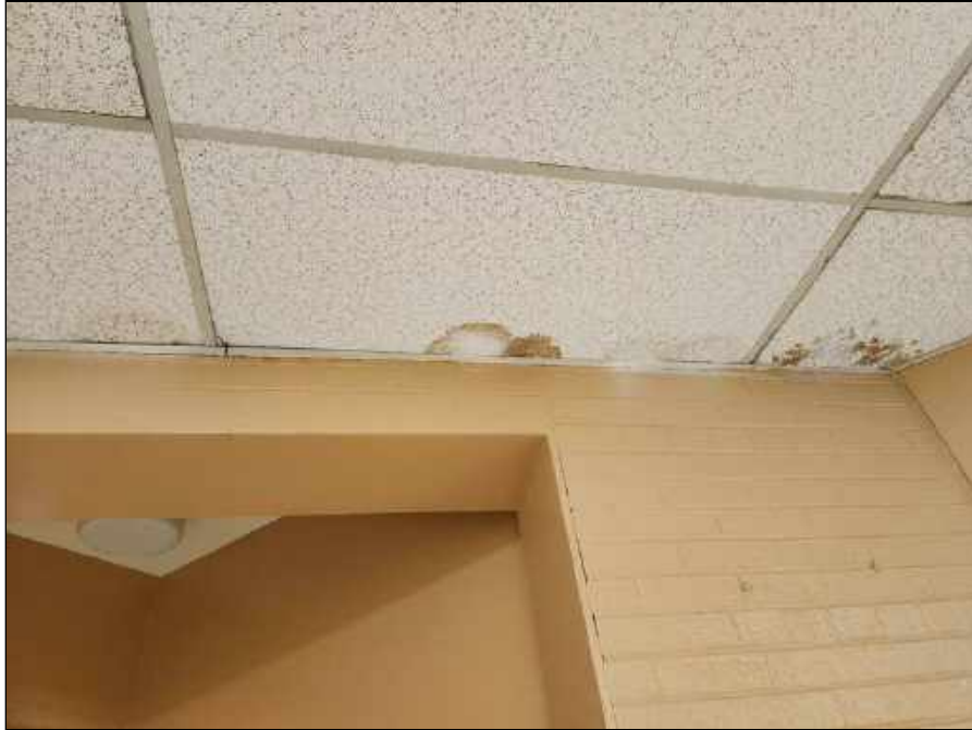
21 - Moisture impacted ceiling tiles in Room 112
