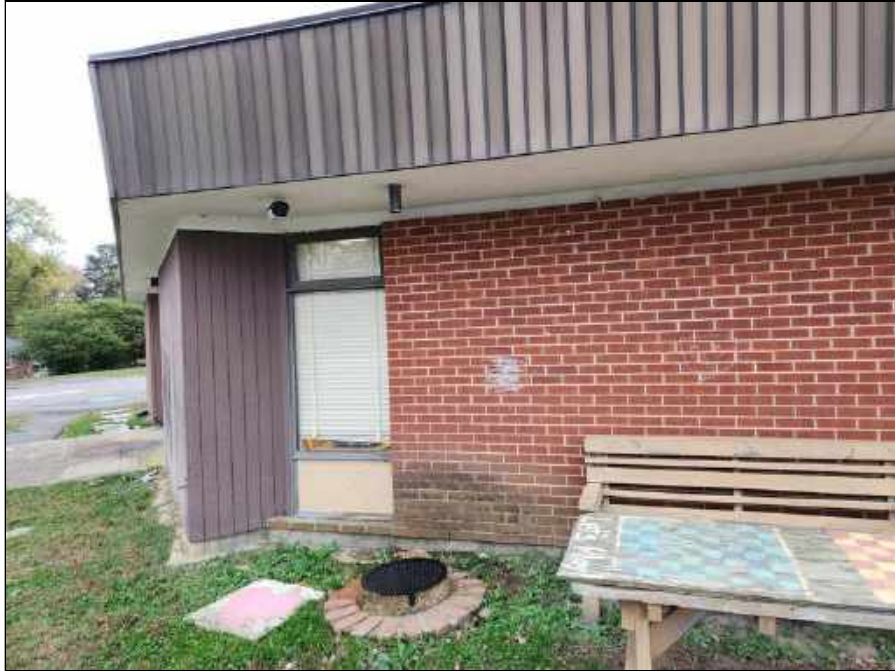
3 - A downspout draining against the foundation
