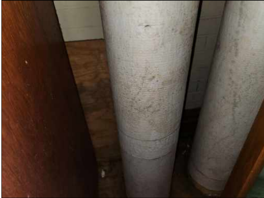
39 - Mold on pipe insulation by the stage (right)
