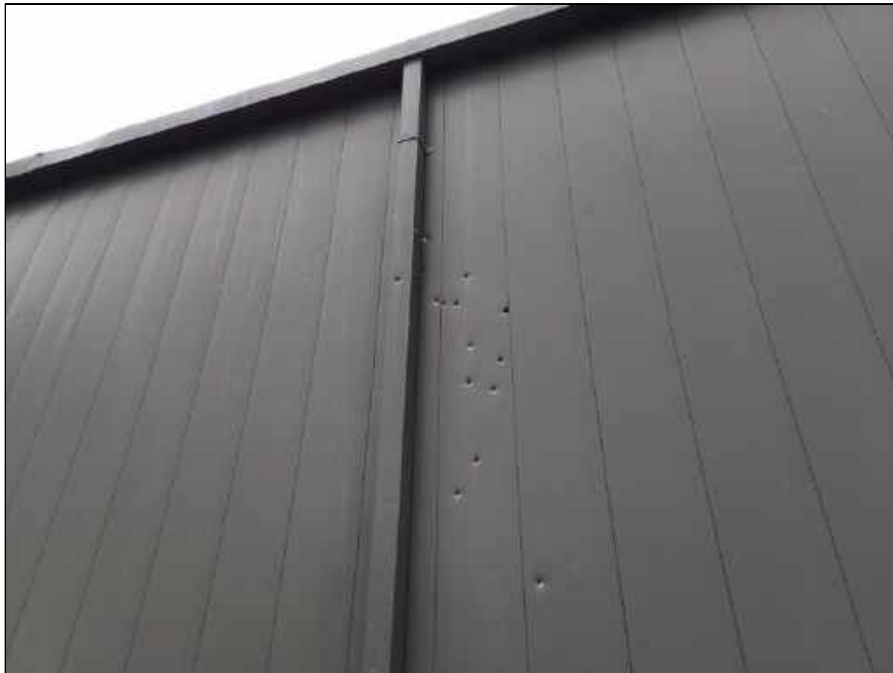
6 - Apparent bullet holes in the exterior metal panels on the Activities portion of the building
