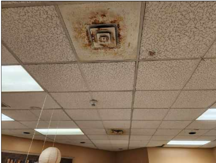
22 - Significant rusting on HVAC diffusers in Room 112
