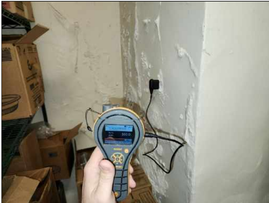
28 - Elevated moisture meter reading collected from the plaster wall in the kitchen by the container storage indicating that the wall is saturated
