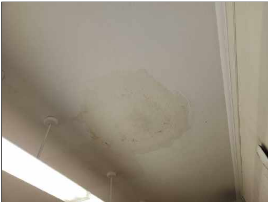
34 - Moisture impacted plaster ceiling in Room 218
