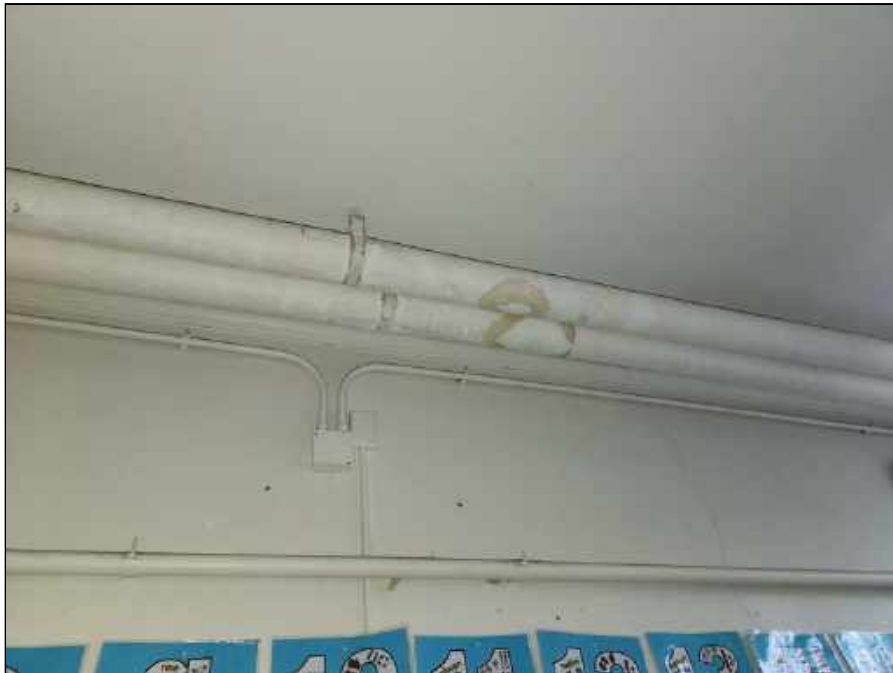
6 - Moisture stained pipe insulation in Room 107
