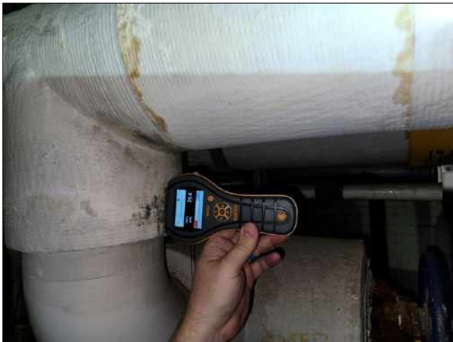
30 - Mold and moisture impacted pipe insulation above the ceiling in the Teacher's Lounge indicating elevated moisture. Elevated moisture readings detected.
