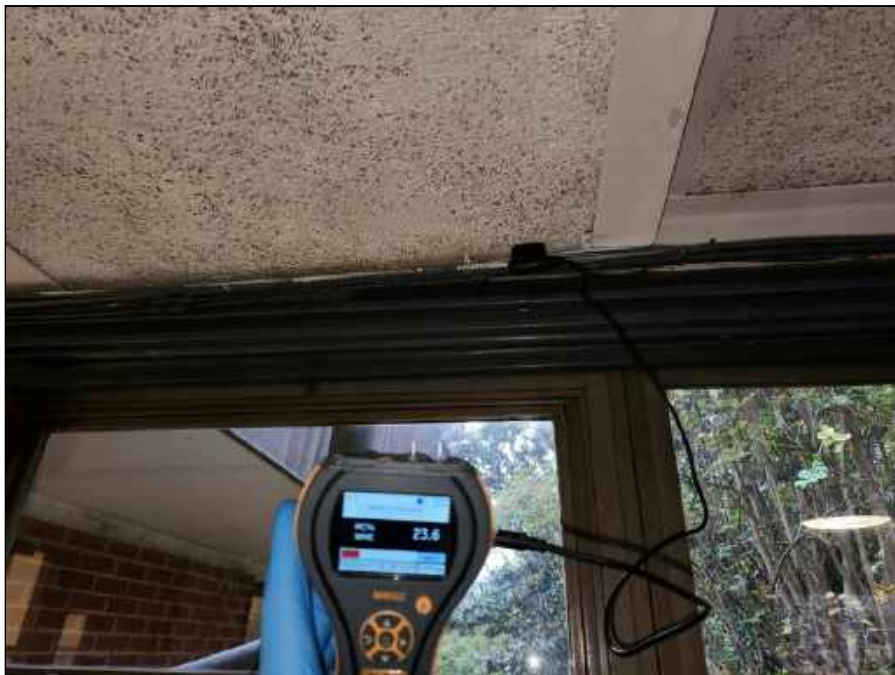
2 - Elevated moisture meter reading collected from the tectum ceiling in the pod connector hall
