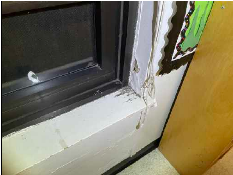
48 - Moisture damaged plaster wall in Room 124 - Activities Room
