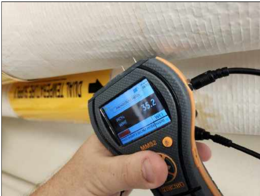
4 - Elevated moisture meter reading collected from impacted pipe insulation in Room 101
