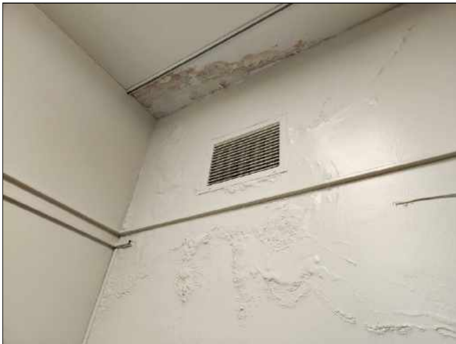
14 - Moisture damaged plaster wall observed in Room 111 on 10-18-23
