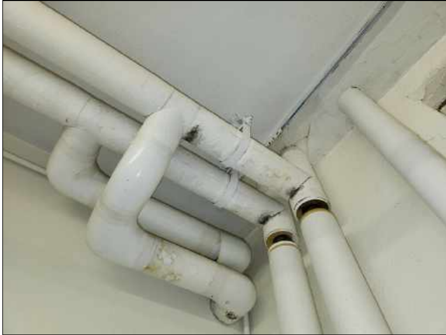
9 - Mold on pipe insulation in Room 102
