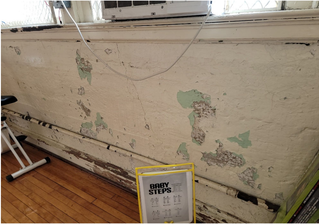
Photograph No. 3 Old/Dry Water Damage - Multi-Purpose Room
