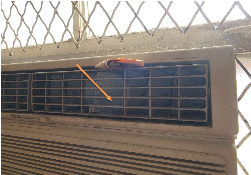
Photograph No. 2 Visible Mold Growth - Multi-Purpose Room
