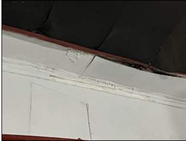
9 - Damaged plaster wall and ceiling from a possible roof leak in the Auditorium.
