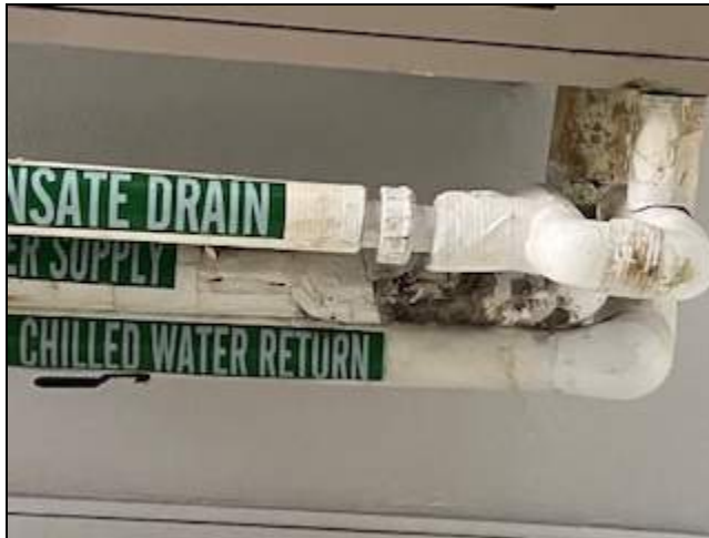
2 - General view of ceiling mounted fan coil unit pipes with visible mold.
