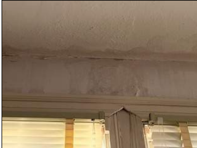
7 - View of damaged plaster from water intrusion in room 307
