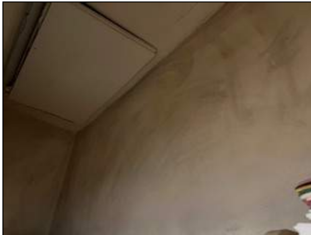
8 - Room 304 closet where it appears cleaning was conducted. Suspect mold was observed on the wall however.
