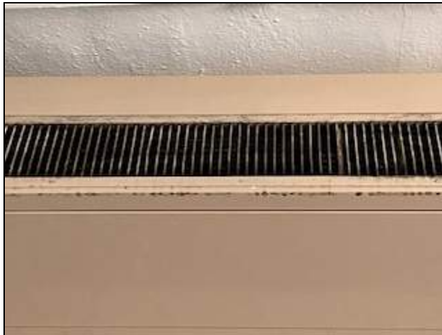
4 - General view of ceiling mounted fan coil unit which contains heavy dust and suspect mold.
