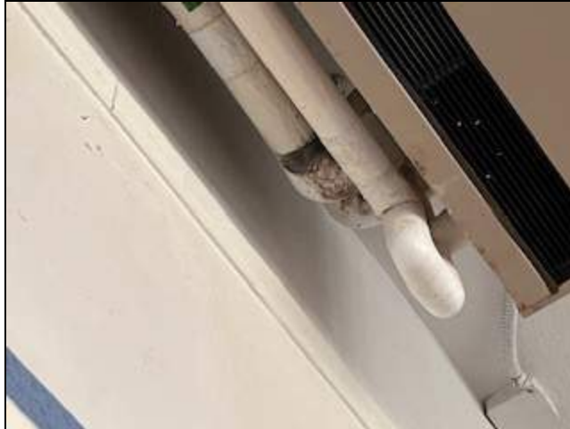
3 - General view of ceiling mounted fan coil unit pipes with visible mold.
