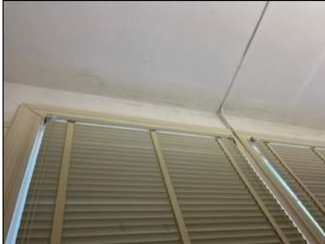
5 - View of plaster ceiling showing water damage from possible roof leaks in room 303.
