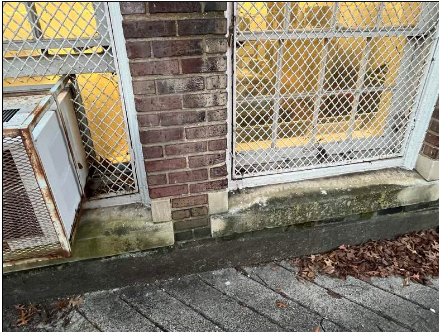
12 - View of the window outside room 101 where heavy staining was observed. The windowsill appeared to be damaged from water intrusion.
