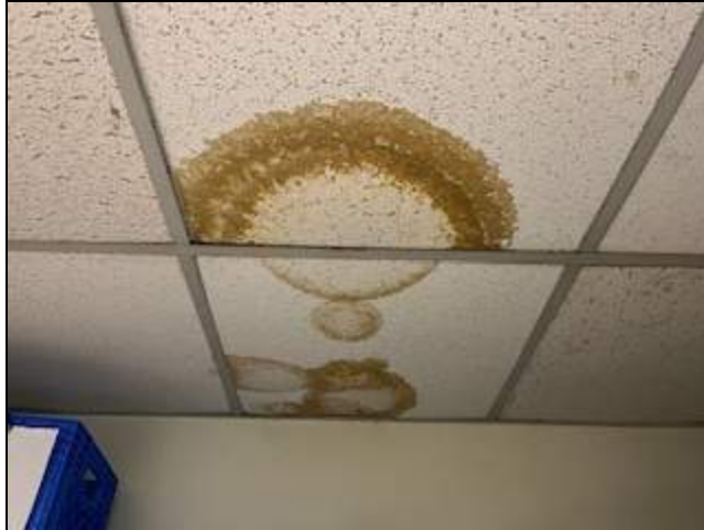
1 - General view of ceiling tile with water intrusion.
