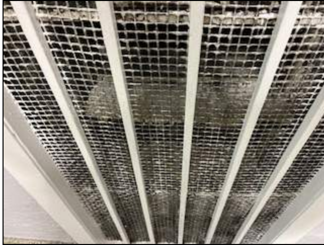
11 - Vent grate near main entrance with heavy dust observed.
