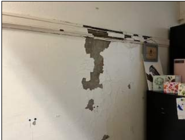
6 - View of damaged plaster wall in the office space near the media center on the 3rd floor.
