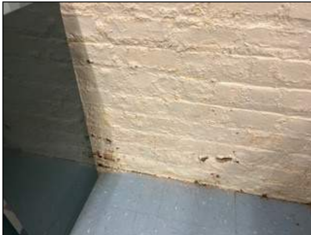
10 - Brick wall where ECS observed moisture intrusion / damage on the lower half of wall in room 101.
