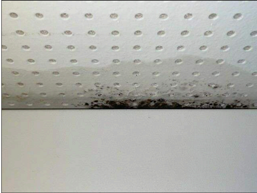
19 - Mold on ceiling tiles above the fan coil unit in the Library
