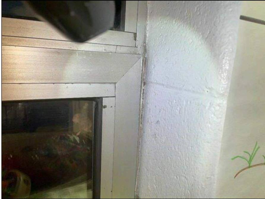
13 - Mold on window frame caulking in an East wing classroom
