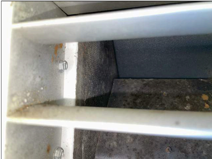
10 - Mold observed within the ceiling mounted fan coil in Room 105
