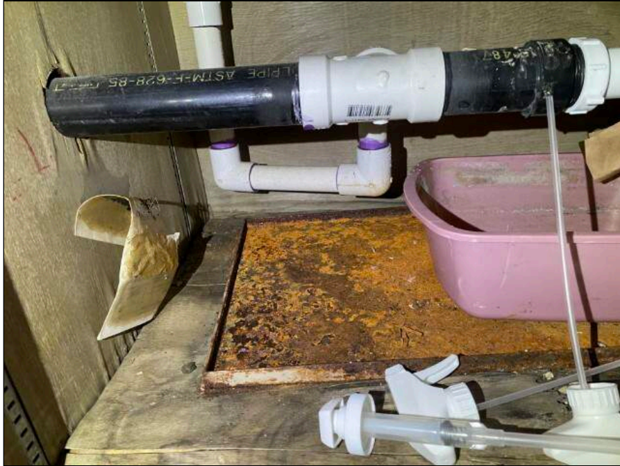
17 - Mold observed in the sink cabinet in Room 106
