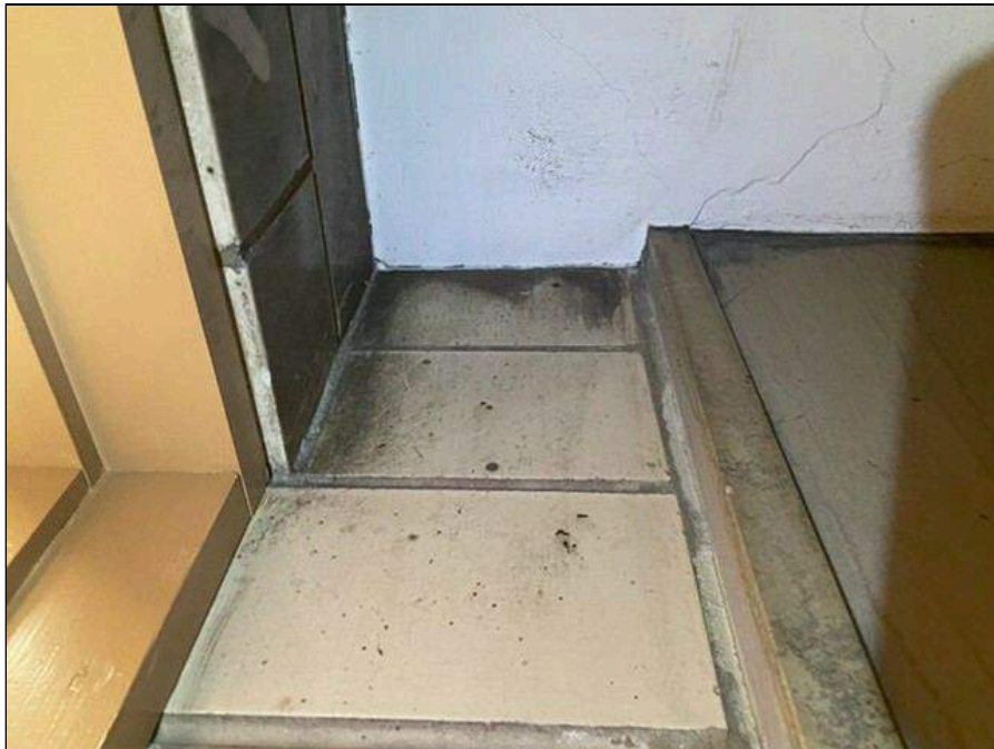
4 - Mold observed on the walls in the shower in the Boy's Room
