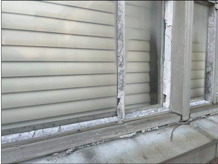
1 - Damaged asbestos containing window caulk and glazing
