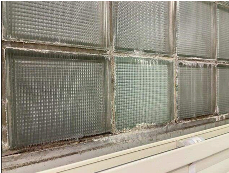
8 - Staining indicating water intrusion through the glass block windows in Room 106
