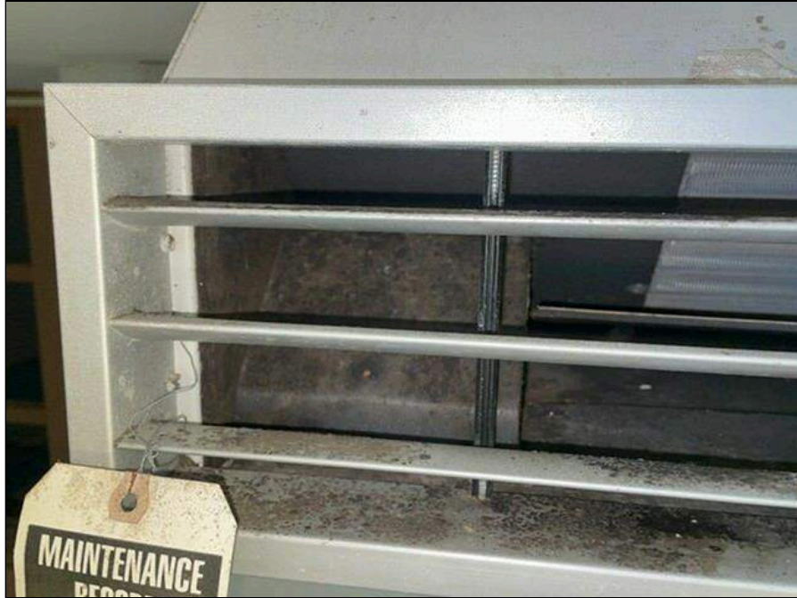
11 - Mold observed within the ceiling mounted fan coil in Room 107
