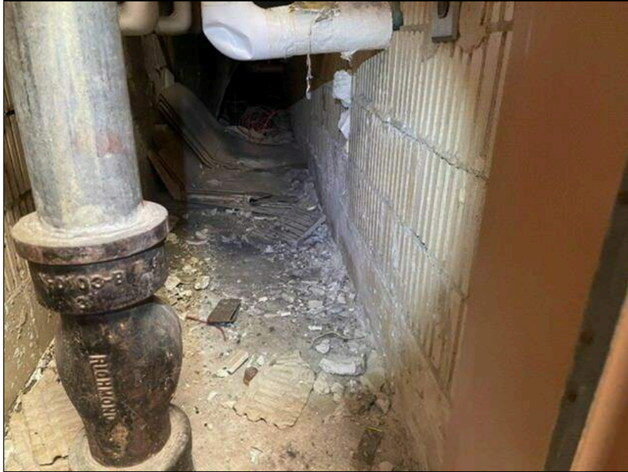
5 - Mold impacted debris on the floor of the wet wall chase between the hall bathrooms
