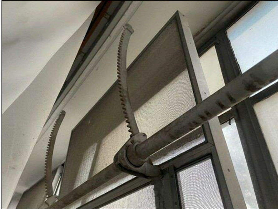
1 - Window apparently stuck open in the Cafeteria
