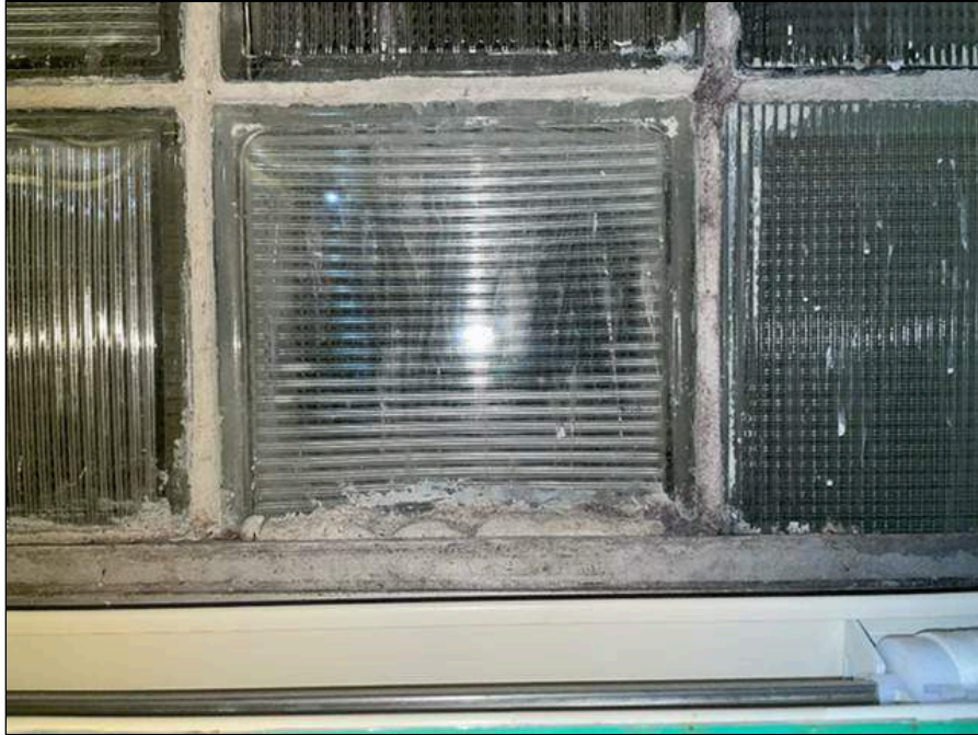
7 - Mold on the glass block window mortar in Room 105
