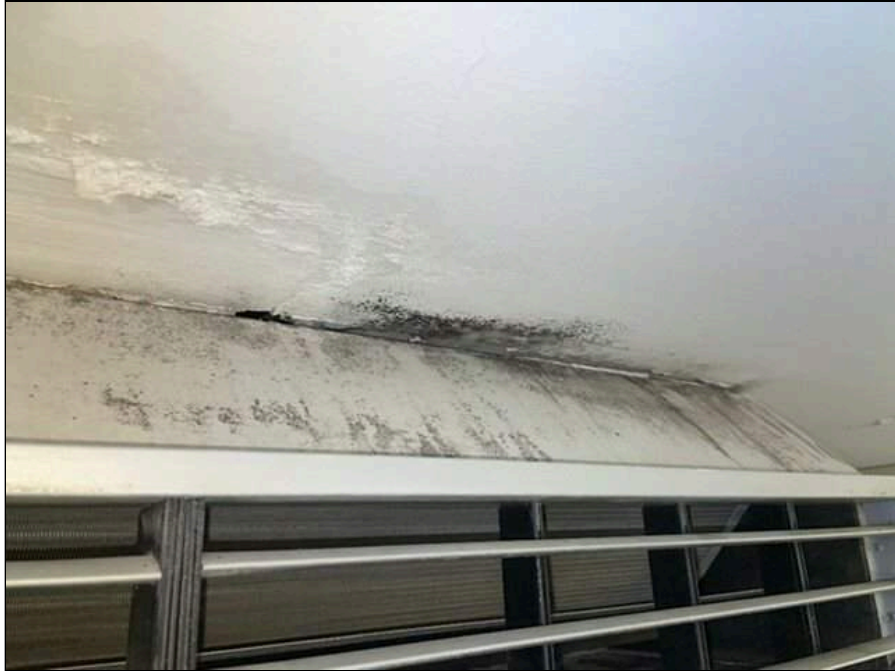
9 - Mold on and above a ceiling mounted fan coil in Room 15
