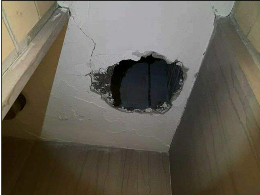
3 - Damaged plaster ceiling in the shower in the Boy's Room
