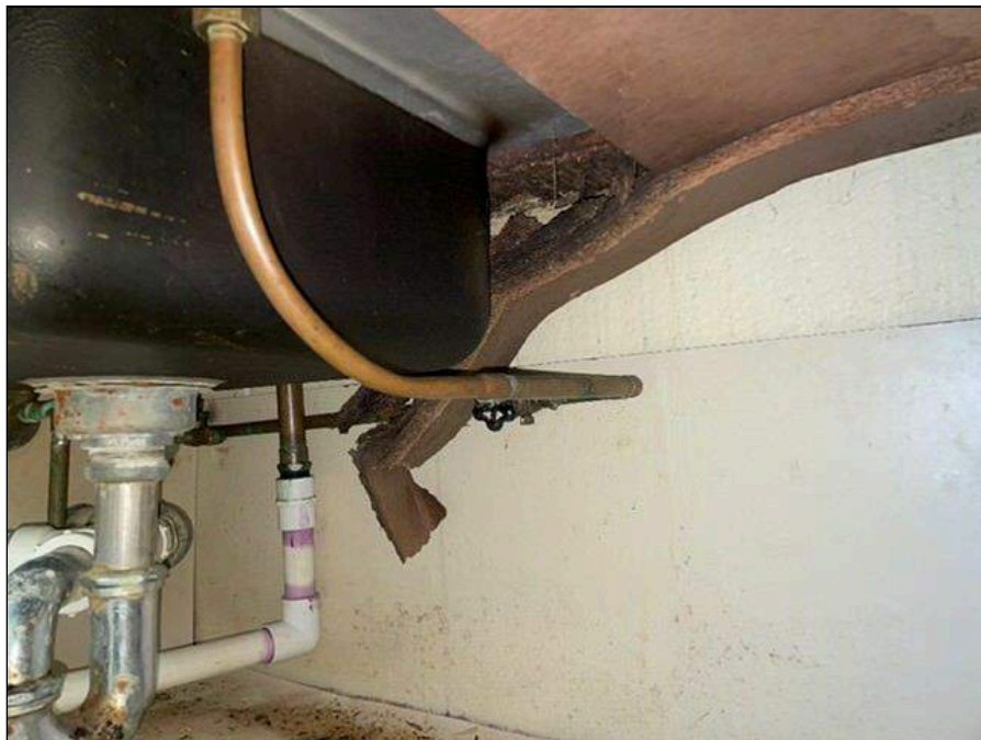
12 - Moisture damaged sink cabinet countertop in Room 113
