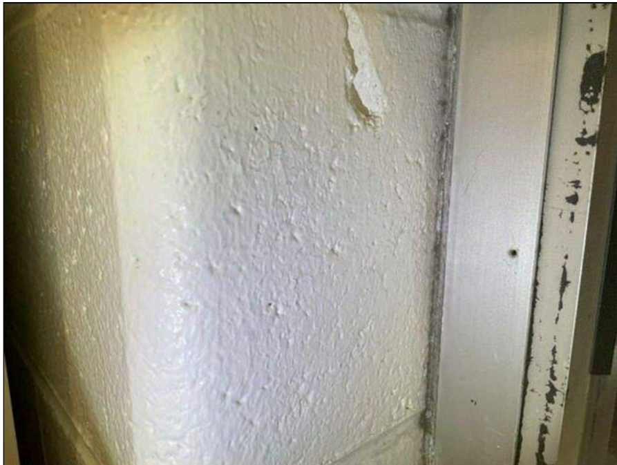
14 - Mold on window frame caulking in an East wing classroom
