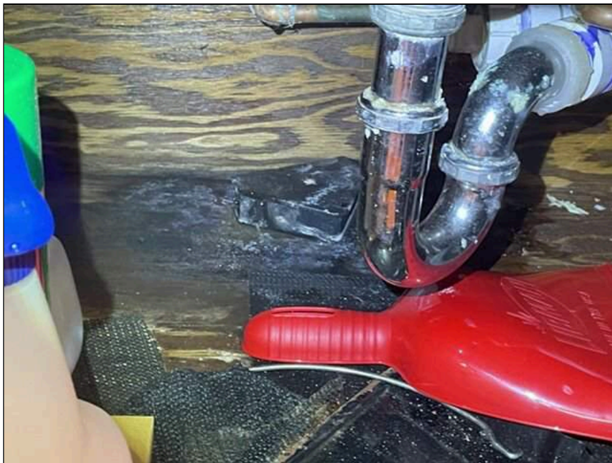
18 - Mold observed in the sink cabinet in Room 112
