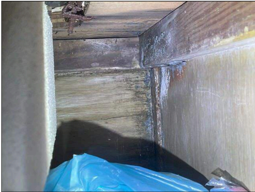
16 - Mold observed in the sink cabinet in Room 104
