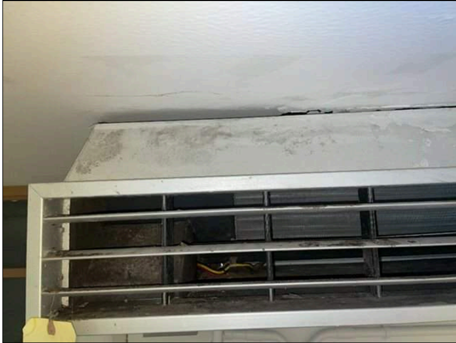
15 - Mold observed on a ceiling mounted fan coil in Room 102
