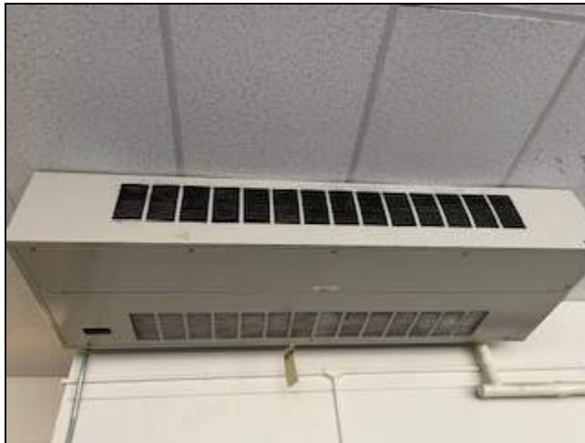
4 - General view of ceiling mounted HVAC unit with suspect mold on supply diffuser.
