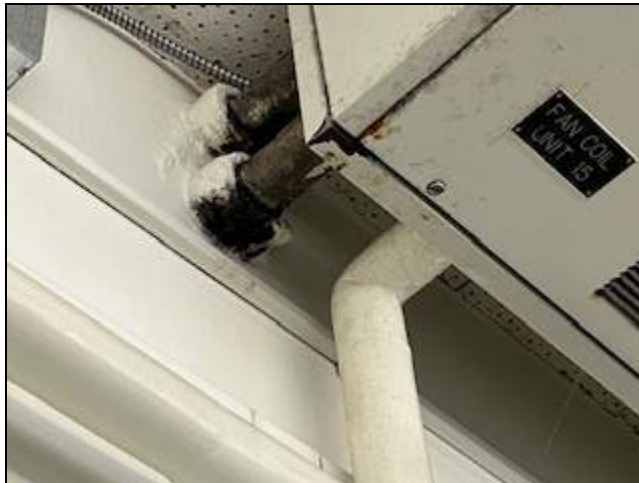
6 - General view of pipe with suspect mold associated with a ceiling mounted HVAC unit.
