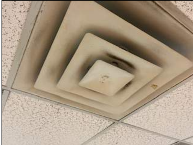
1 - General view of supply vent showing heavy dust accumulation.
