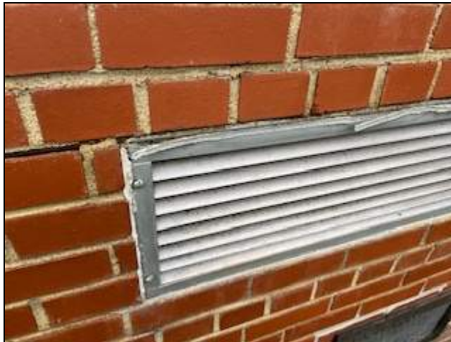
16 - View of exterior wall vent with caulk peeling and falling out.
