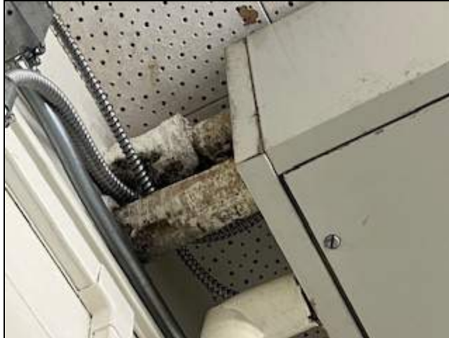
5 - General view of pipe with suspect mold associated with a ceiling mounted HVAC unit.
