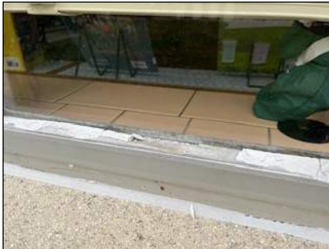
14 - View of damaged window glazing from weathering.
