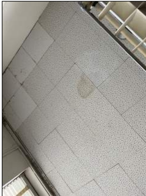
2 - General view of ceiling tiles with water staining.
