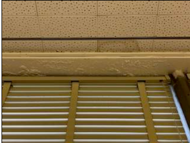
7 - View of the window lintel having signs of water intrusion within room 203.
