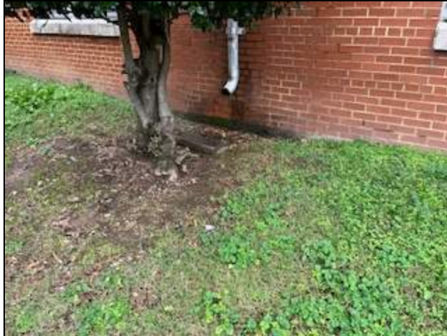
15 - View of roof drain draining against the foundation.
