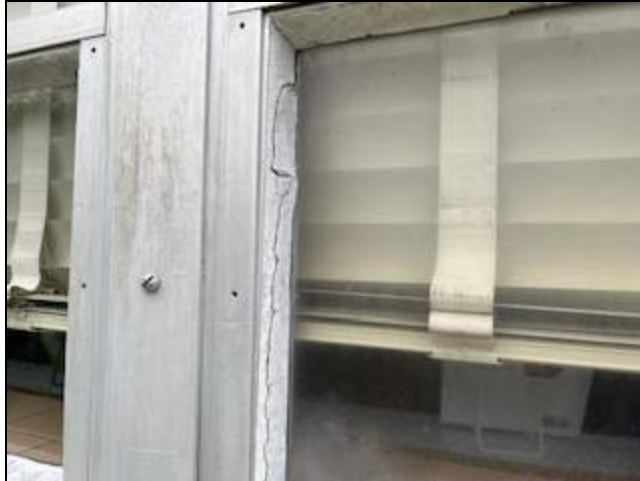
13 - View of degraded window glazing from weathering.
