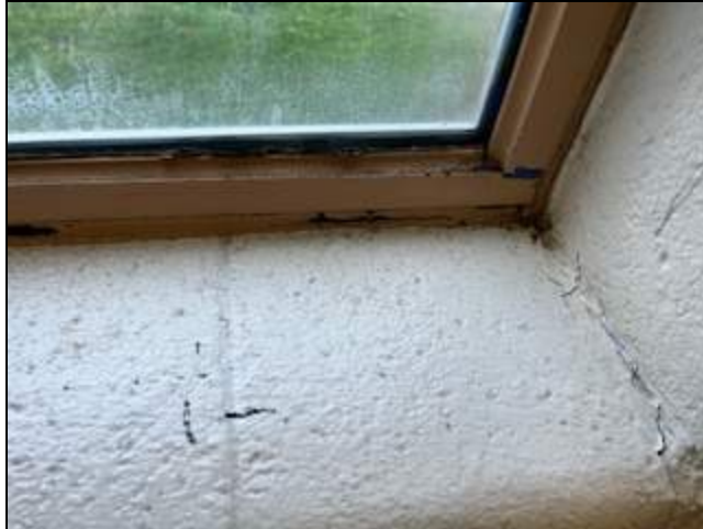
9 - Window in room 112 showing peeling paint possibly from water intrusion from caulk failure.
