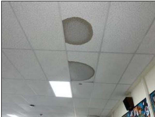
8 - Cafeteria - stained /water impacted ceiling tile showing active water leak from roof.
