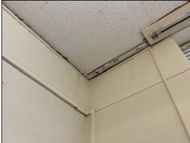
11 - View of damaged ceiling tile and wall showing staining from a previous leak.
