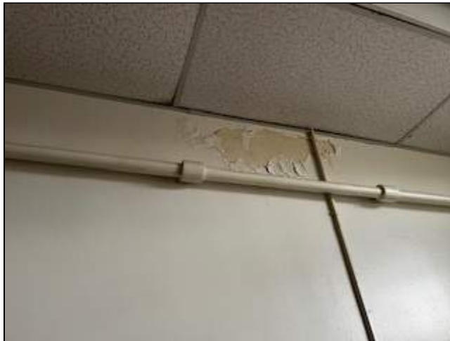
10 - View of wall bubbling/peeling paint from possible water intrusion in room 208.
