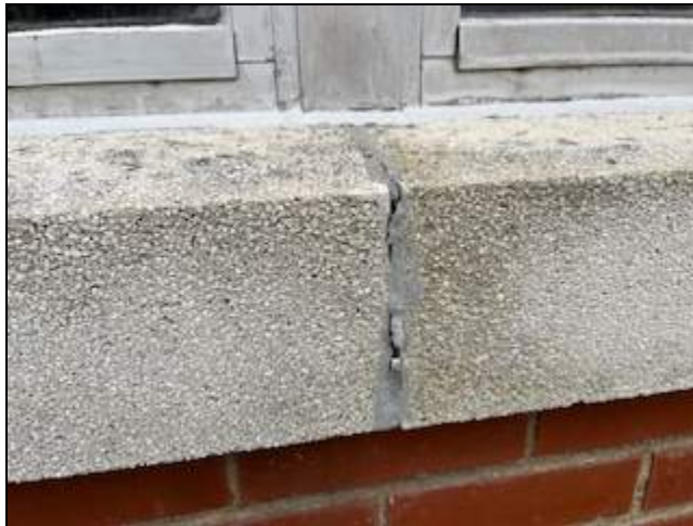
12 - View of exterior window sill with damaged caulk/sealant.
