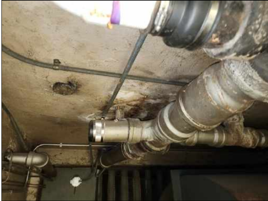
17 - Mold and moisture impacted plaster ceiling in the basement fan room
