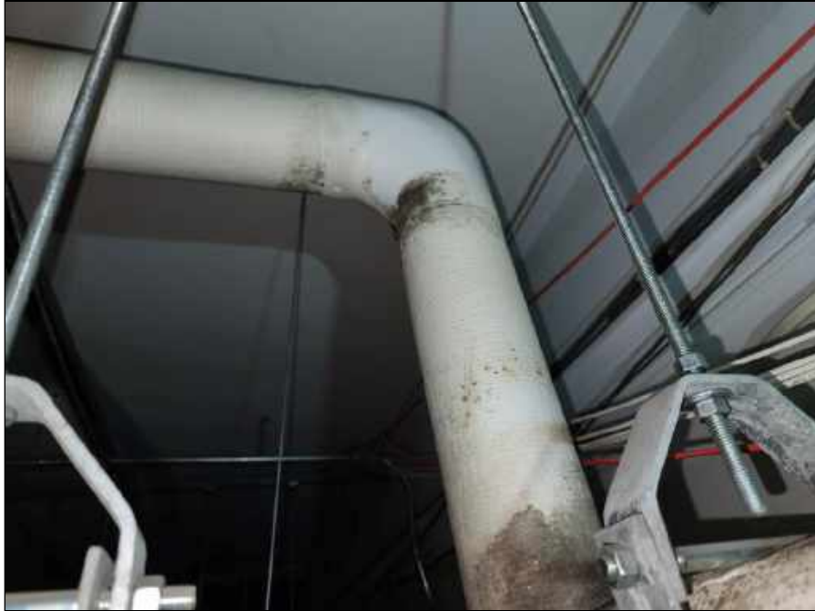
23 - Mold on pipe insulation above the ceiling in the 2nd floor hallway
