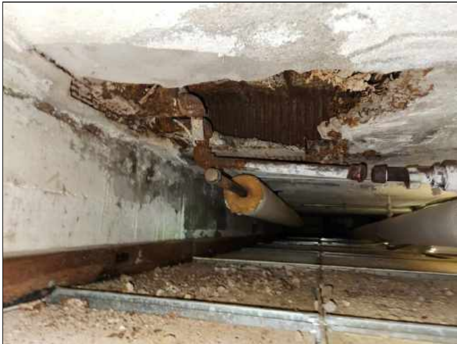
14 - Moisture damaged plaster ceiling in the basement outside of the boiler room
