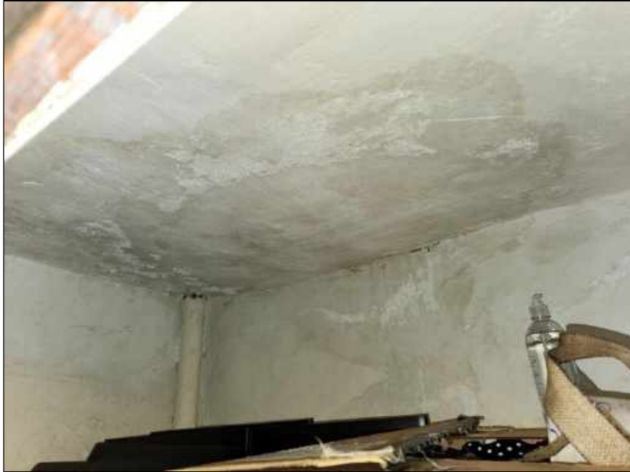
31 - Moisture stained plaster ceiling in the closet in Room 301
