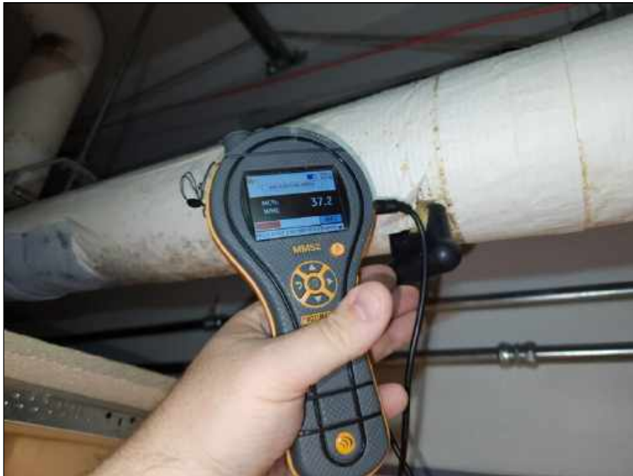
24 - Elevated moisture meter reading associated with the mold impacted pipe insulation
