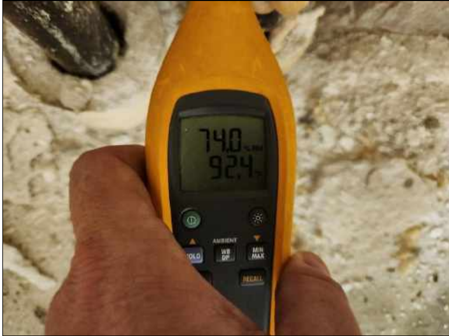
5 - Elevated relative humidity near the moisture damaged plaster wall
