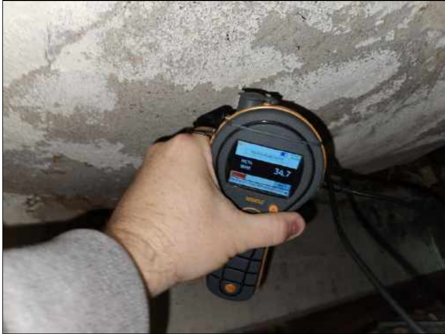
15 - Elevated moisture meter reading associated with the plaster ceiling outside of the boiler room
