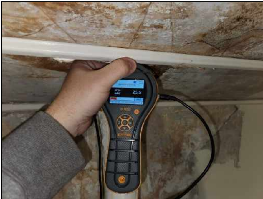
28 - Elevated moisture meter reading associated with the damaged plaster ceiling
