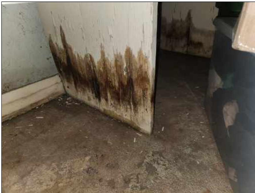
38 - Mold impacted storage shelves in the Coats for Communities storage room in the basement
