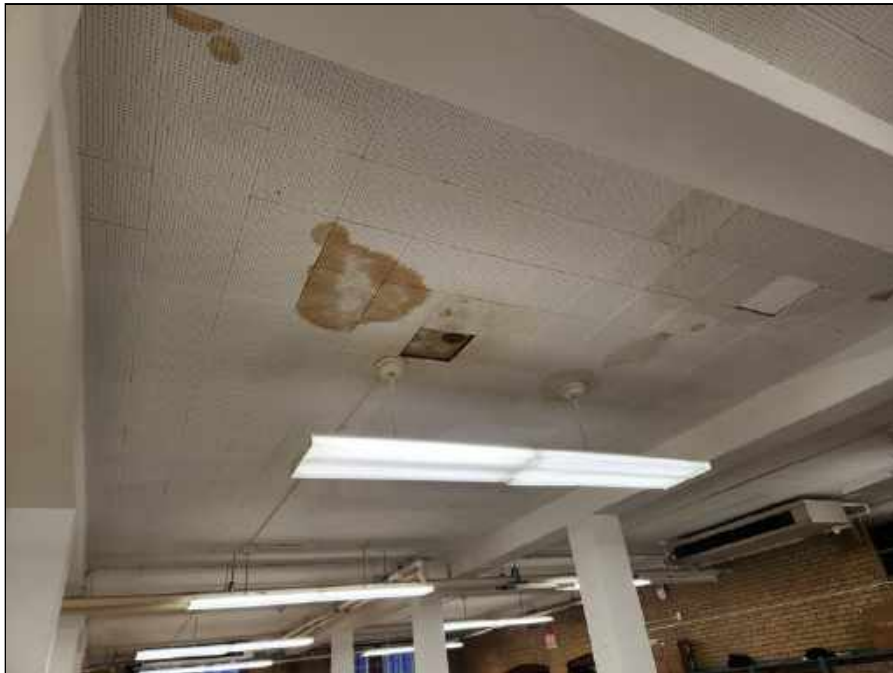
2 - Moisture damaged ceiling tiles in the cafeteria
