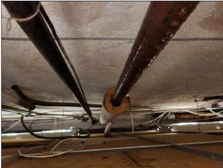
12 - Un-insulated condensating pipe above the ceiling in the band room
