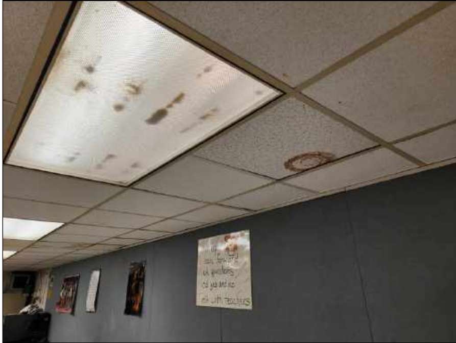
7 - Moisture stained ceiling tiles in the band room
