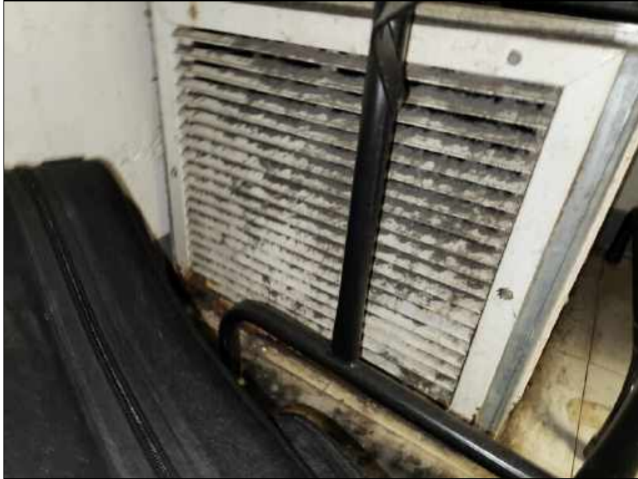
13 - Mold on the air handler return in the band room
