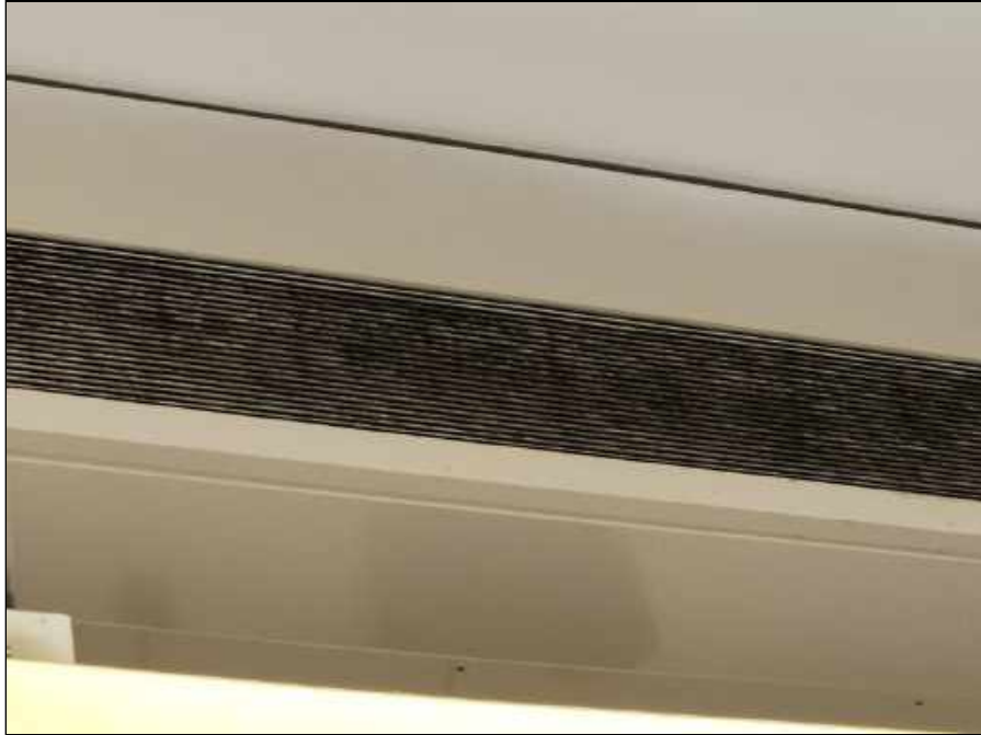
29 - Mold on the ceiling mounted fan coil in Room 301
