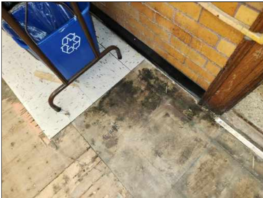
20 - Mold impacted sub-floor in Room 212
