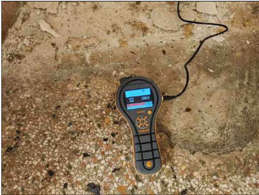
6 - Moisture meter reading indicating a portion of the damaged plaster wall is wet
