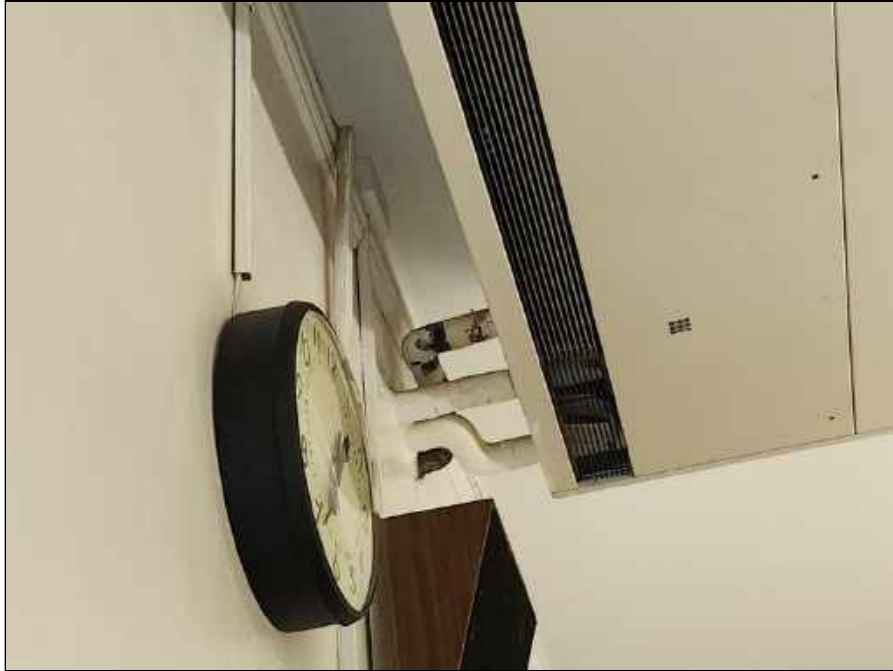
21 - Mold on pipe insulation in Room 216
