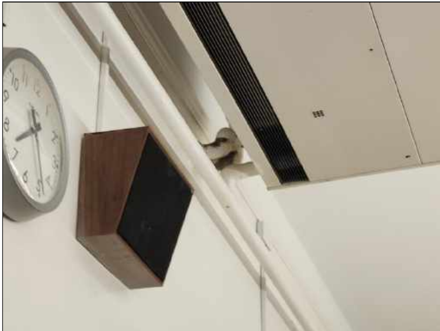
30 - Mold on pipe insulation in Room 301
