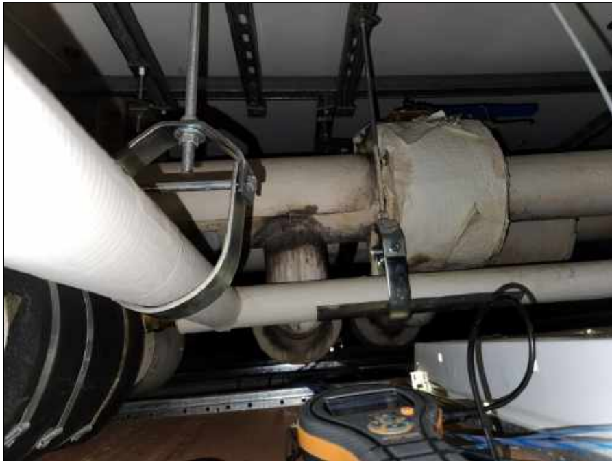
18 - Mold on pipe insulation above the 2nd floor ceiling
