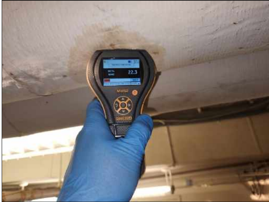
39 - Elevated moisture meter reading from pipe insulation in Ms. Macklin's office in the basement
