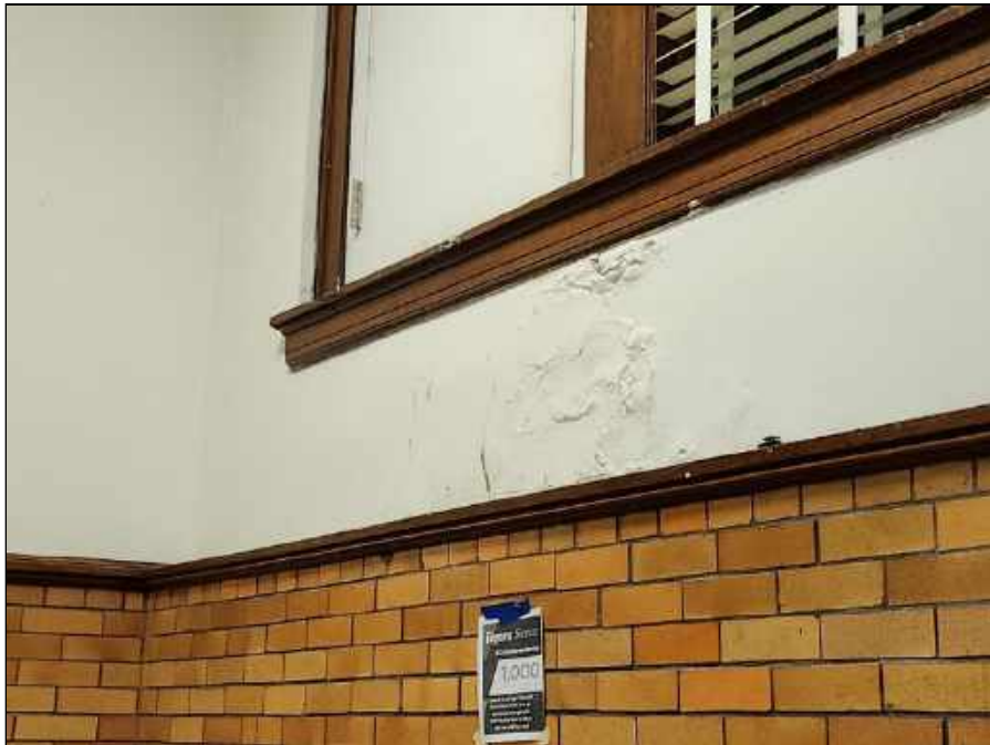
32 - Moisture damaged plaster wall in the 3rd floor hallway
