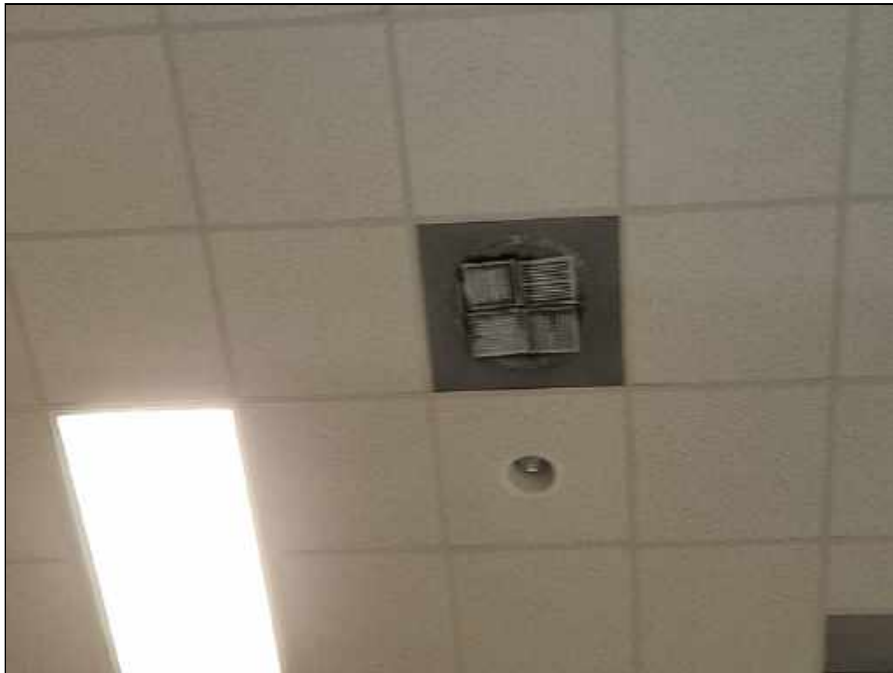
34 - Suspect mold on HVAC supplies in the Auditorium
