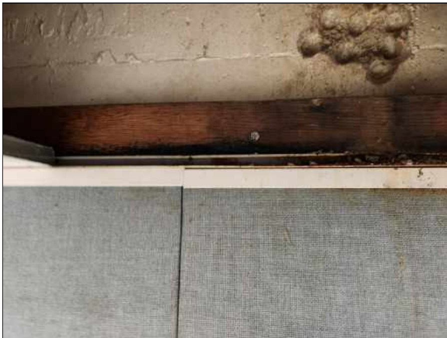
10 - Mold on wood framing above the ceiling in the band room
