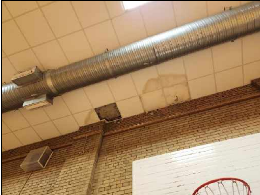
25 - Moisture damaged drop ceiling and plaster ceiling in the gym
