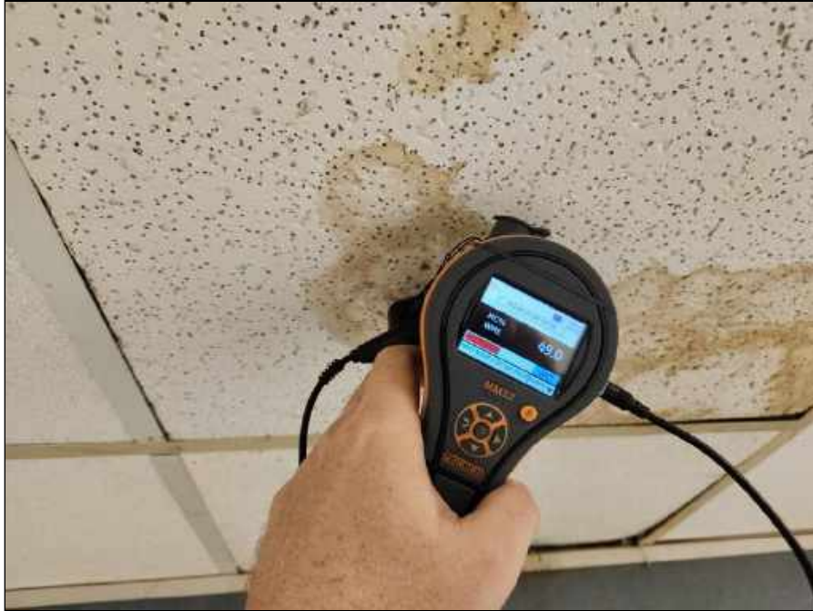
11 - Elevated moisture meter reading collected from ceiling tile in the band room
