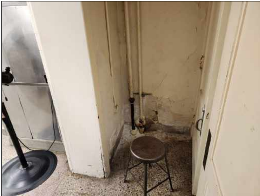
4 - Moisture damaged plaster wall in the kitchen
