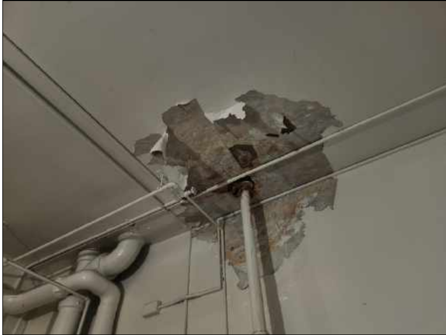
27 - Moisture damaged plaster ceiling in the girl's locker room
