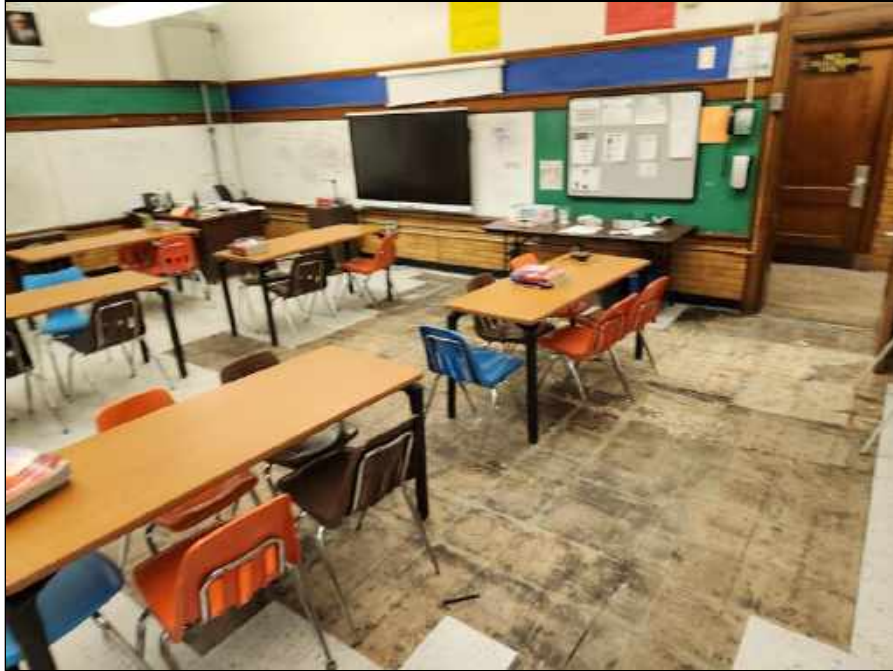
19 - Moisture impacted sub-floor in Room 212
