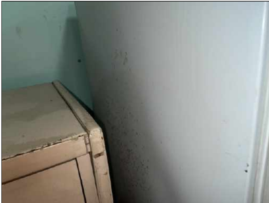
36 - Mold on the plaster wall beside the sink in Room 111
