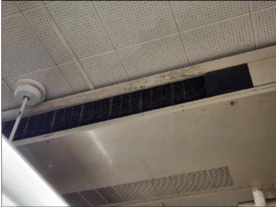
3 - Mold on the ceiling mounted fan coil in the cafeteria
