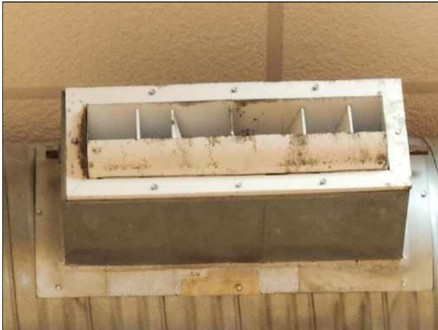
26 - Suspect mold on the HVAC supply ducts in the gym
