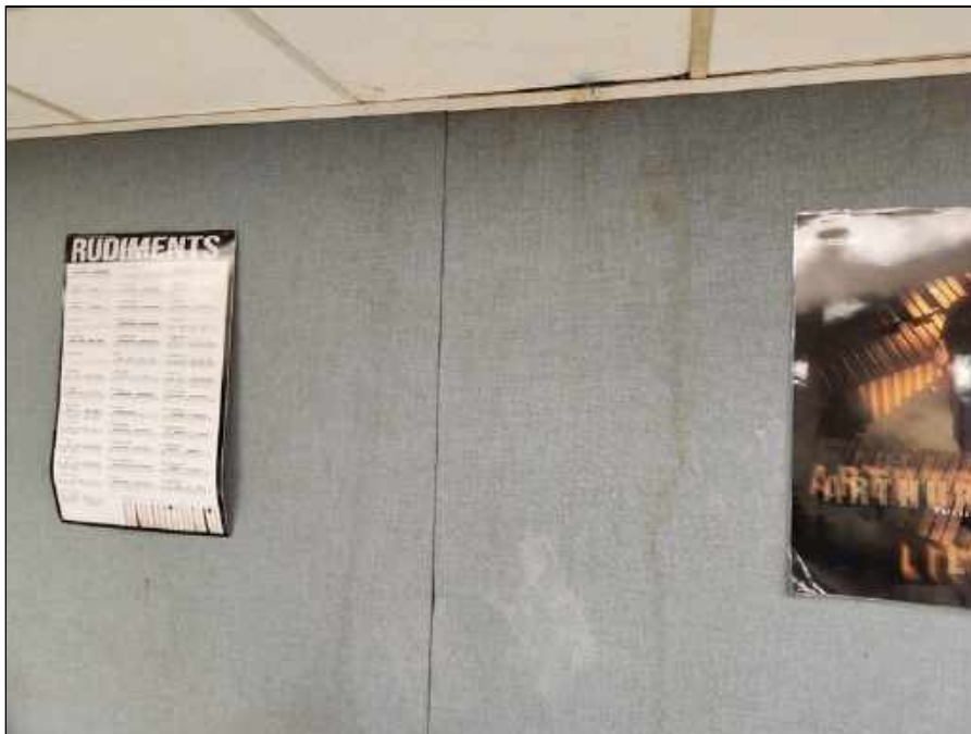
8 - Moisture stained wall panels in the band room
