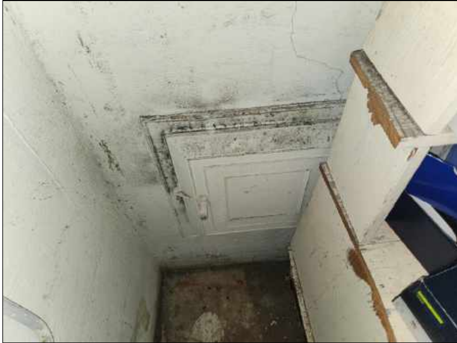
37 - Mold impacted access door and wall in the Coats for Communities storage room in the basement
