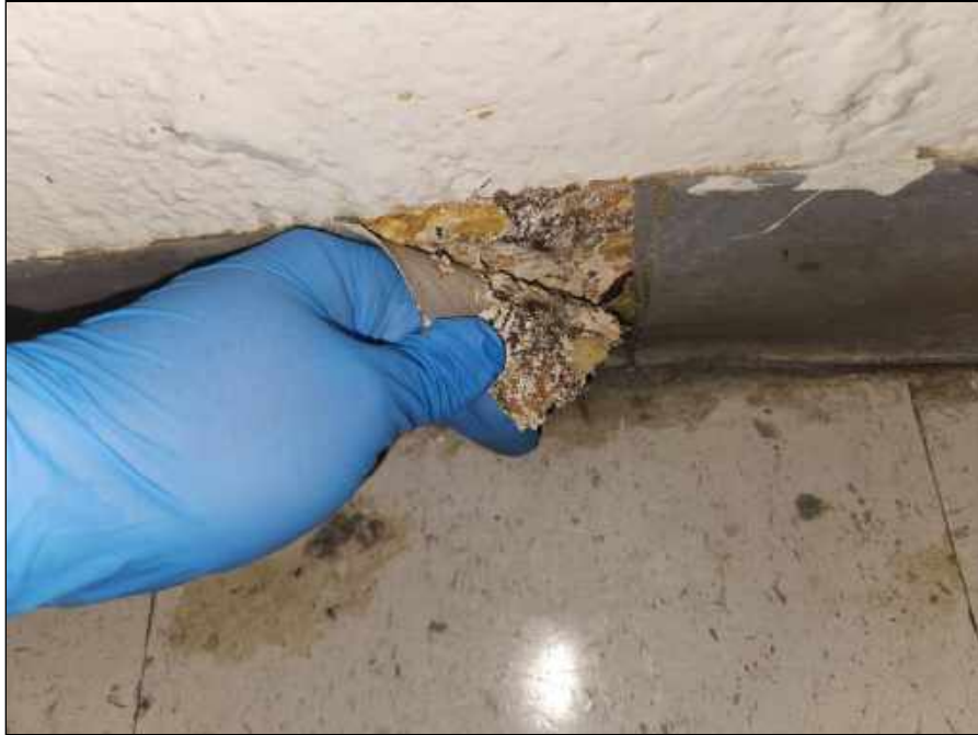
9 - Mold behind vinyl cove baseboard in the band room
