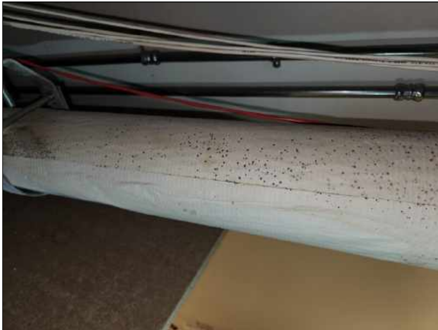
22 - Mold on pipe insulation above the ceiling in the 2nd floor hallway
