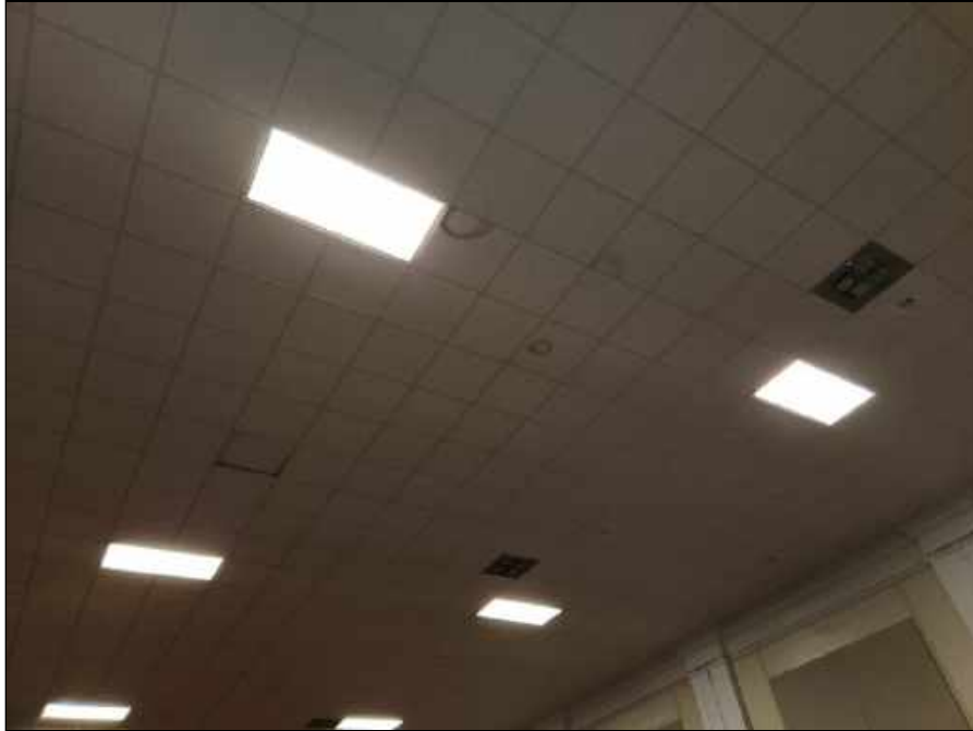
33 - Moisture stained ceiling tiles in the auditorium
