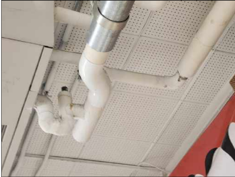
1 - Mold on hydronic plumbing insulation in the cafeteria
