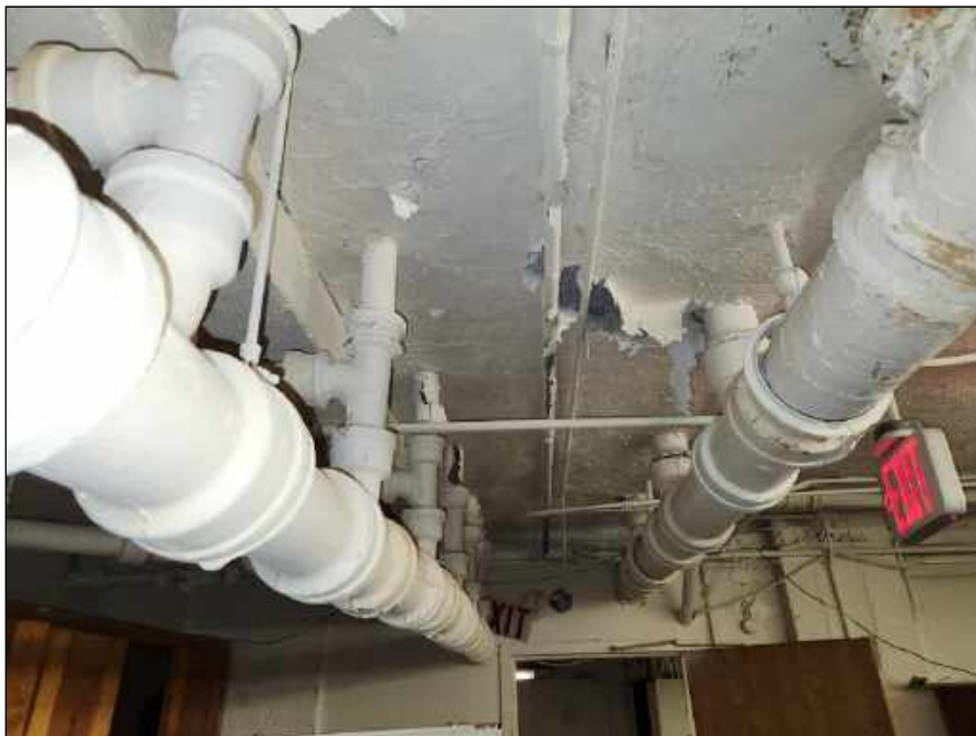
16 - Moisture damaged plaster ceiling in the Harp Room
