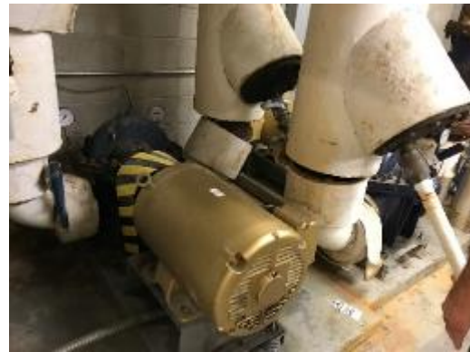
Water-Source Heat Pump Circulation pump
