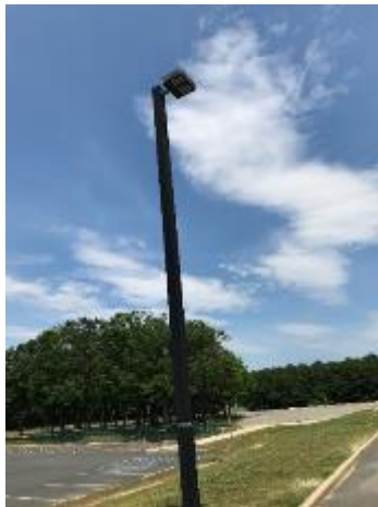
Pole-mounted LED Fixtures
