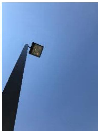
Pole-mounted LED Fixture
