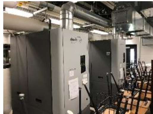
Condensing Boilers – New Addition
