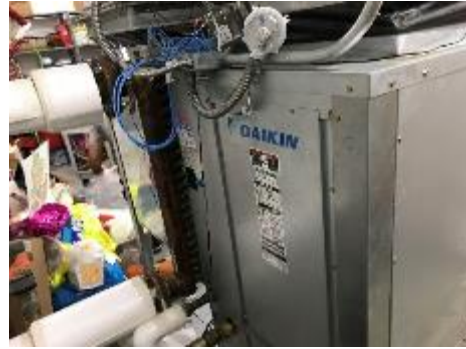
Water Source Heat Pump Unit
