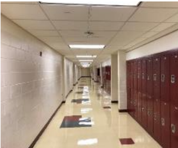
Hallway 4-foot T8 Troffers
