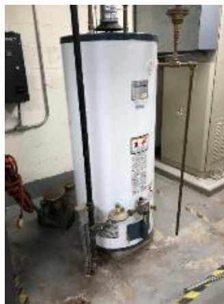
Hot Water Heater
