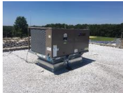
Cafeteria Packaged Units
