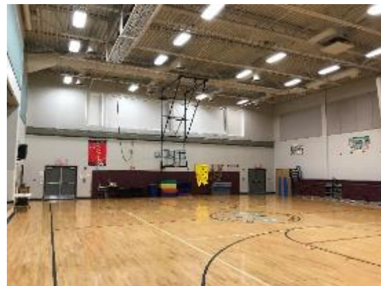
Multi-purpose Room High-ceiling Fixture
