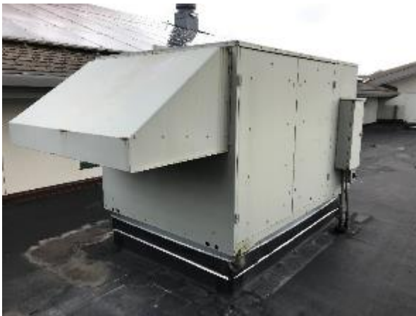
Energy Recovery Units
