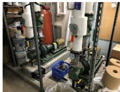
Heating Hot Water Pumps
