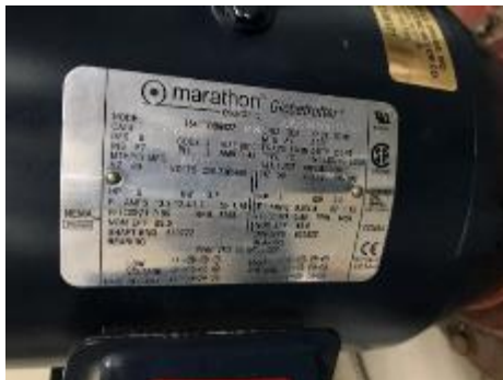
Heating Hot Water Pump
