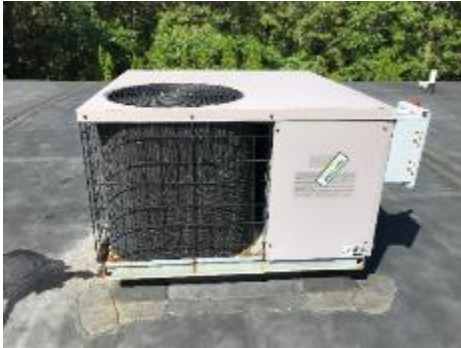
Packaged AC and Heater
