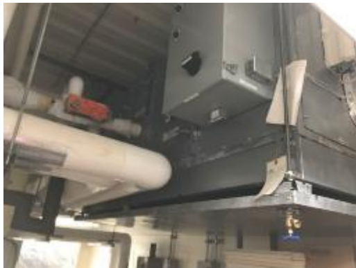
Air Handling Unit
