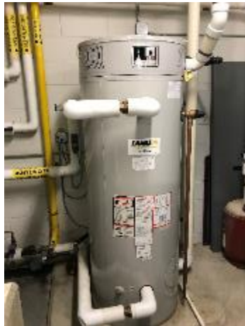
Laars Gas-fired Unit
