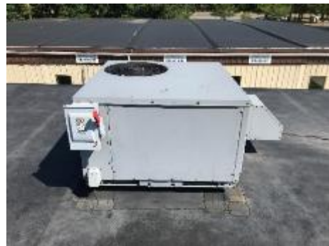
Packaged AC and Heater
