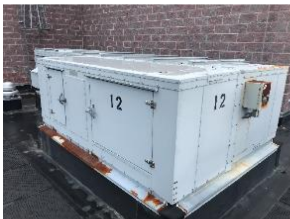
Air Handling Units
