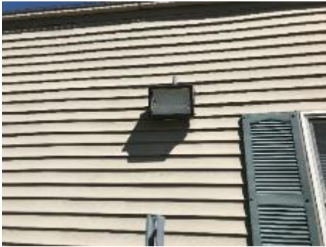
Exterior Light Fixtures
