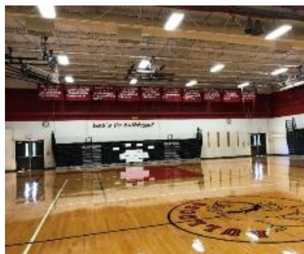
Gym Lighting T5 Fixture
