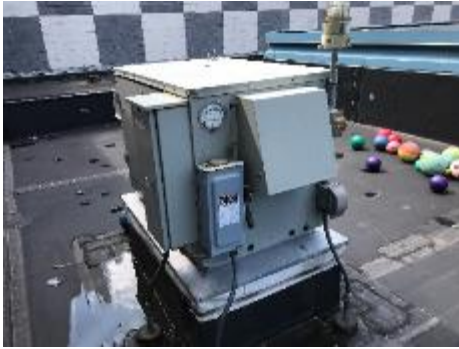
Energy Recovery Units
