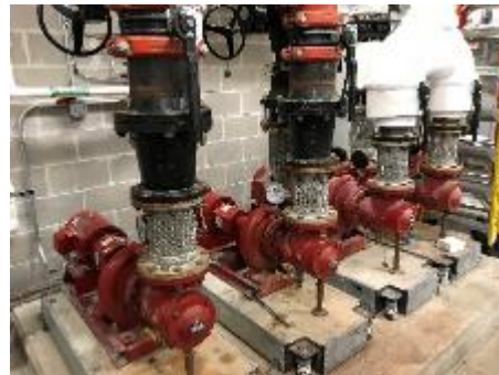
Heating Hot Water Pumps
