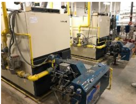
Non-condensing Hot Water Boilers
