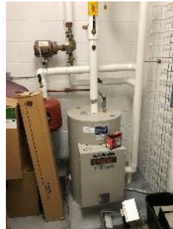
AO Smith electric Unit
