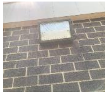
Wall-mounted LED Fixtures
