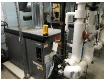
Condensing Hot Water Boiler
