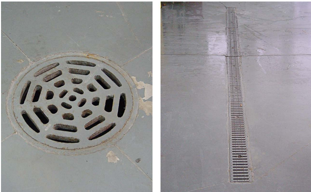
Keeping floor drains clear helps eliminate standing water.
