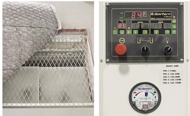
Replacing filters and maintaining proper balance ensure proper operation of a spraybooth.
