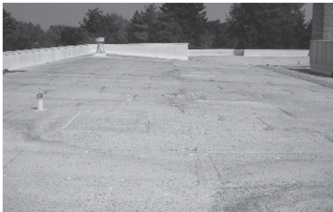
MAIN ROOF AREA WITH SOME EROSION
