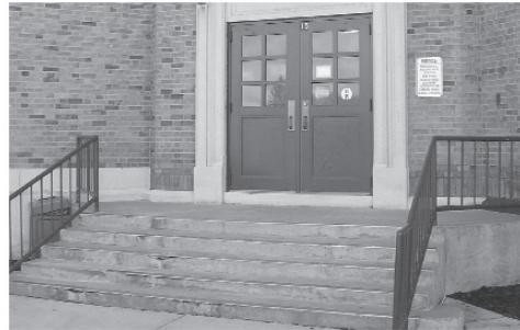
OLD STEEL DOOR, WORN STEPS
