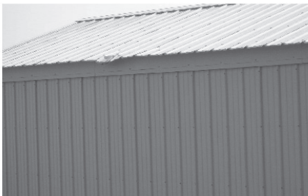
DAMAGED ROOF EDGE
