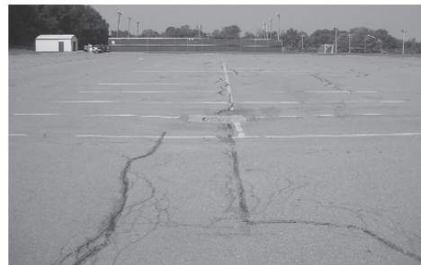
PAVEMENT CRACKING IN LINE WITH DRAIN STRUCTURE
