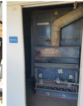
AGING HEATING/COOLING SYSTEM
