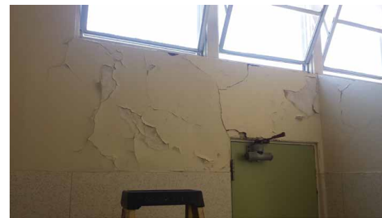
LEAKING WINDOWS CAUSE WATER DAMAGED WALLS
