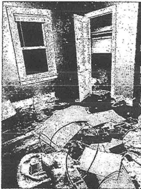
88 Woodstock, 2/19/2020, Pytko move-out condition
