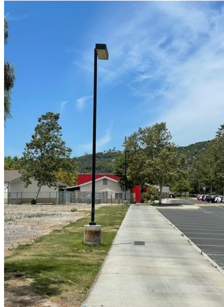
East Parking lot light post
