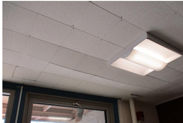
3.6 Sagging acoustical ceiling tiles
