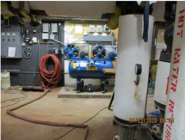
4.2 Air compressor tank for pneumatic control
