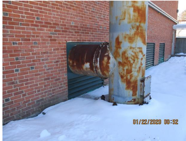
2.2 Rusted boiler flue
