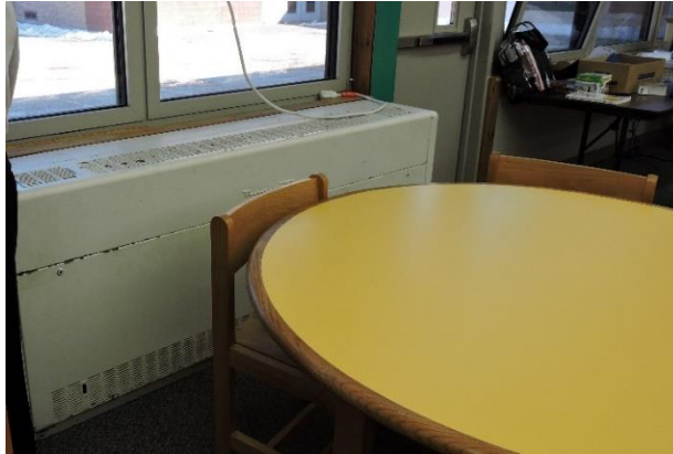
4.6 Unit ventilator in 1950 building
