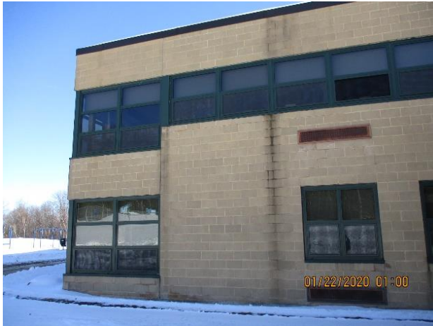
2.1 Staining and efflorescence on masonry wall
