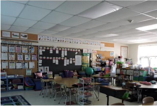
3.11 2x4 ACT tiles in the 1989 addition are warped and sagging
