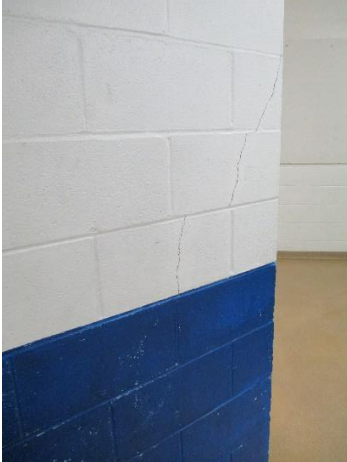
3.35 Stress cracks on masonry wall.
