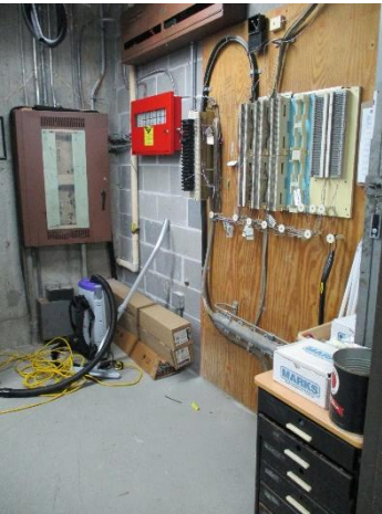
5.1 Telephone network panel.
