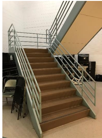
3.28 Non-compliant handrails / guardrails.
