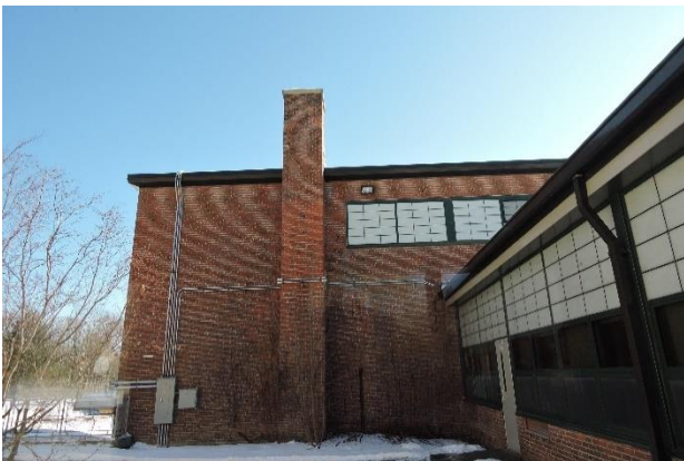
3.8 Roof leak through chimney
