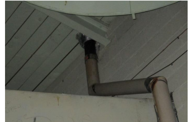
3.7 Leaking interior roof drain leader
