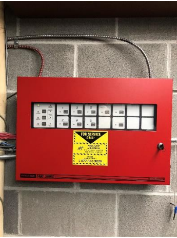
5.4 Fire alarm panel.
