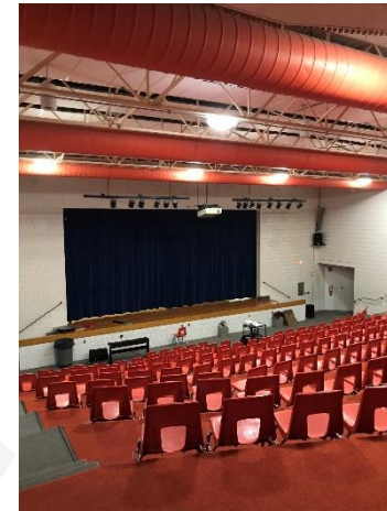
3.29 Auditorium stage lighting.
