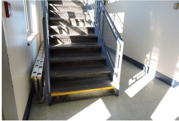
3.12 Non-compliant Handrails/Guardrails on Stairs in 1989 Addition
