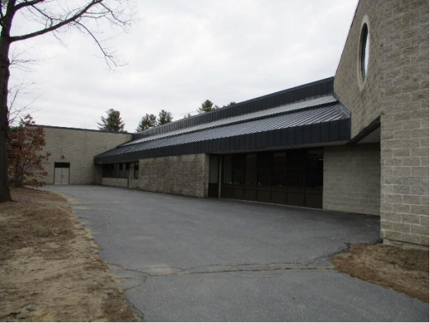
2.4 Staining on masonry wall.
