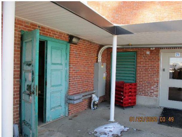
5.4 Main electrical room
