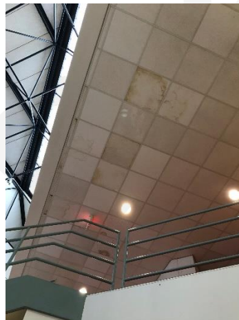
3.12 Stained ceiling tile.
