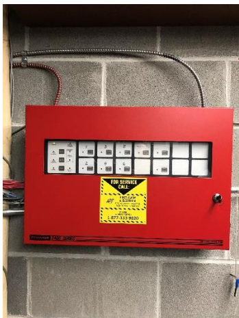
5.4 Fire alarm panel.
