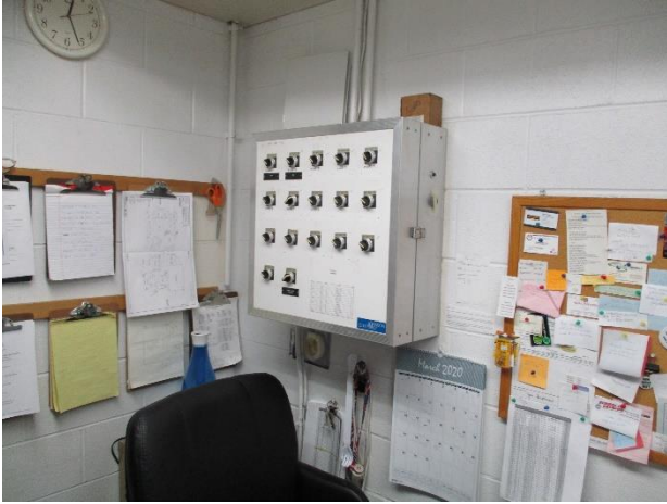
4.1 Pneumatic control panel
