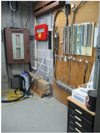
5.1 Telephone network panel.
