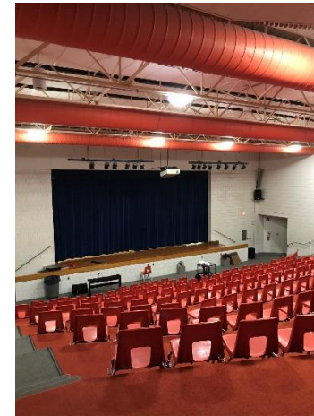
3.29 Auditorium stage lighting.
