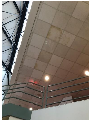
3.12 Stained ceiling tile.
