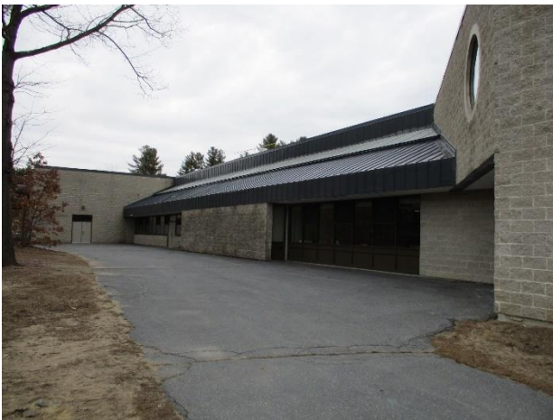
2.4 Staining on masonry wall.
