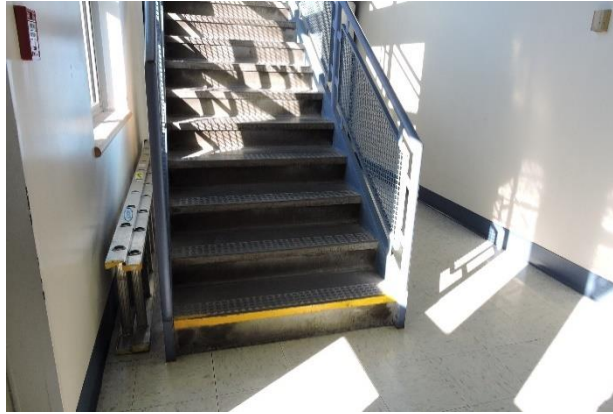
3.12 Non-compliant Handrails/Guardrails on Stairs in 1989 Addition
