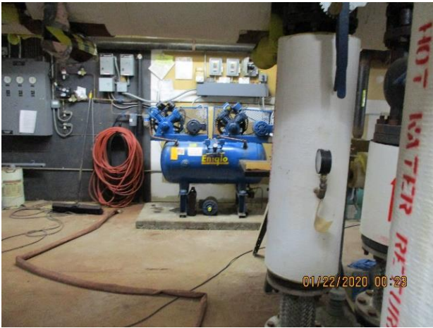
4.2 Air compressor tank for pneumatic control
