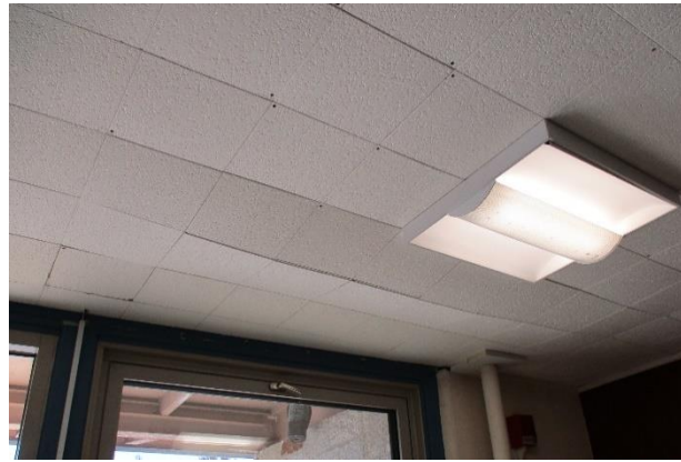
3.6 Sagging acoustical ceiling tiles
