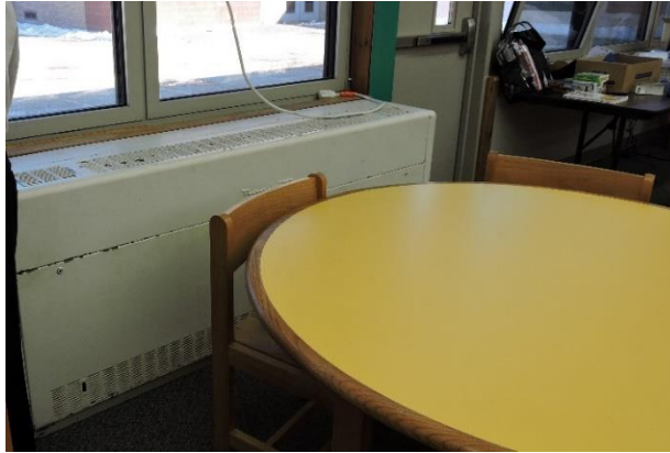
4.6 Unit ventilator in 1950 building
