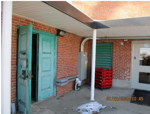
5.4 Main electrical room
