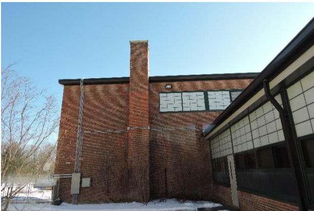
3.8 Roof leak through chimney
