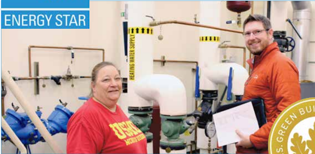
Resource Conservation Manager Jeff Hamman and Head Custodian Shelley Grimsrud inspect the boiler system at Imlay Elementary School.
