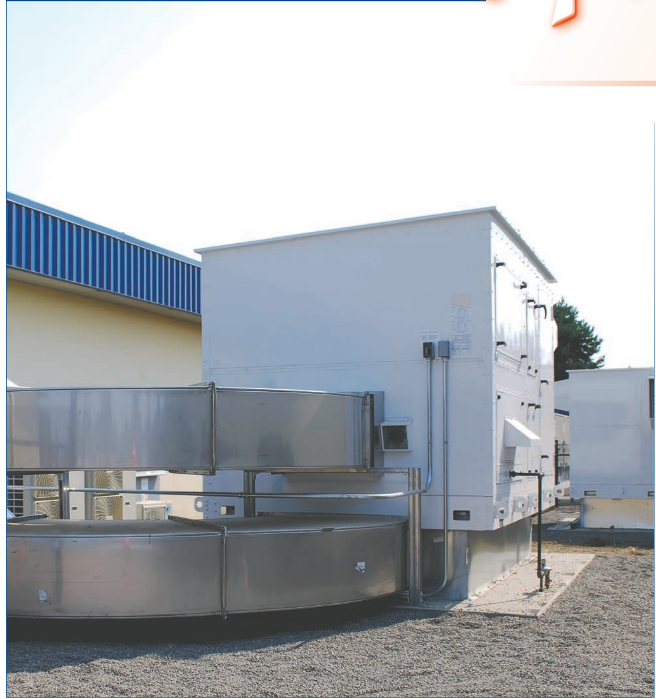
▲Ladd Acres ES: higher-efficiency HVAC units were installed as part of building renovations in summer 2021.
