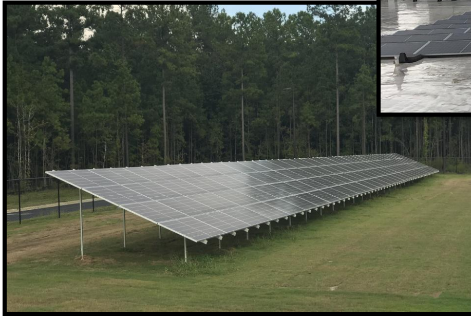
New Hampstead K8 Solar Field
