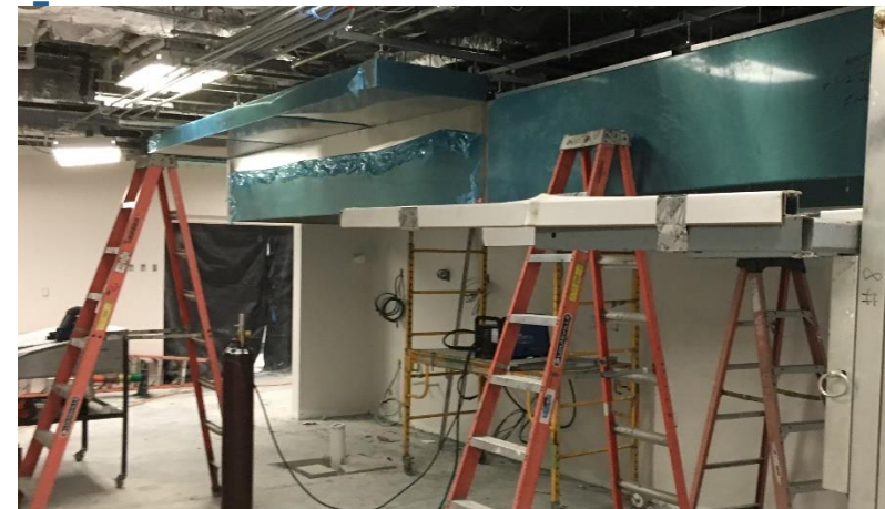
New Exhaust Hood
