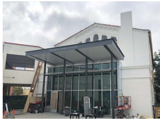
Fremont High School - Modernization project providing New Administration Offices and Main Entrance
